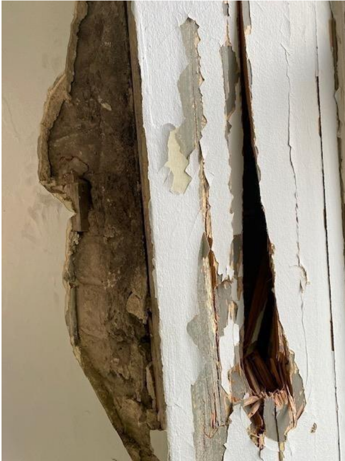
Damaged timber window reveals
