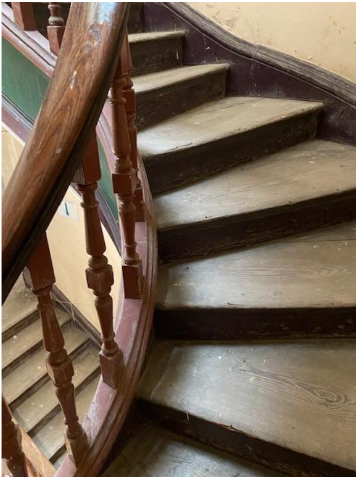
Above: Staircase treads above cracking falling in to central stair sections and as a consequence out of level
