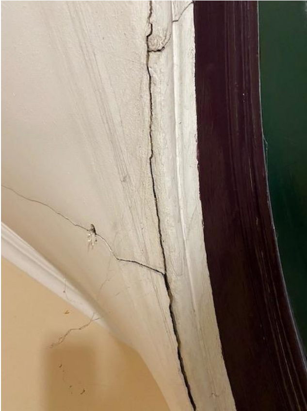
Above: Cracked and deboned geometric stair soffit
