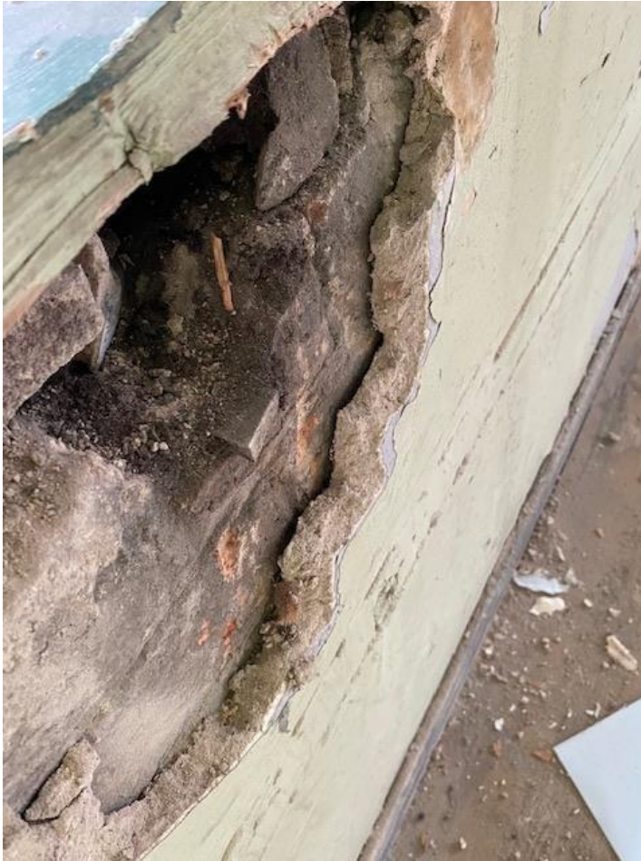
Lime plaster losing its adhesive bond to the brick substrate
