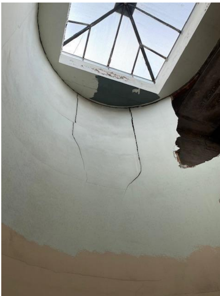
Mindel cracking modern to upper plaster work around staircase
