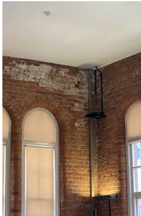
Water ingress to first floor
