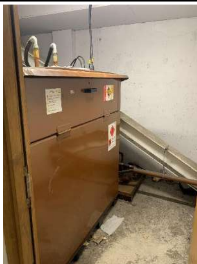
Figure 5 – Looking north, showing the 4300l deisel tank in a small room in the north east corner of the basement.
