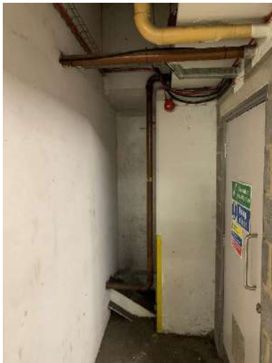
Figure 9 – Looking north, showing the pipe which transfers the deisel throughout the building.
