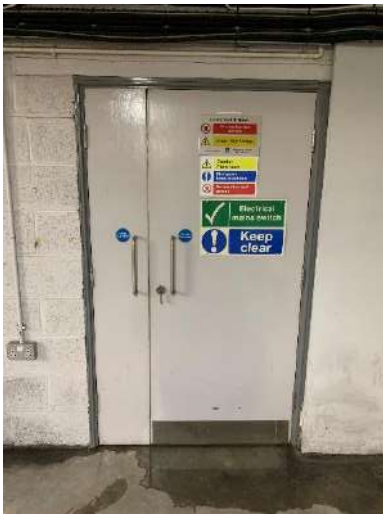
Figure 7 – Looking east, showing a water leak in the mains electrical switch room.
