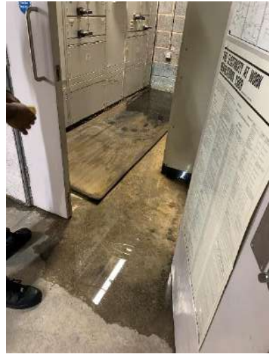
Figure 8 – Looking north east, showing the water leak inside the mains electrical switch room.
