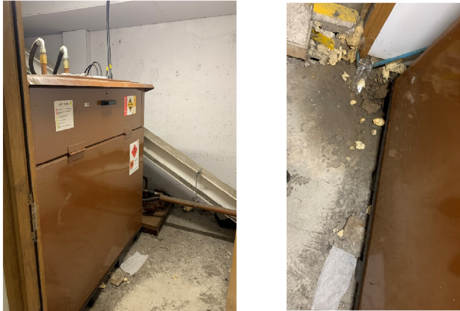
Figure 4: Photographs showing the 4300l diesel tank (left) and no evidence of spillages or leaks on the floor surrounding it (right).
