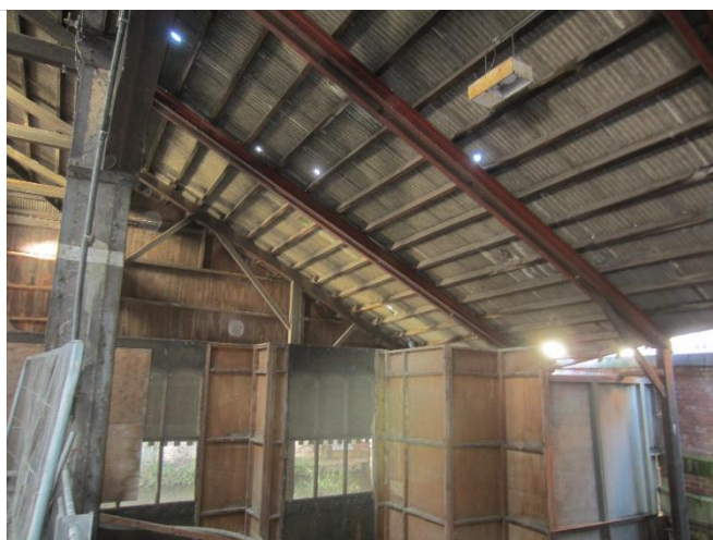
Photo 16: Steel and timber frame supporting corrugated sheet covered roof
