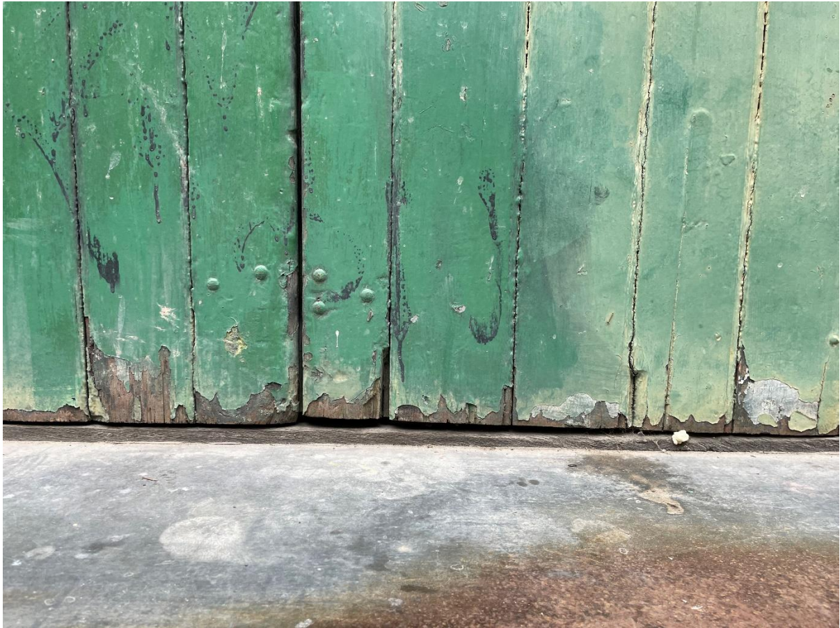
Photograph 5 – Gaps surrounding the loading bay.
