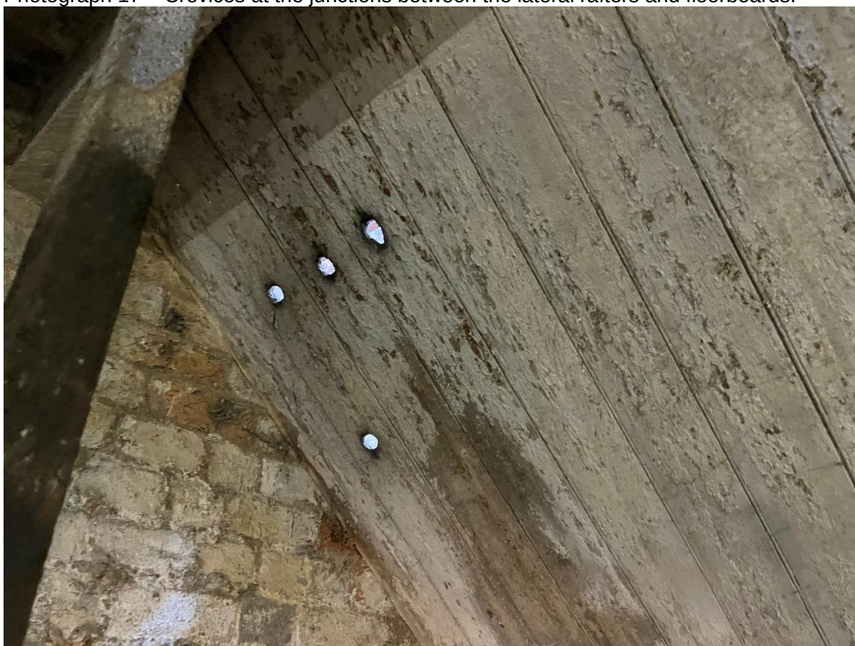
Photograph 18 – Knotholes within the cladding.
