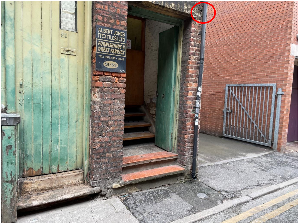
Photograph 3 – Gaps in the brickwork.
