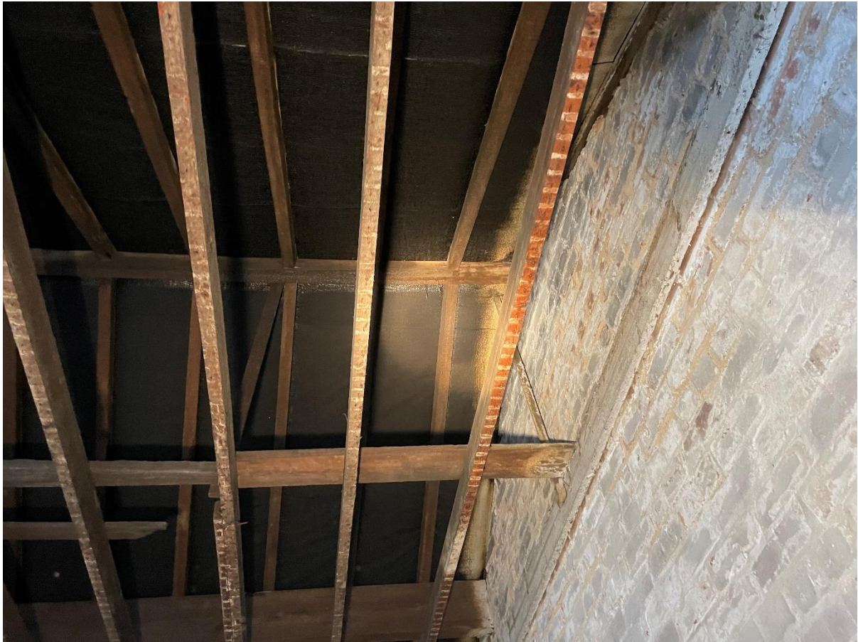
Photograph 13 – Gaps beneath the end rafters.
