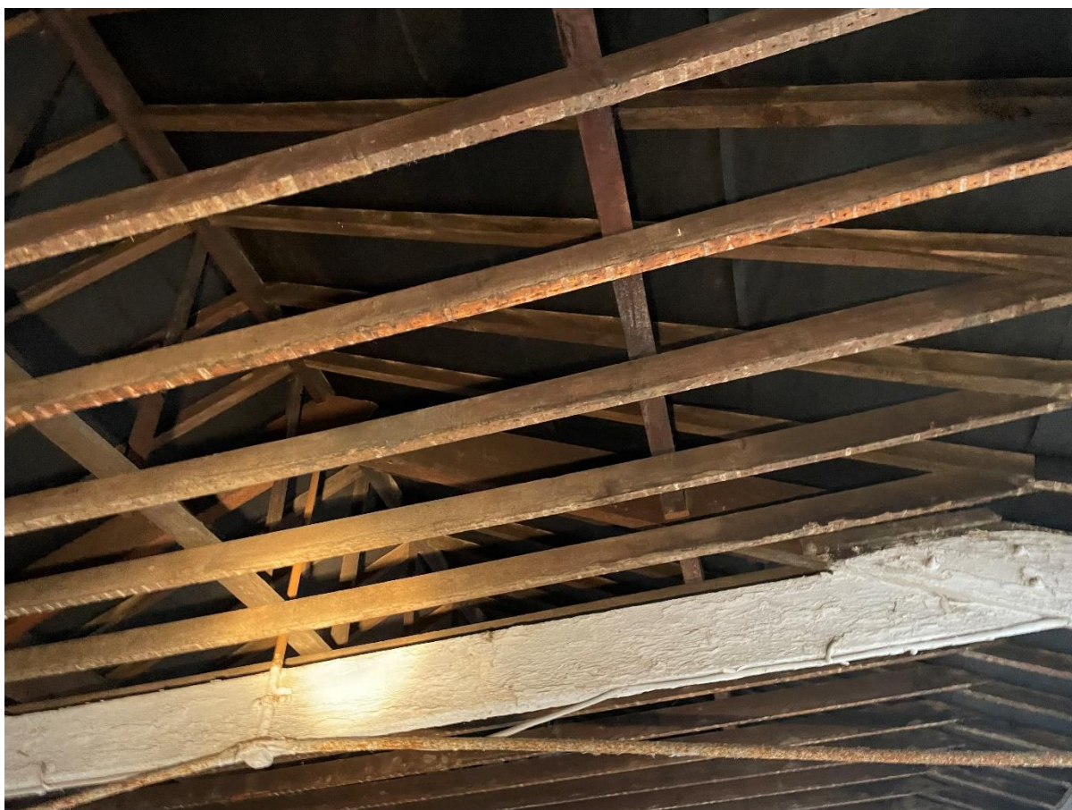
Photograph 9 – Junctions between the ridge beam and rafters.
