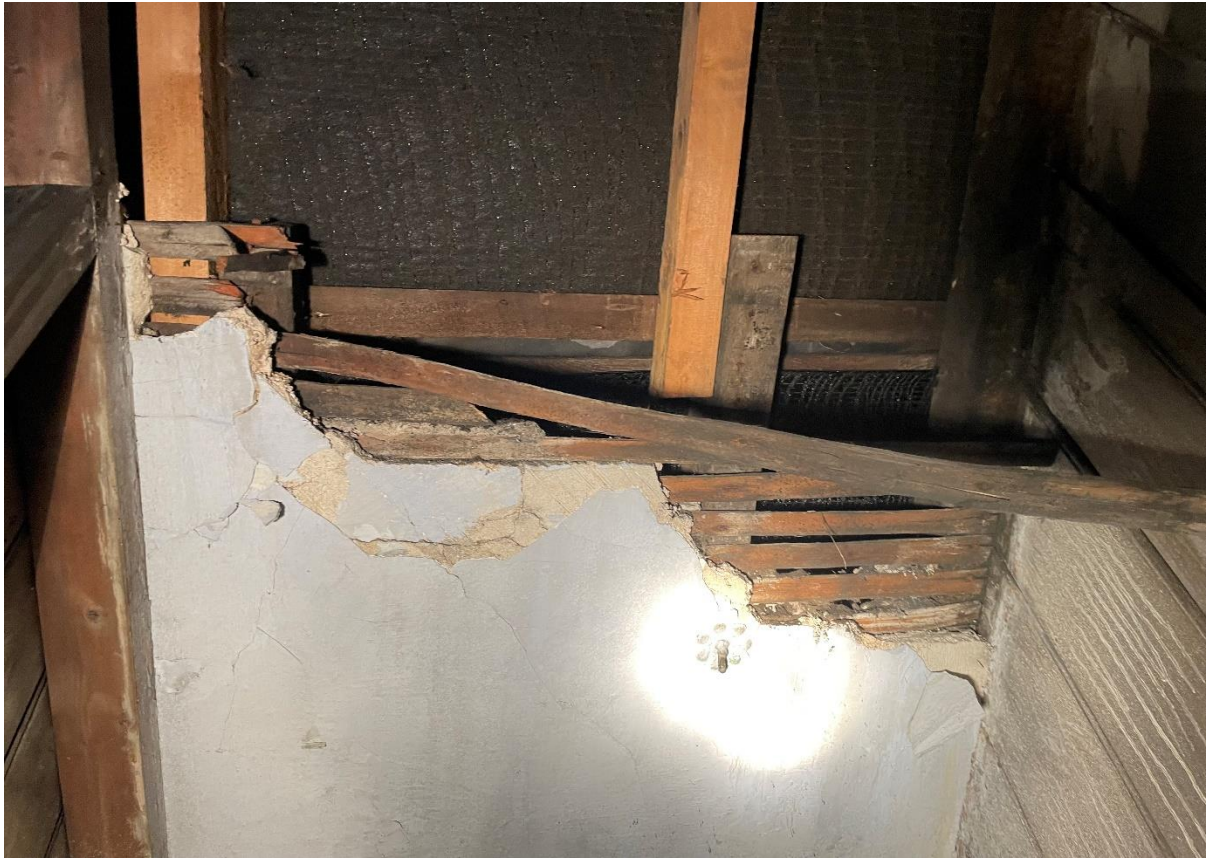
Photograph 11 – Damaged wooden laths and plaster.
