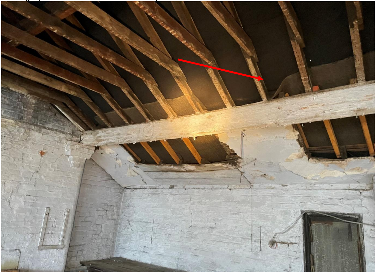
Photograph 8 – Gaps where the bitumen membrane overlaps.
