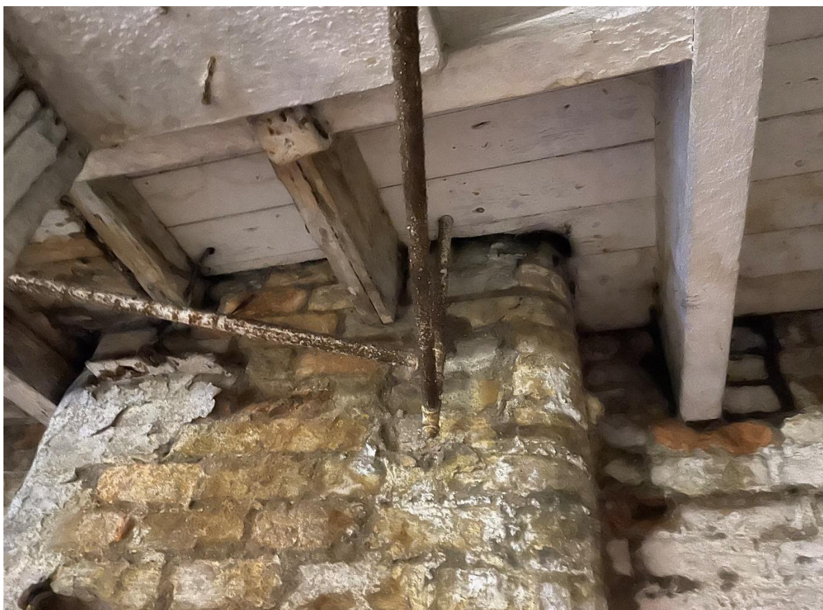
Photograph 19 – Crevices between the floorboards and rendered walls.
