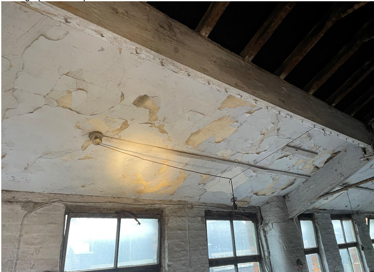
Photograph 14 – Light ingress within the loft void.
