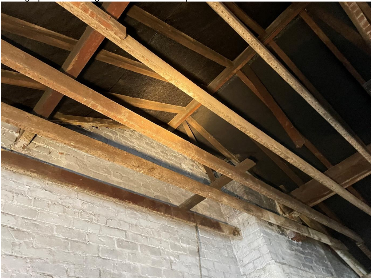
Photograph 12 – Gaps beneath the end rafters.
