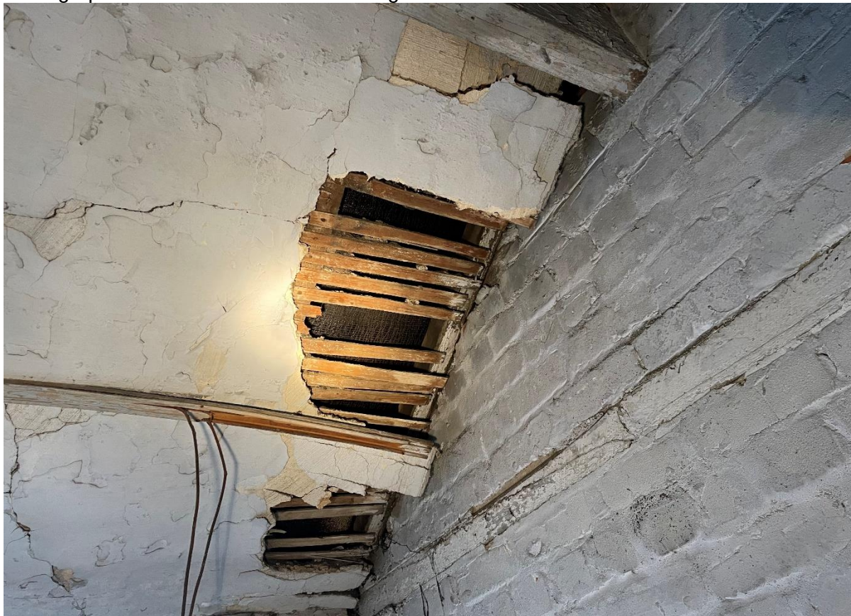
Photograph 10 – Damaged wooden laths and plaster.
