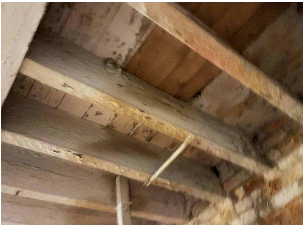
Photograph 17 – Crevices at the junctions between the lateral rafters and floorboards.
