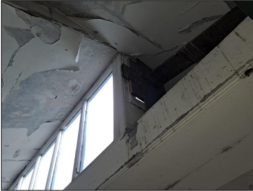
Photograph 7 showing a gap leading to the exterior
