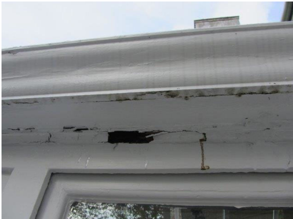
Image 21: Water staining to gutter and wet rot affected timber linings
