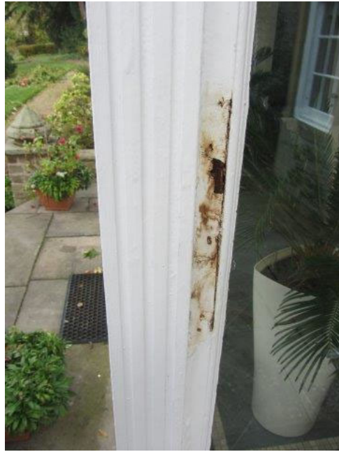
Image 6: Wet rot affected timber
