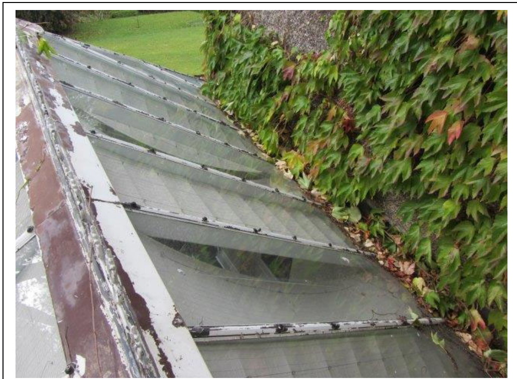
Image 15: Vegetation within trough gutter at abutment to main building
