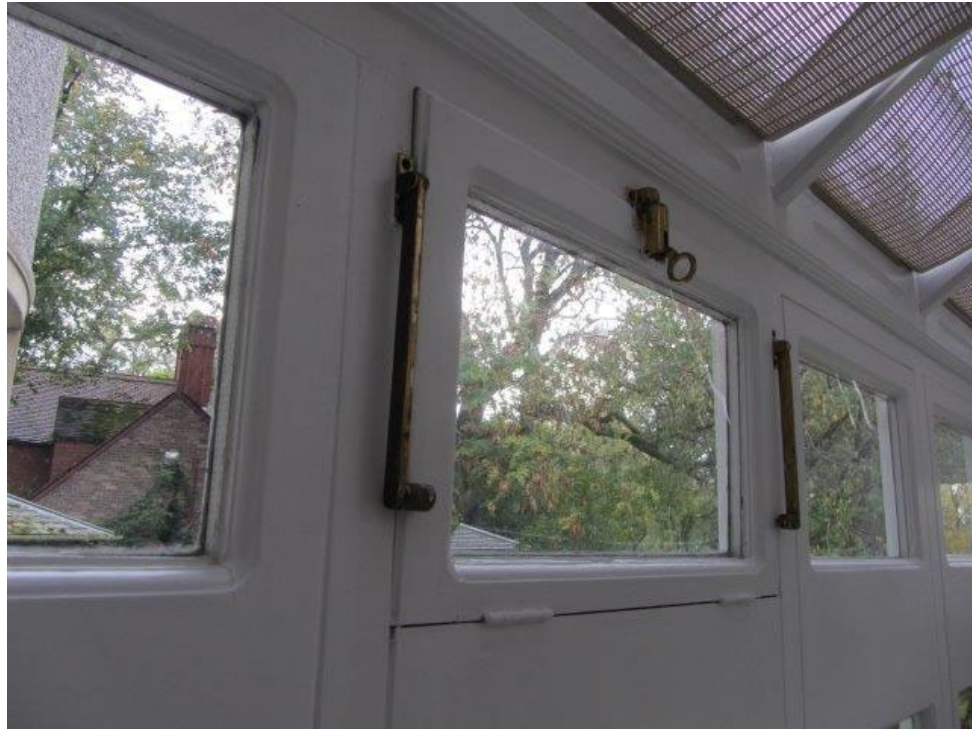
Image 24: Poorly fitting opening casement
