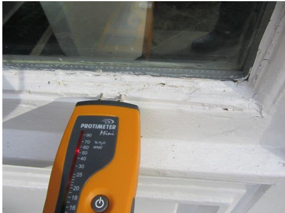
Image 10: High moisture content within glazing beads
