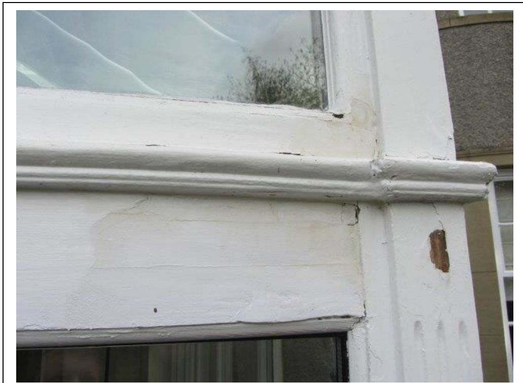
Image 11: Deterioration of decorative finishes
