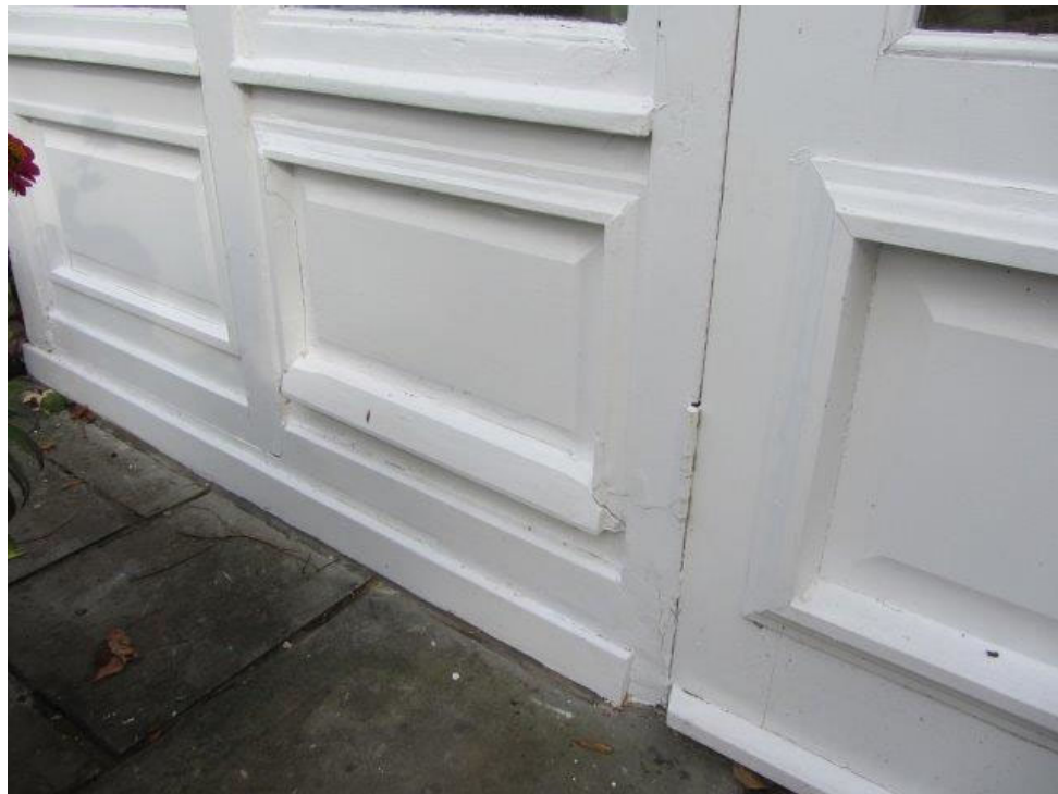
Image 25: Poorly matched timber replacement moulding to infill panel
