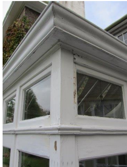
Image 5: Wet rot affected timber
