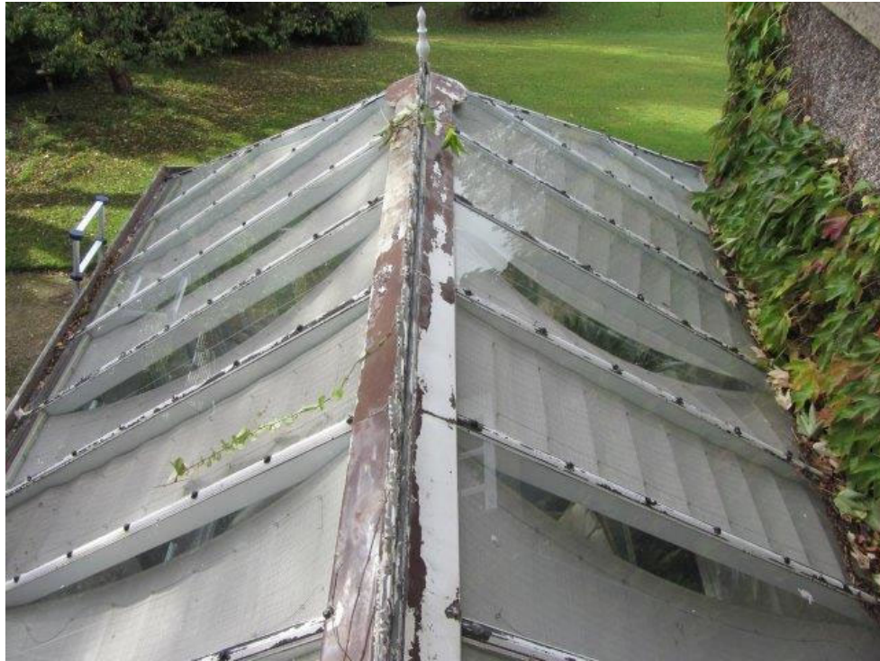
Image 13: Pitched roof in poor condition
