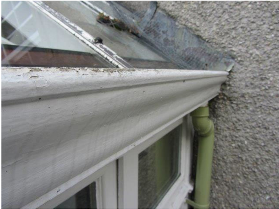
Image 20: Water staining to timber gutter linings
