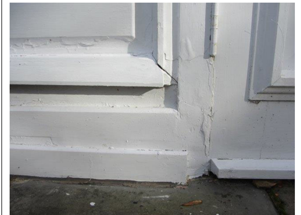
Image 12: General standard of previous timber repairs
