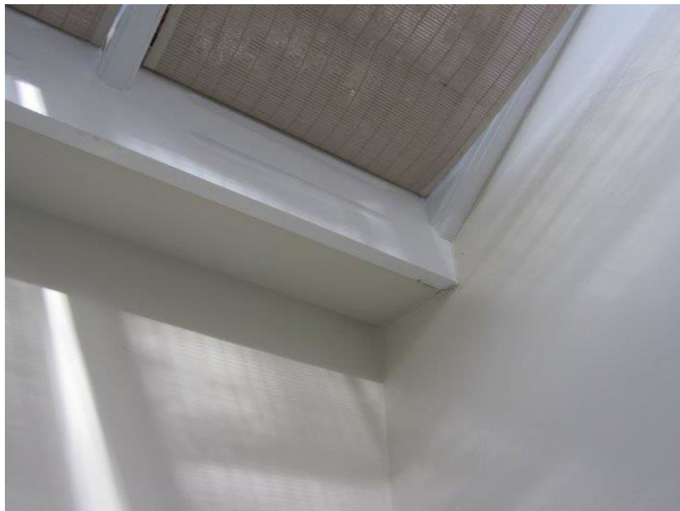
Image 23: Location of reported internal water ingress, under trough gutter
