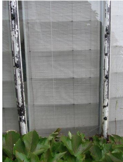
Image 7: Damaged glazed roof panel
