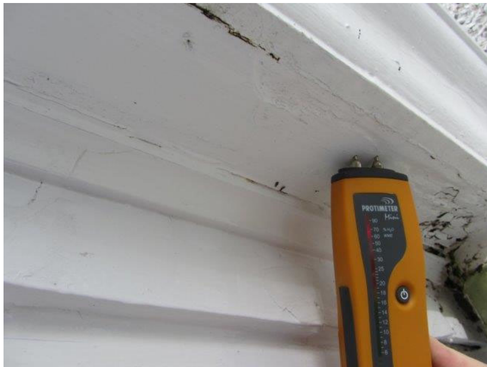
Image 8: Wet rot affected timber soffits to u/s of gutter
