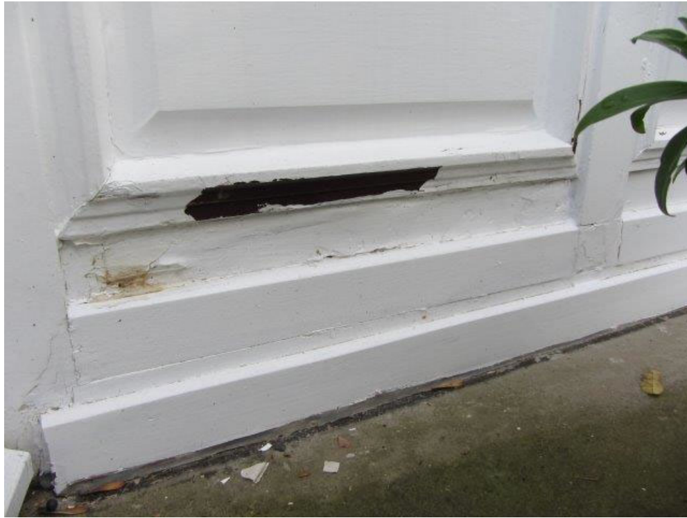
Image 9: Wet rot affected timber, varnished finish exposed
