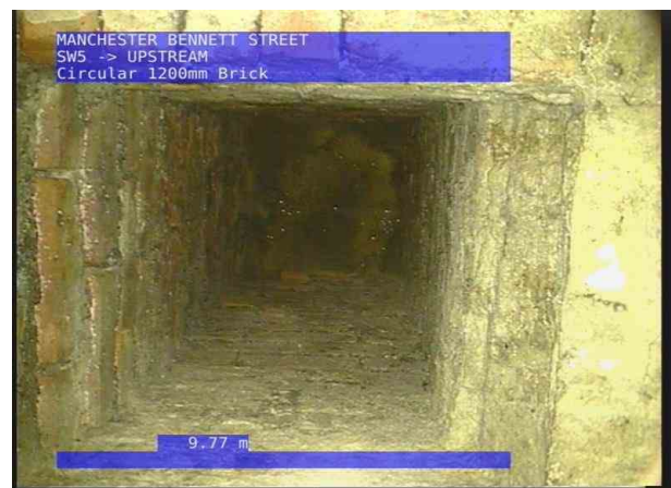
UPSTREAMX_d1bb645d-c35e-4a0e-9bdf-6efff4b8fb1d_20220 715_102205_405.jpg, 00:01:53, 9.77 m General remark, UNCHARTED BURIED MH
