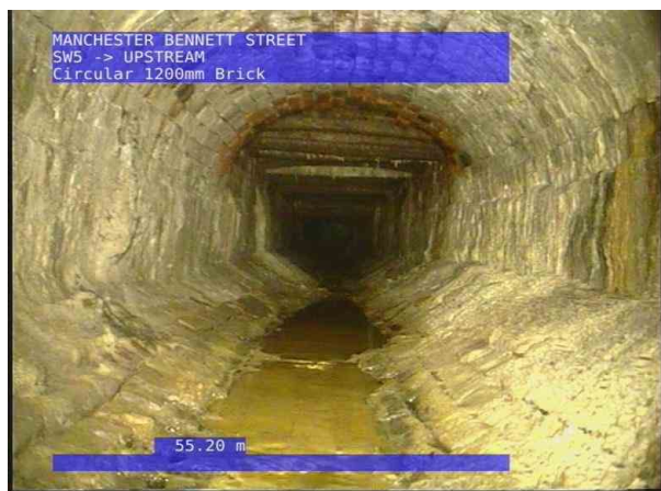
UPSTREAMX_f8c24418-a13f-4c55-a70c-192bd851e9d4_202 20715_103934_959.jpg, 00:17:58, 55.20 m Finish node, other special chamber, reference: UPSTREAM, OFF SITE BOUNDRY
