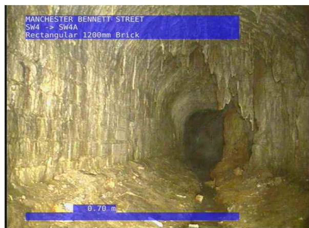
SW4X_19342451-eba2-4aeb-90f1-b38667470ab7_20220714 _100113_847.jpg, 00:00:14, 0.70 m Attached deposits, encrustation from 9 o'clock to 3 o'clock, 5% cross-sectional area loss, start
