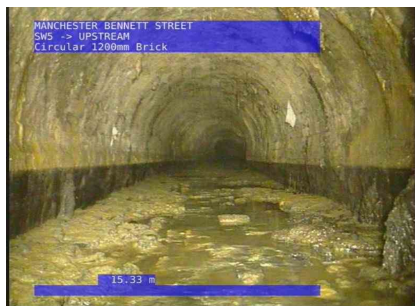
UPSTREAMX_6f20c8d0-bca2-4553-87b5-30119180304b_202 20715_102623_179.jpg, 00:05:48, 15.33 m Attached deposits, encrustation from 12 o'clock to 12 o'clock, 5% cross-sectional area loss, start
