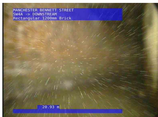
SW4AX_c84c1016-437e-471c-9877-f595c03dc179_20220714_100647_964.jpg, 00:03:21, 20.93 m Line deviates right
