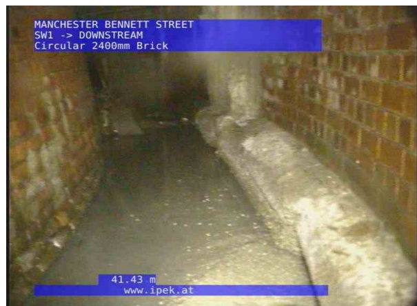
SW1X_1c0b4acb-78a6-4cd2-92f4-c5eb4298fc5d_20220715_114657_886.jpg, 00:16:17, 41.43 m Finish node, other special chamber, reference: DOWNSTREAM, PAST SITE BOUNDARY
