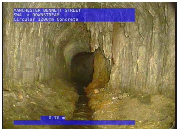
SW4X_c77be944-c213-405d-9b54-fc652ab781be_20220715_105917_832.jpg, 00:00:07, 0.70 m Attached deposits, encrustation from 12 o'clock to 12 o'clock, 10% cross-sectional area loss
