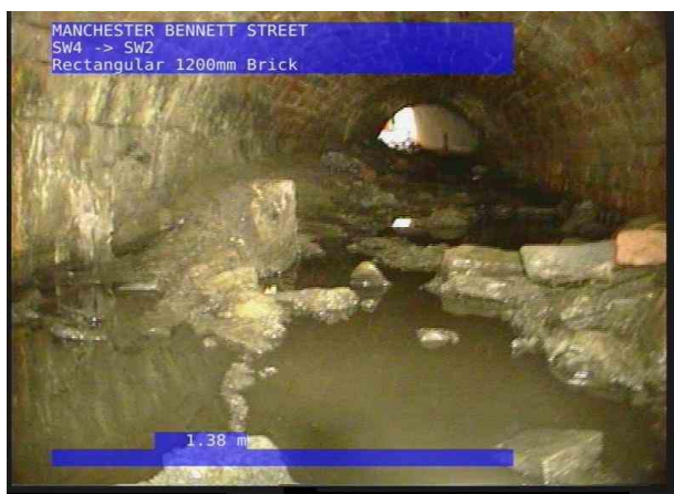
SW2X_b4adb64d-9b77-4045-81e2-e264cd73f99f_20220715_100039_278.jpg, 00:00:10, 0.89 m Settled deposits, fine, 10% cross-sectional area loss
