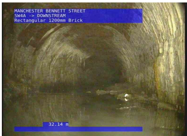
SW4AX_13e2b733-7b1f-4afc-997a-a5fdcf8bd8a1_20220714_100929_571.jpg, 00:05:47, 32.14 m General remark, JOINTS UP WITH THE D/S FROM MH SW1
