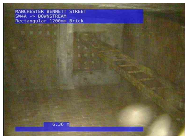
SW4AX_53ac047a-fb86-4483-b433-5af403bff074_20220714_100413_580.jpg, 00:01:11, 6.36 m General remark, BURRIED & UNCHARTED MH
