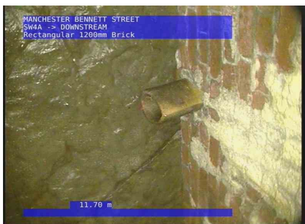
SW4AX_5ae7b2b5-66d7-4b22-b059-5b9f368d99a0_20220714_100536_352.jpg, 00:02:15, 11.69 m Connection defective, connecting pipe is intruding at 1 o'clock, 150mm dia, intrusion: 5%
