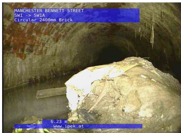
SW1AX_a6df3ce6-3909-4ee5-a819-268de26b1f8f_20220715_115405_753.jpg, 00:01:45, 6.23 m Settled deposits, fine, 20% cross-sectional area loss
