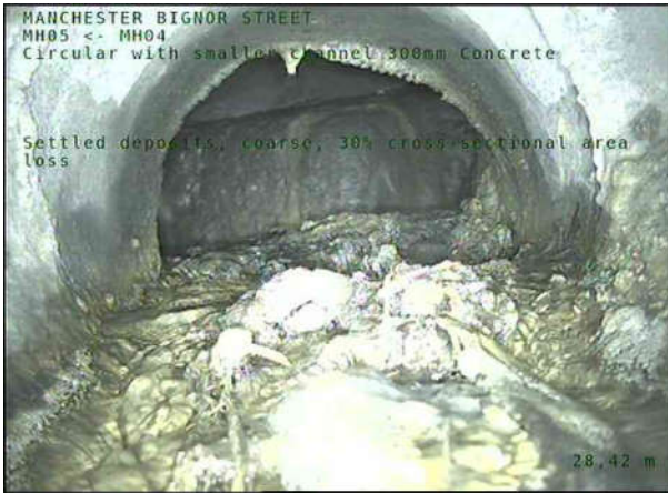
MH05X_2e726287-96e5-4341-aad3-81de6327b705_20201214_103749_426.jpg, 00:02:43, 28.42 m Settled deposits, coarse, 30% cross-sectional area loss
