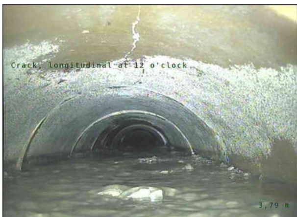
MH08X_90980464-f189-4a2b-930c-d57861c437eb_20201214_113648_280.jpg, 00:00:09, 1.20 m Settled deposits, coarse, 55% cross-sectional area loss, start
