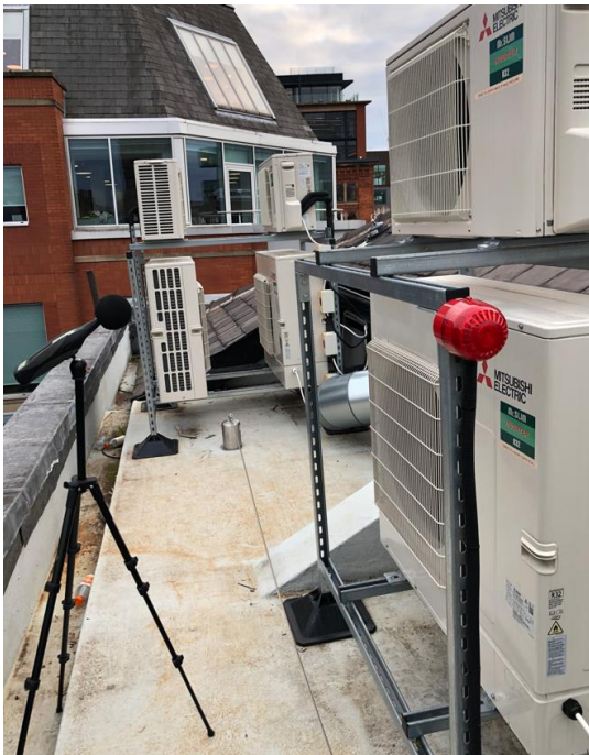
Figure 2 Photograph of the rooftop plant deck including externally mounted plant items
