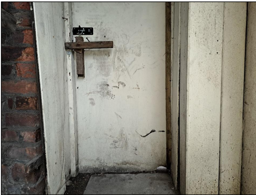
Photograph 8 showing a hole in the door that leads to the external staircase
