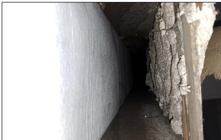
Photograph 13 showing a gap leading to a significant cavity
