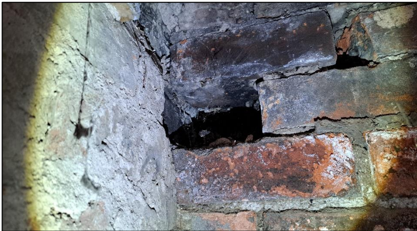
Photograph 12 showing a missing brick
