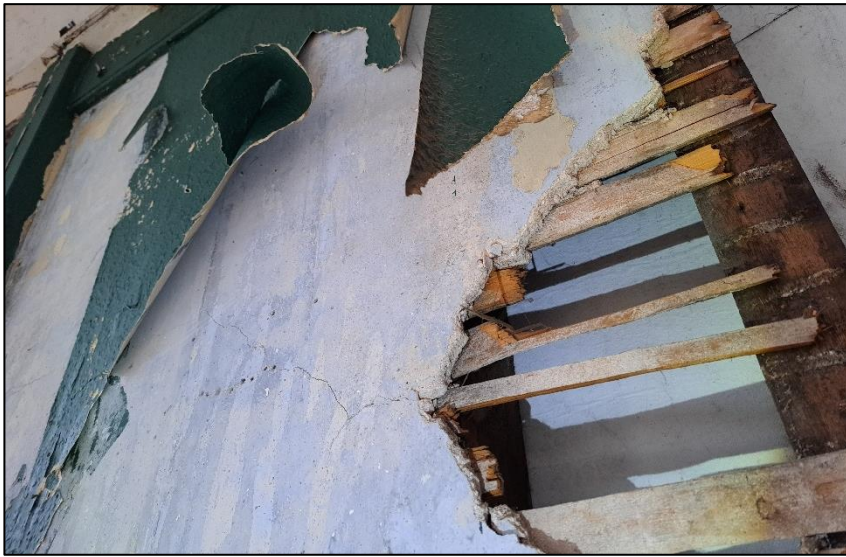
Photograph 11 showing damage to the wall (the cavity wall can be seen)
