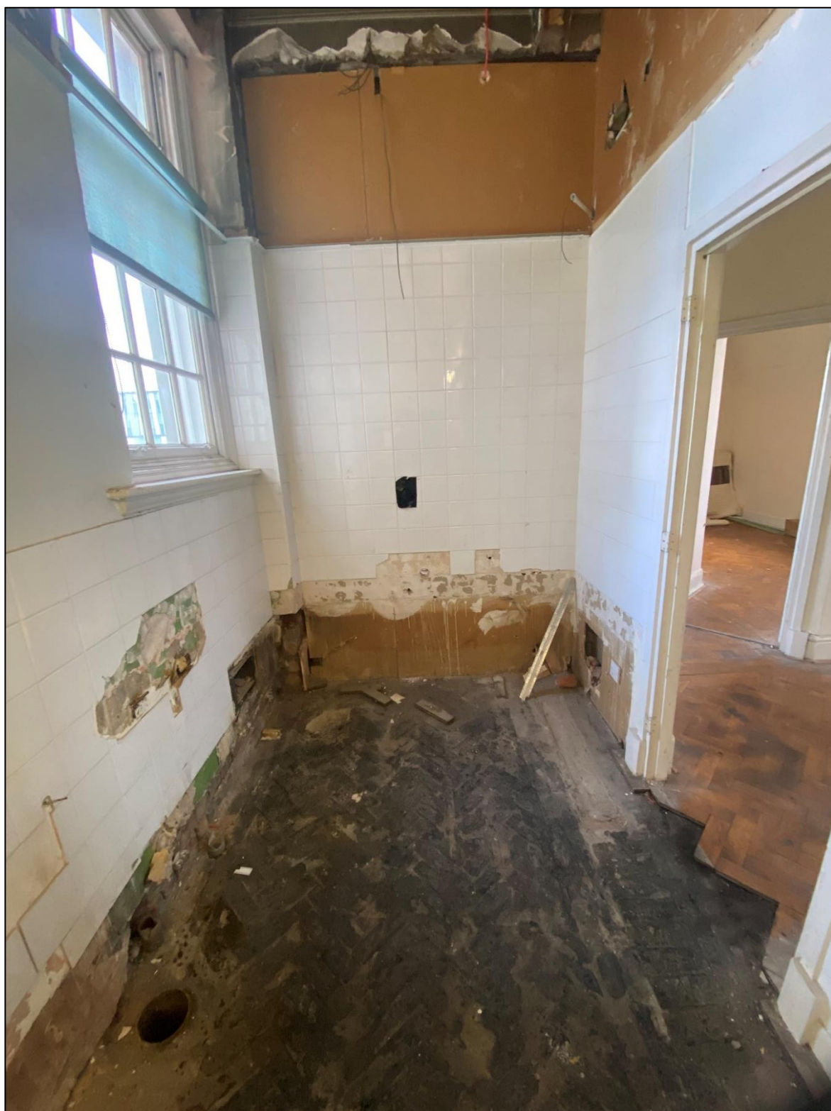
Caretaker's flat with deteriorating material
