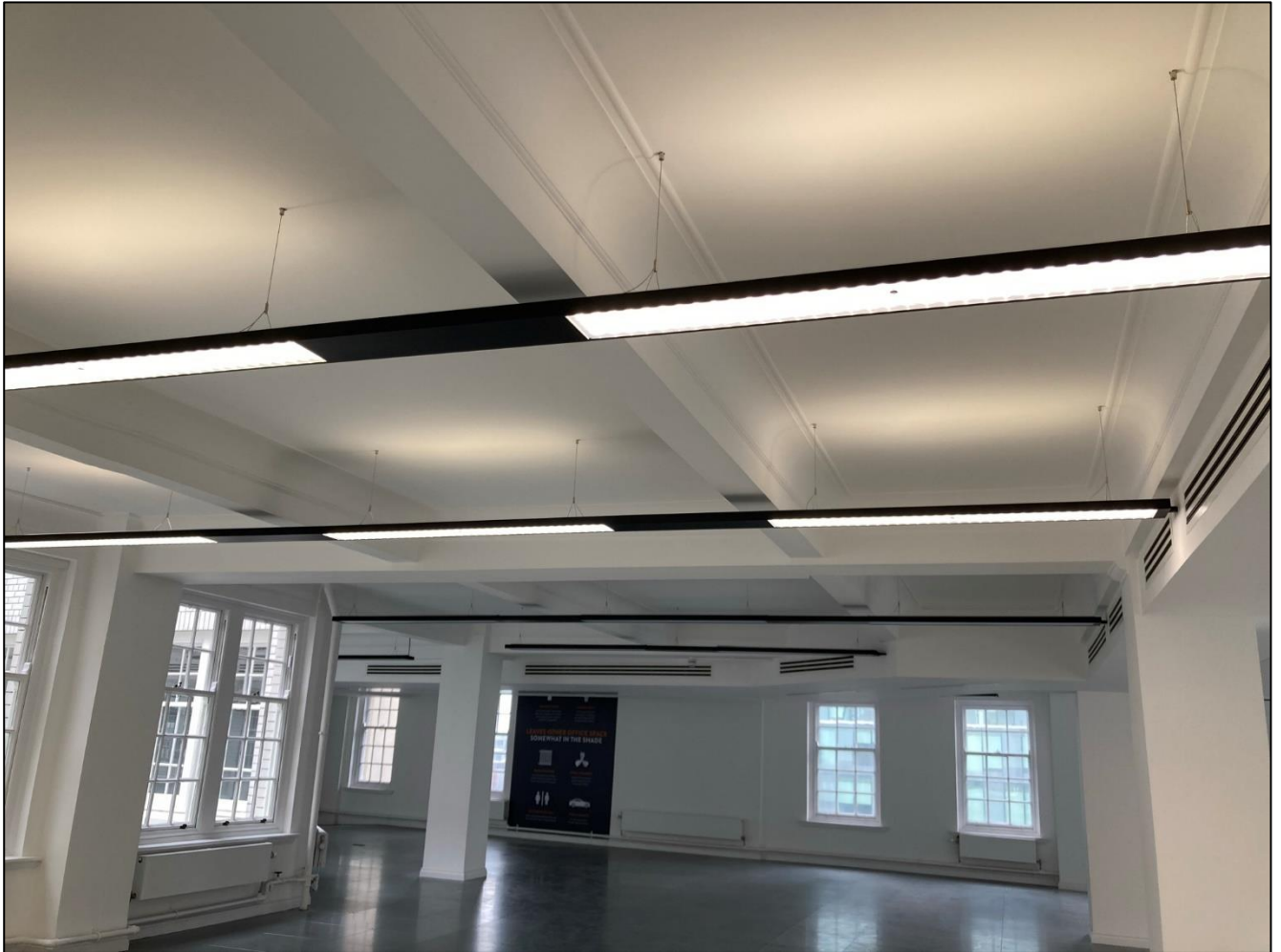
Eighth floor coffered ceiling, with unsympathetic modern lighting
