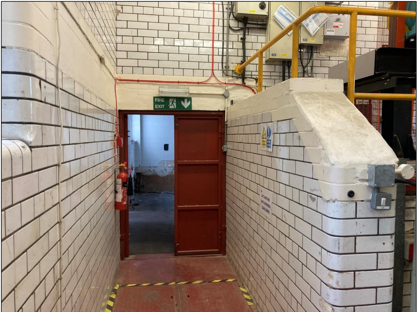
Lift motor room
