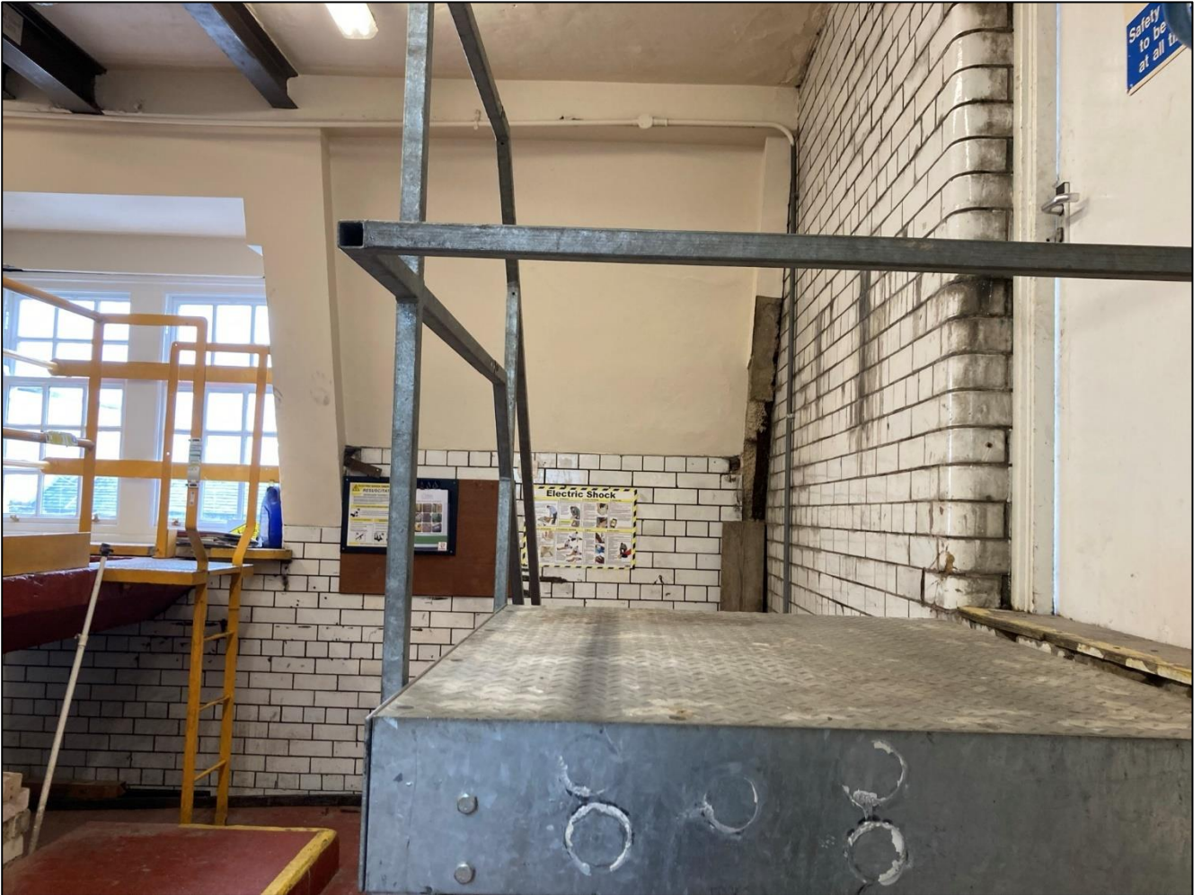
Lift motor room
