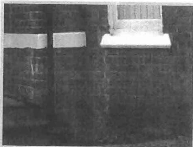
Plate 11. Sign of structural movement
