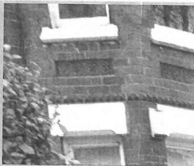
Plate 12. Sign of structural movement
