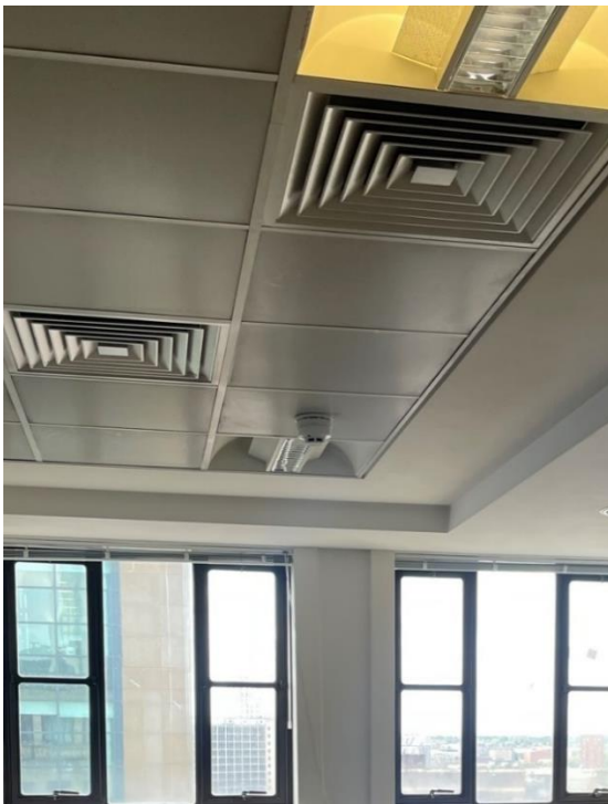
Figure 22: Modern ducted heating / ventilation system evident from grilles within the suspended ceiling
