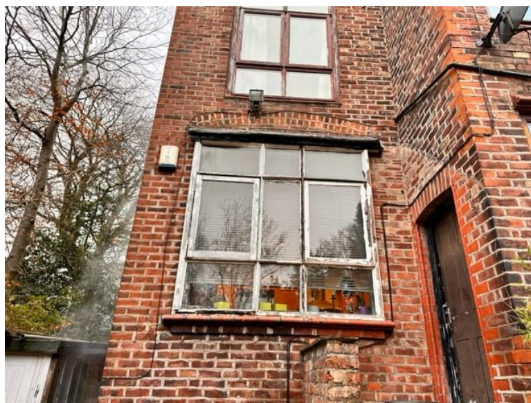
Figure 5.4: Example of deteriorating wooden frame at rear elevation
