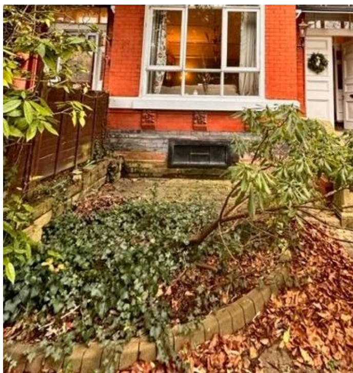
Figure 5.3: Photo of deteriorating opening
