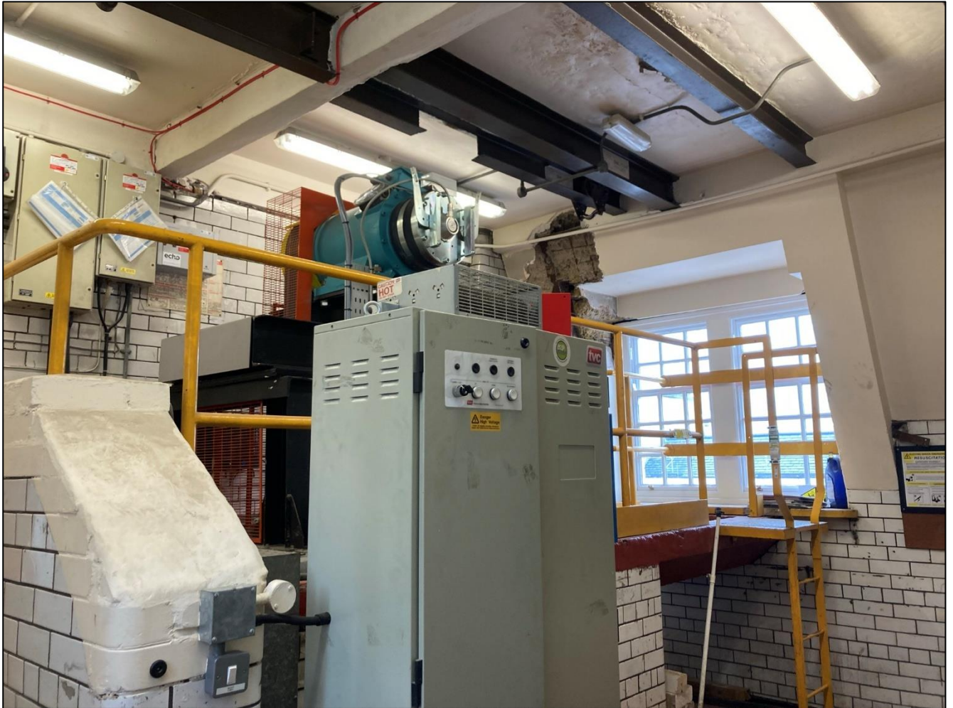
Lift motor room with original tiling
