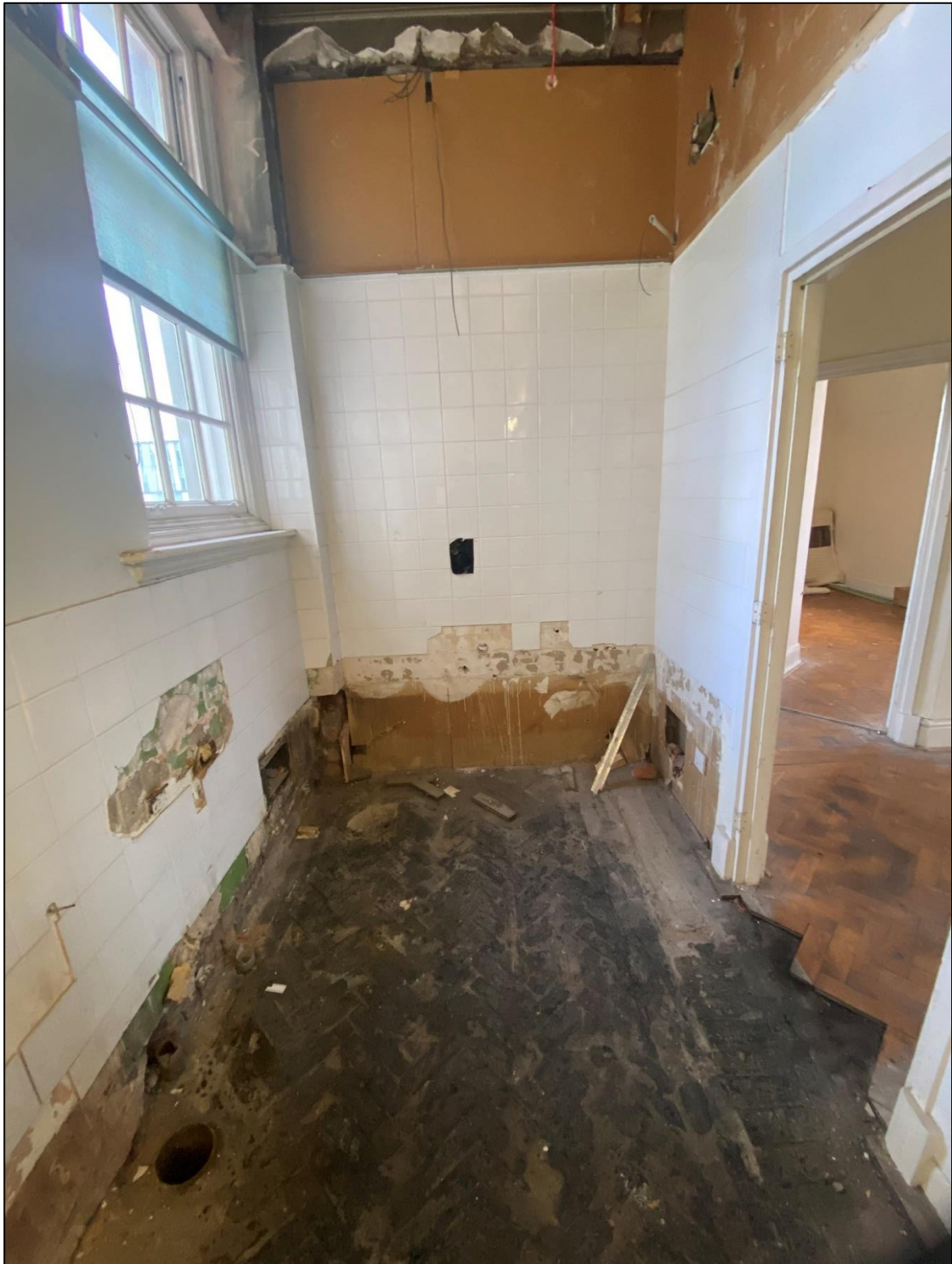
Caretaker's flat with deteriorating material
