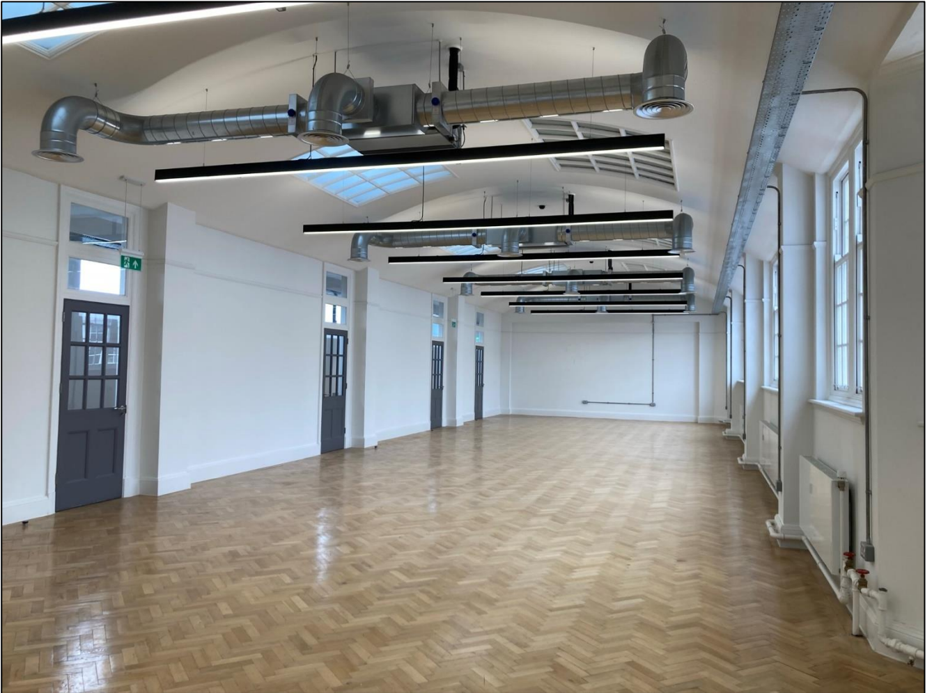
Thirteenth floor with modern fan coil units and lighting
