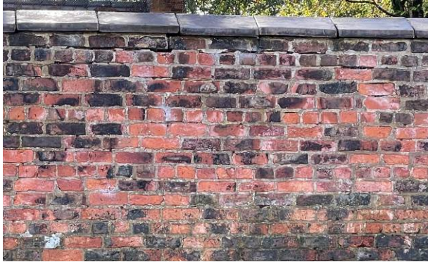
Effects of cement pointing seen on the softer, common brickwork (blown faces).
