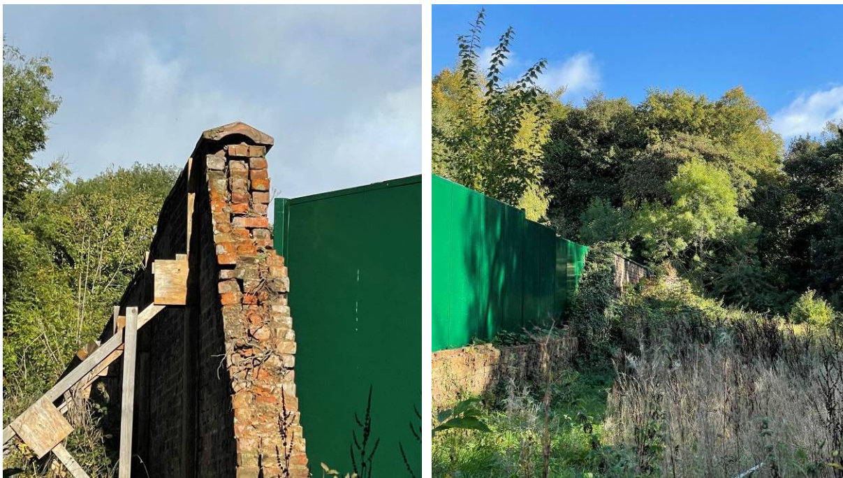
Root growth in the core of the west wall (L), vegetation taking hold on / trees overhanging south wall (R)
