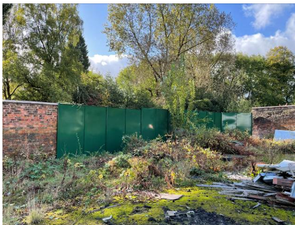
Vegetation build up, collapsed section of south wall.
