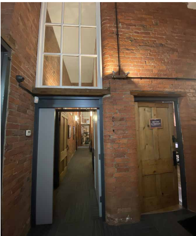
New fire doors to corridor
