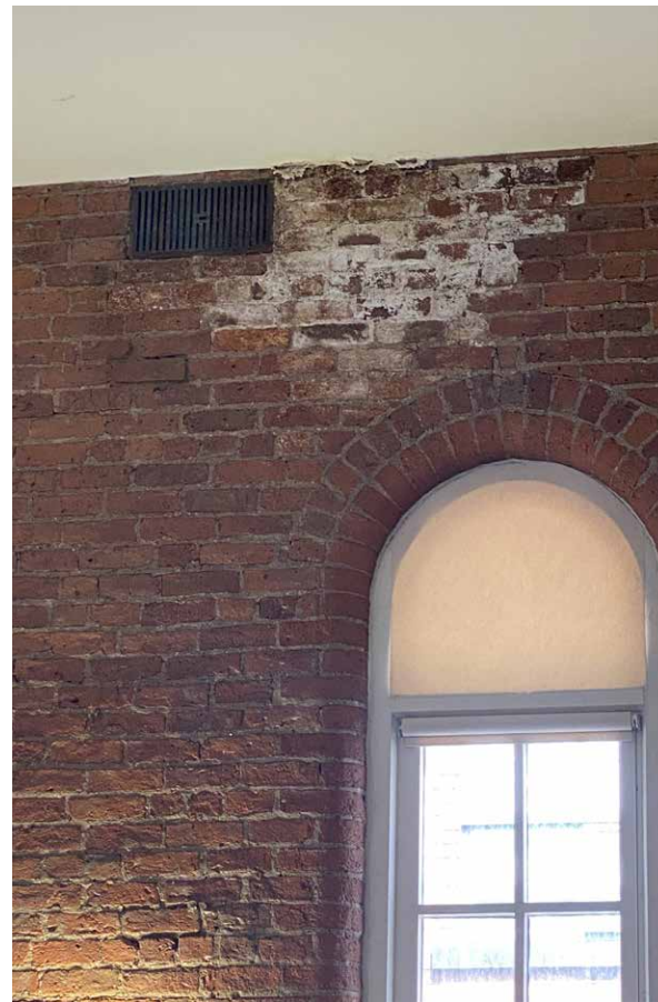
Water ingress to first floor
