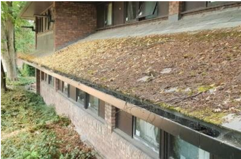
Ewings Building – example of deterioration and maintenance problem
