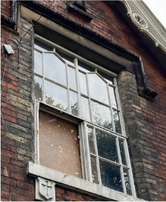
Missing top hung pane to be replaced to match existing
