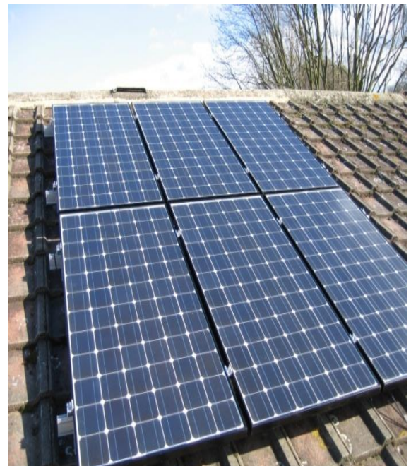
Figure 5 - Photovoltaic array on a pitched roof
