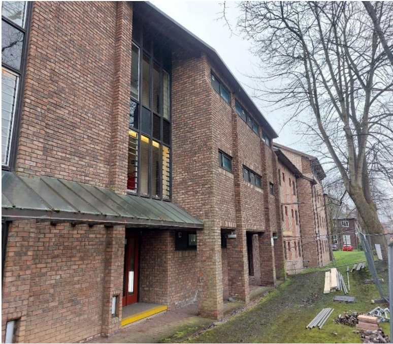
C: Branches obstructing scaffold.
