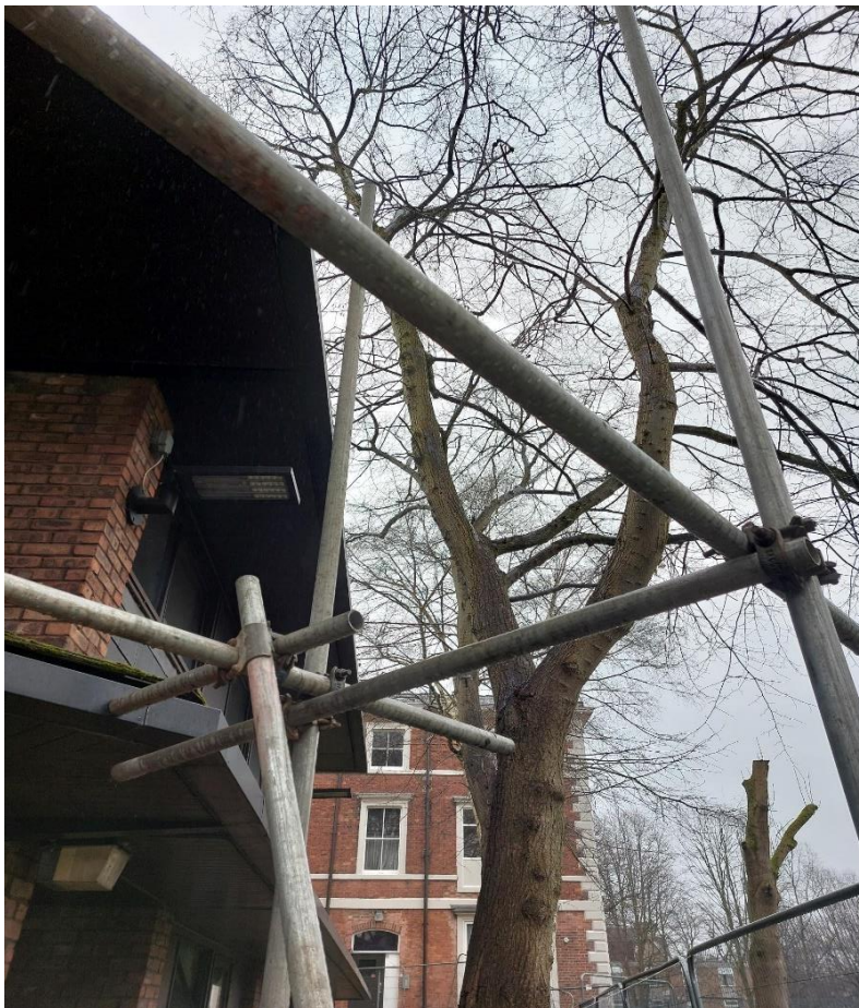
D: Branches obstructing scaffold.
