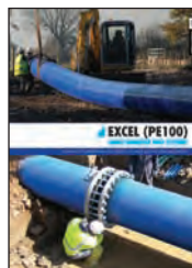
G0020 Large Diameter Pipe Systems
