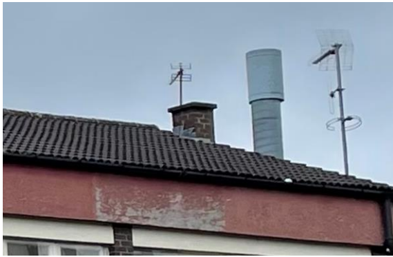
Photograph 6 – Lifted lead flashing around chimney stack
