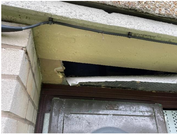
Photograph 17 – Metal sheeting peeling
