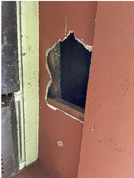
Photograph 18 – Damaged window casing
