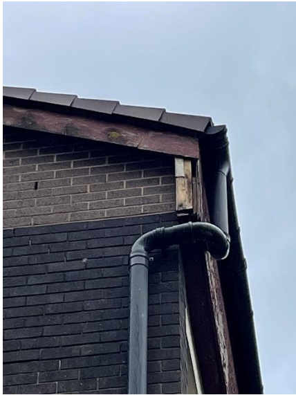
Photograph 11 – Damaged fascia (south-eastern corner)
