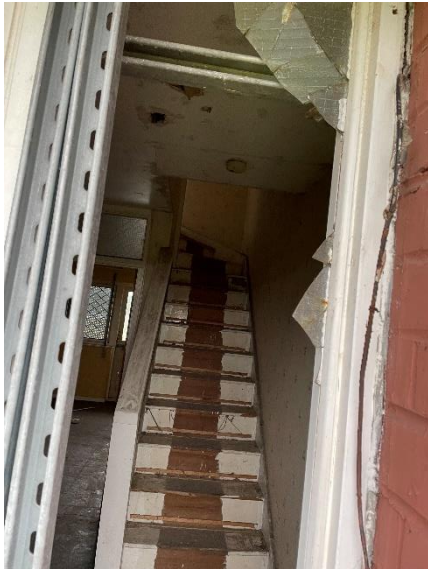
Photograph 15 – Broken window around door
