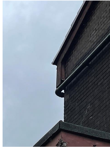
Photograph 12 – Damaged fascia (south-western corner)
