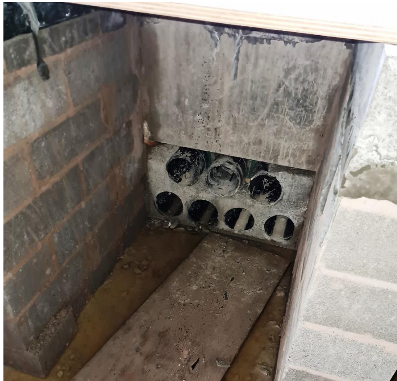
Figure 3.5 Ducts for HV cables into the substation enclosure within the cable trenches under the floor.
