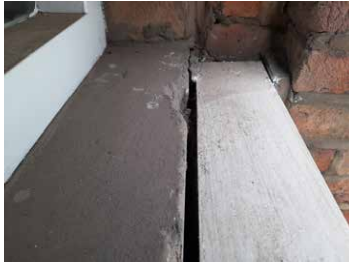
A1001: Loose sill. Check sill stability/replace sill
