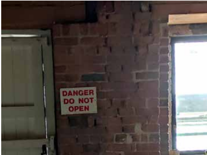
A0036: Defective pointing. Re-point
