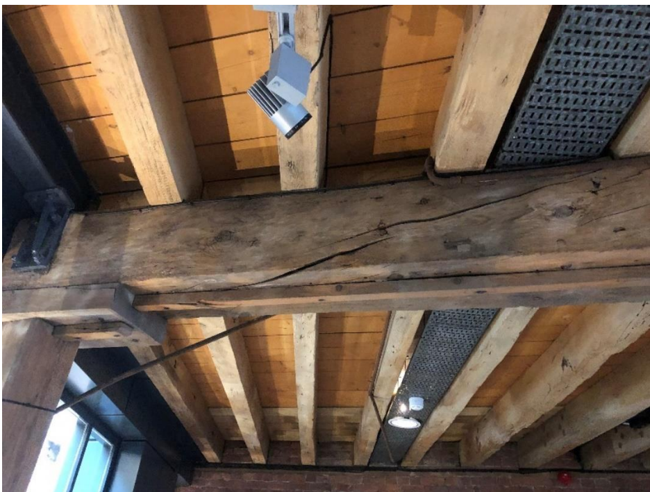
Photograph 16 – View from first floor level of diagonal cracking in floor beam.
