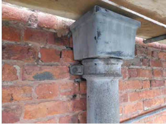
A1042: Defective pointing. Repoint
