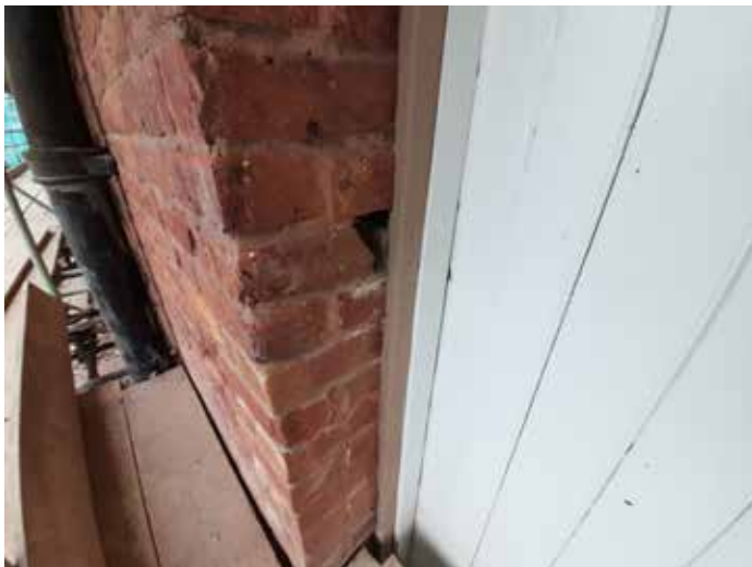
A1036: Broken brick. Brick repair required
