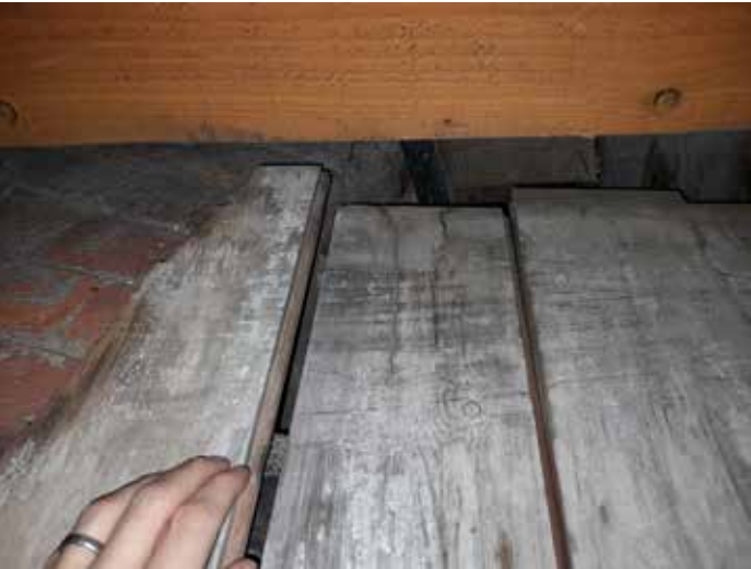
A0004: Loose floorboard. Re-fix / Repair / Make good
