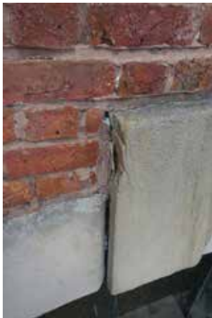
Material loss to keystone. Indent repair to stone block. Repoint using lime mortar.
