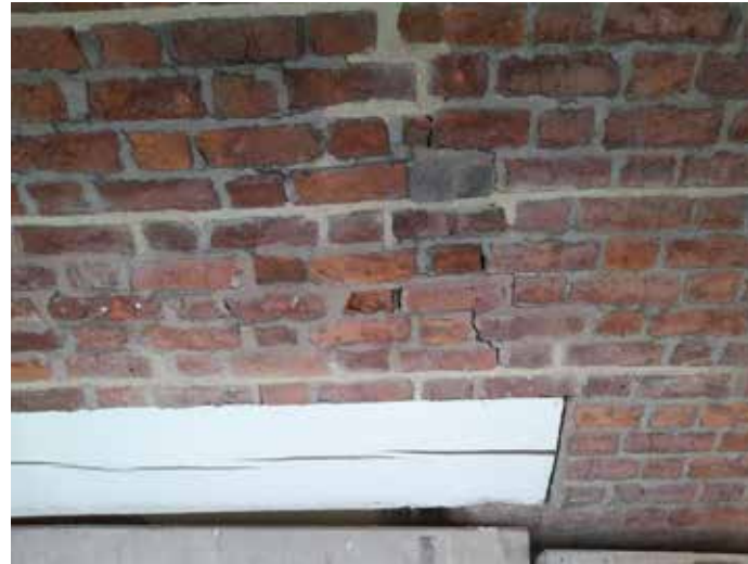
A1014: Movement in brick. Brick repair required
