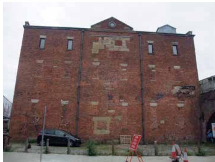
A1022.1: Forecourt area hardcore - rough surface with vegetation, water leak damp from overflowing (hopper blocked by vegetation). Clean/ replace RWP to Viaduct.
