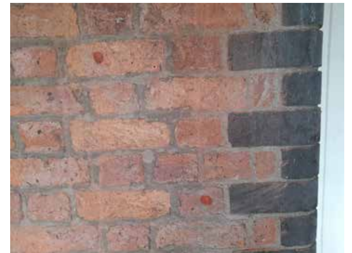
A1008: Poor repair. Repair brick repairs with brick dust
