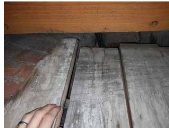
Loose floorboard. Re-fix, repair , make good.
