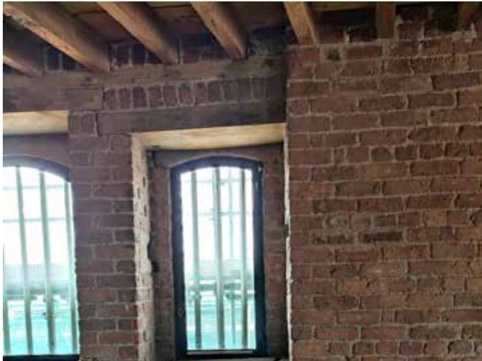
A0078: Brickwork damaged. Re-point check brick movement and repair
