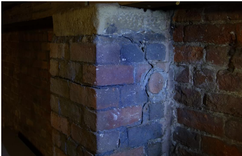
Photograph 02 – Vertical cracking through a primary beam support pier at the South wall at basement level.
