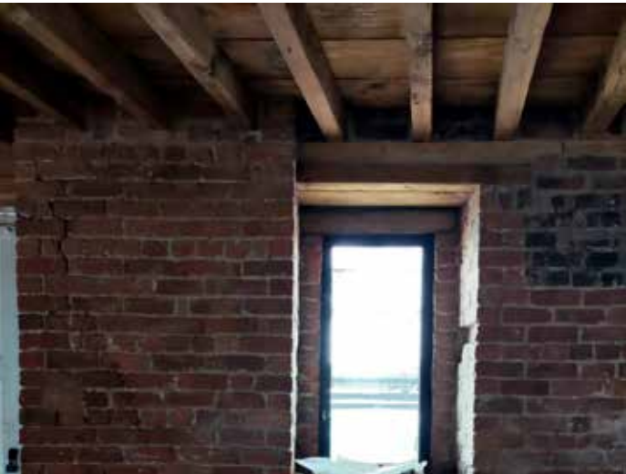
A0028: Brickwork damaged. Brick repair required
