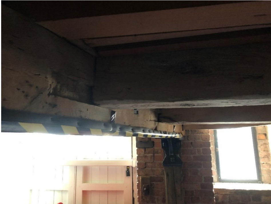
Photograph 09 – View of limited bearing of floor joist on floor beam, and brick cracking beyond.
