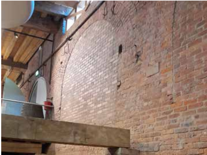
A0083. Defective pointing. Re-point
