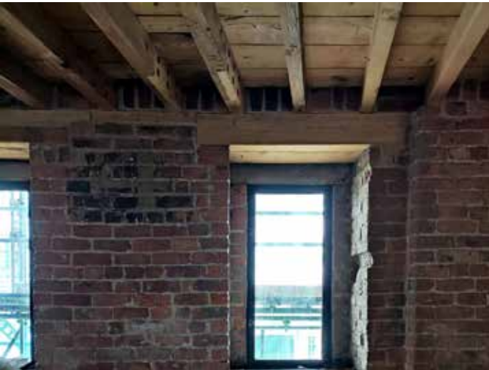
A0029: Brickwork damaged. Brick repair required
