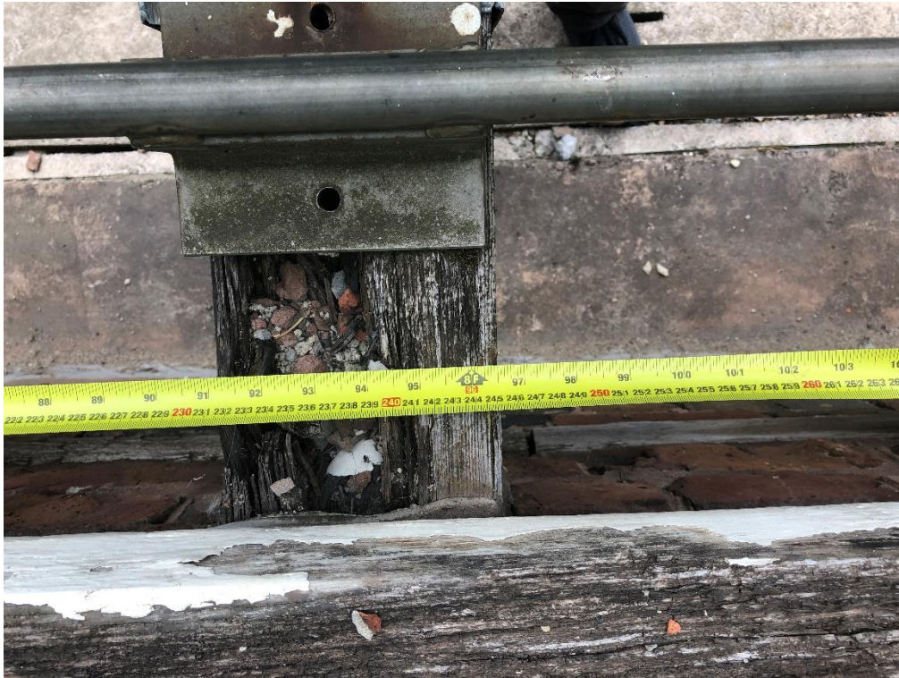
Photograph 7: Typical example of decay to floor joist projection
