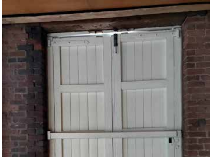
A0082. Defective pointing. Re-point
