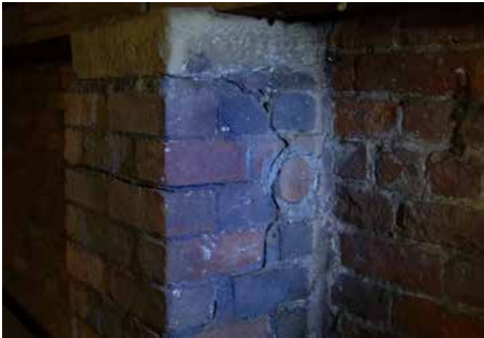
Vertical cracking through a primary beam support pier at the South wall at basement level.
