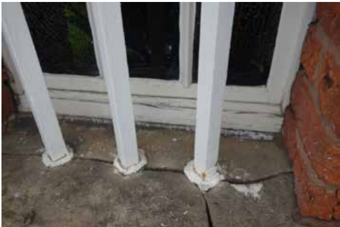
Corrosion of iron bar ends and cracks to cill. Cut out around bar embedments and treat iron. Repoint cracks using lime mortar.
