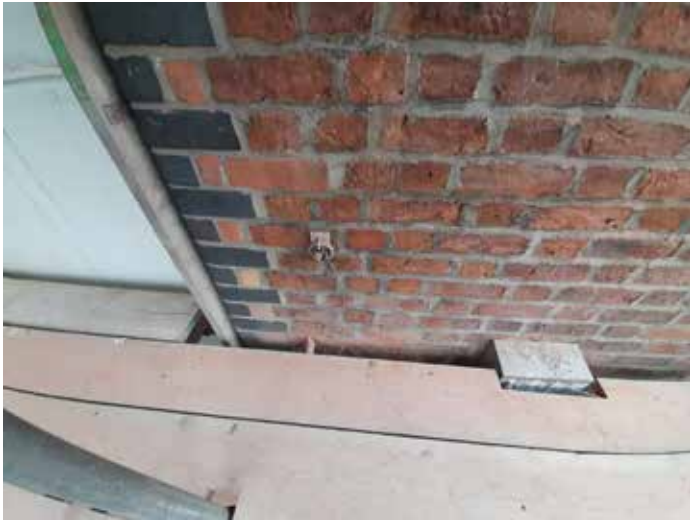
A1028: Metal fixed to wall. Remove redundant metalwork and fill hole with brick dust
