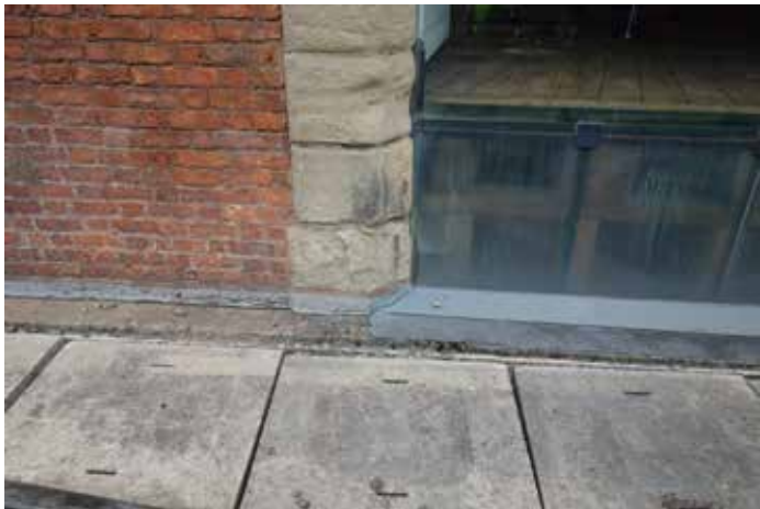
Material loss/spall. Indent repair to stone block.
