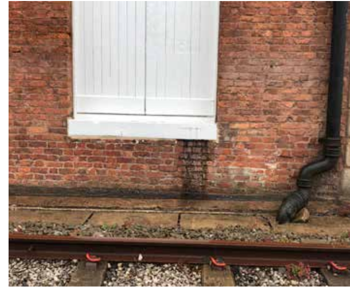
Visible staining to brickwork due to absence of any drip.
