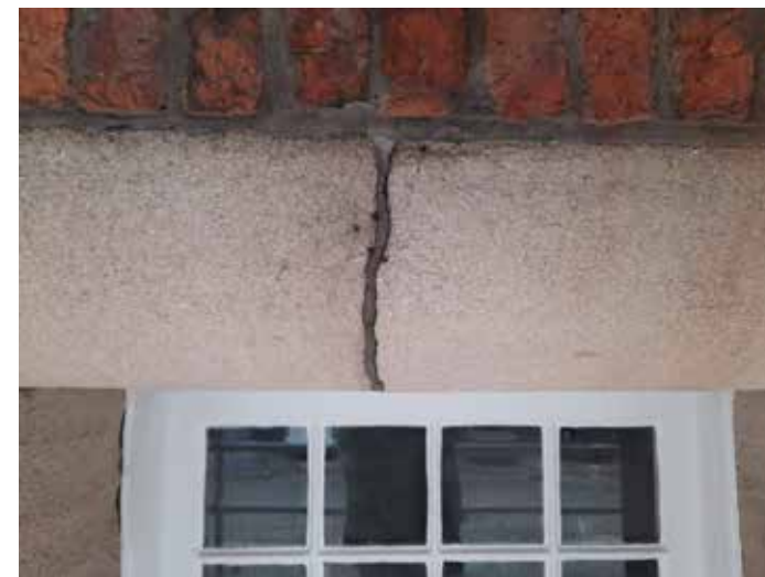
A1007: Lintel damaged. Structural engineer to review
