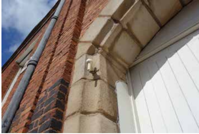
S1025: Spall at hinge fixing. Indent repair to stone block.
