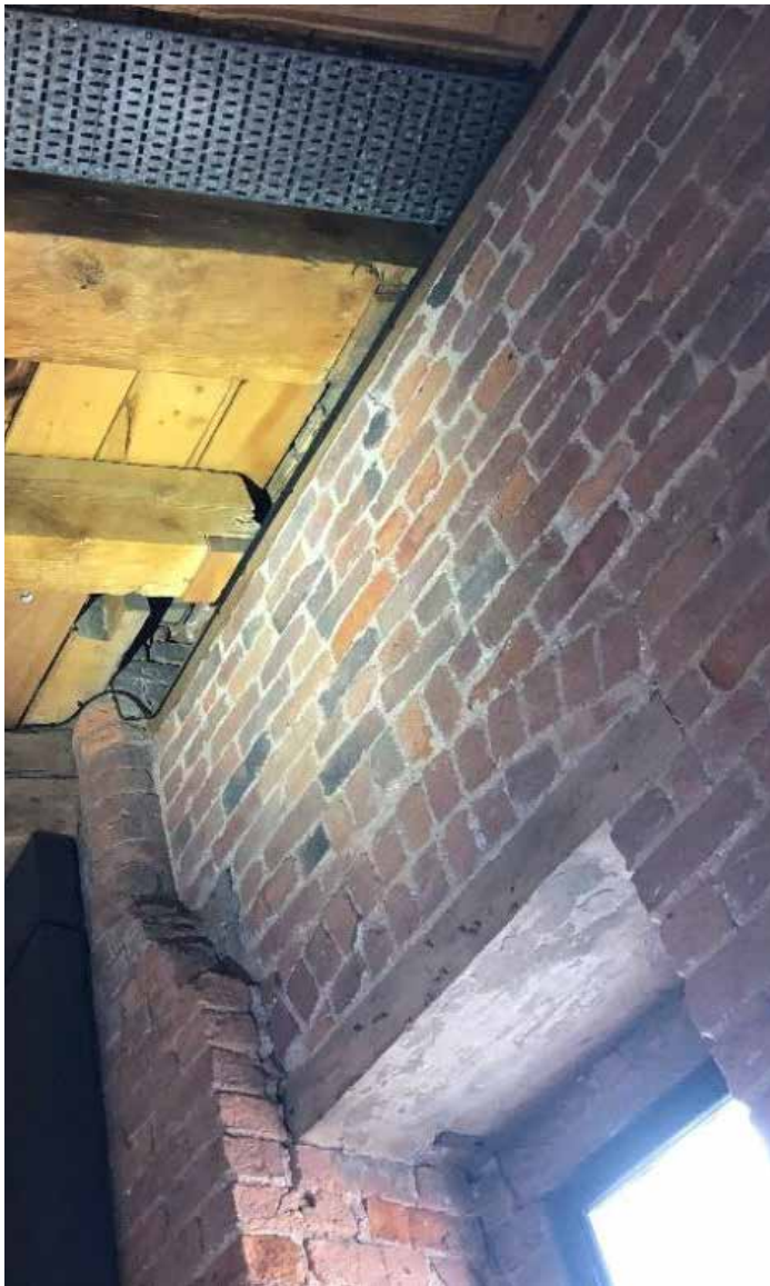
A full height photo of a ground floor pier at the inside of the north elevation, showing the extent of vertical cracking evident through bricks.
