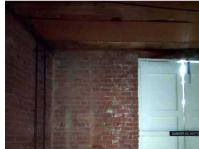
A0059: Wall stains. remove stains
