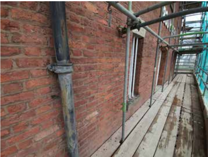
Heavily weathered rainwater downpipe
