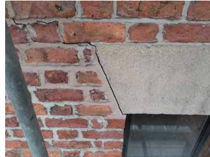
A1015: Lintel movement. Structural engineer to review
