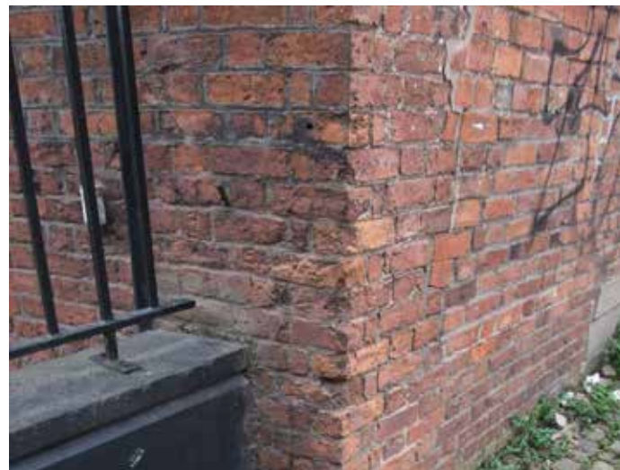
A1018: Damaged brick: Loss of brickwork at base. Loss of corners
