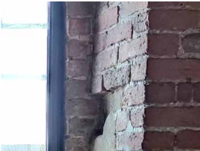
Missing masonry. Masonry repair required.
