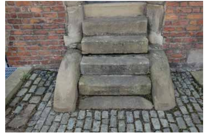
S1036: Settlement of steps. Dismantle and rebuild on new foundation.
