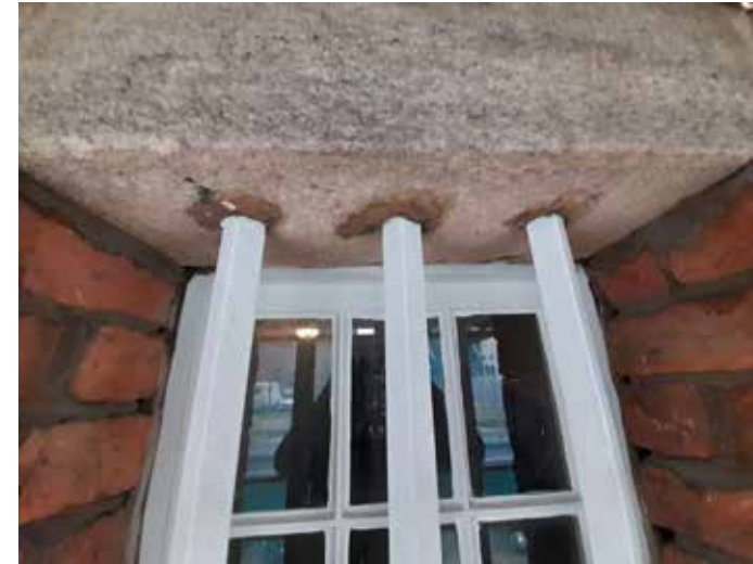
A1003: Lintel damaged. Lintel repair required, associated anti corrosion works to security bars.
