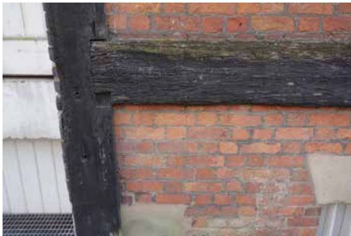
S1041: Vertical crack due to corroded fixing. Remove fixing and replace with stainless steel. Repoint crack with lime mortar.
