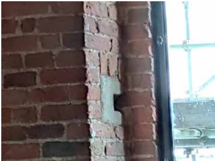
A0044: Brickwork damaged. Brick repair required
