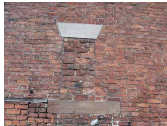
A1019: Extensive movement to brickwork, loss of mortar under timber lintel. Check lintel stability and repoint
