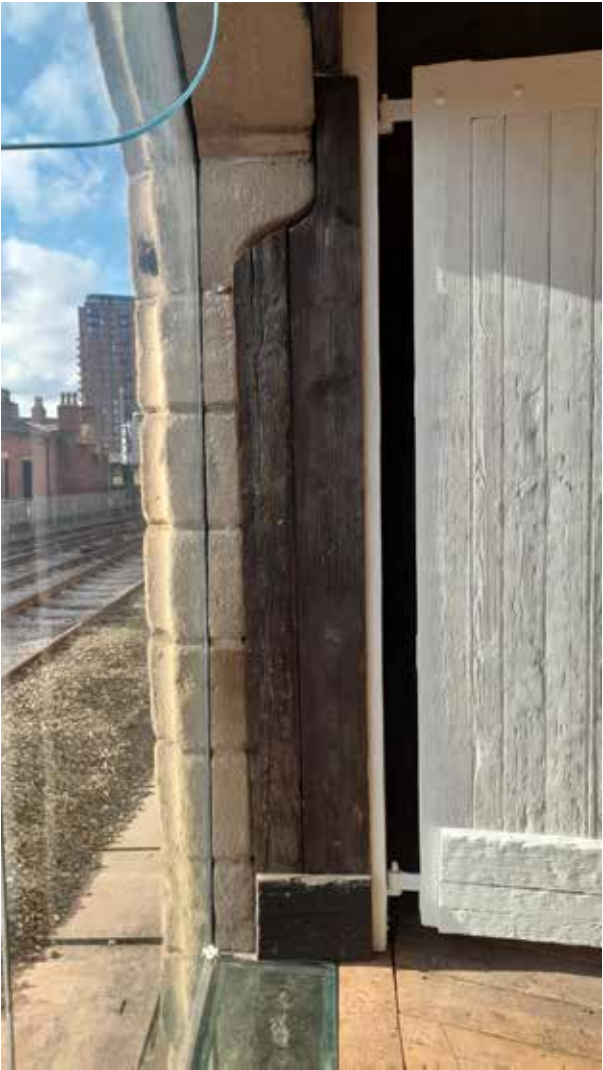
The glazing detail is very similar to the failed detail at Bay 1
