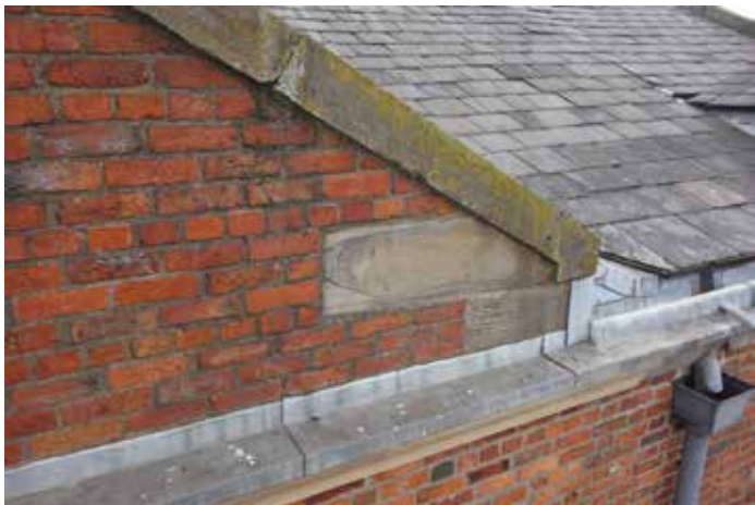
S1067: Delamination of RHS pediment block face. Indent repair to restore lost section.
