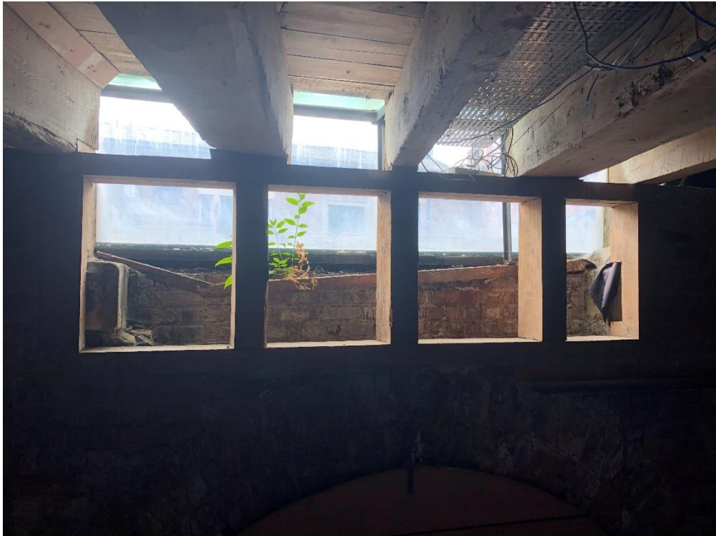
Photograph 2: General internal view showing the floor joists cut back and re-supported on a new sub-frame. The decayed sill is visible beyond.
