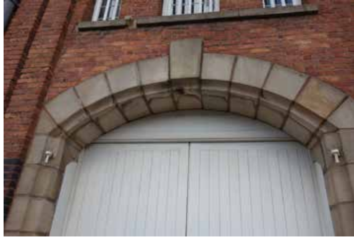
S1026: Spall at hinge fixing. Indent repair to stone block.
