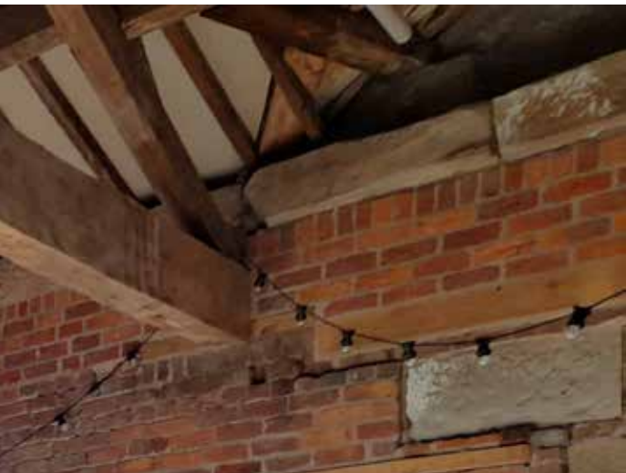
A0015: Brickwork damaged. Brick repair required
