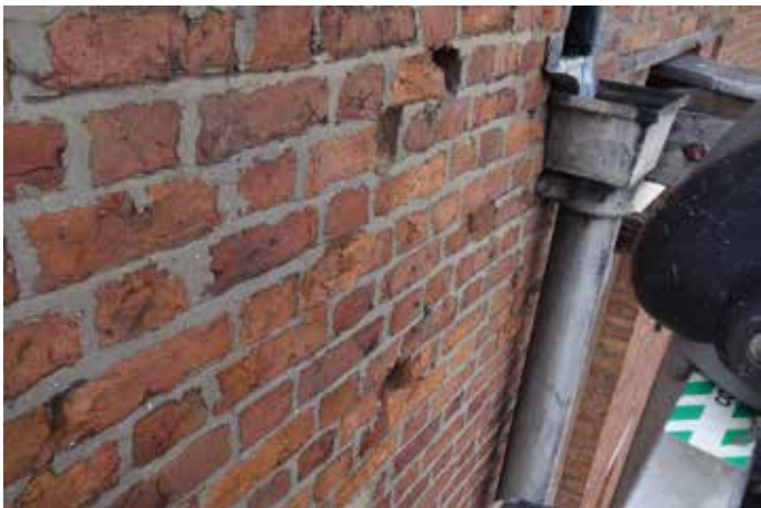
Spalled bricks. Cut out and replace bricks where erosion exceeds 15mm depth. Repoint using lime mortar.
