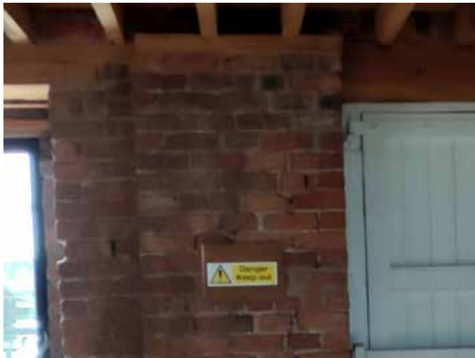
A0043 Defective pointing. Re-point
