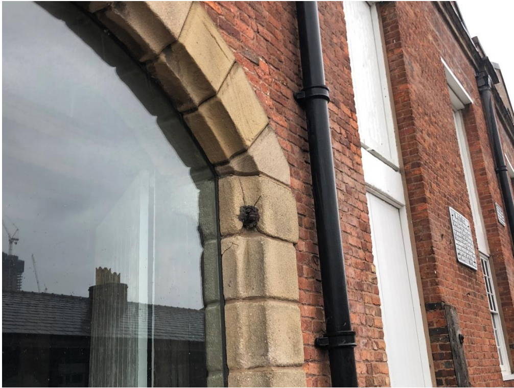
Photograph 10: Corroded historic hinge ironwork at Bay 3
