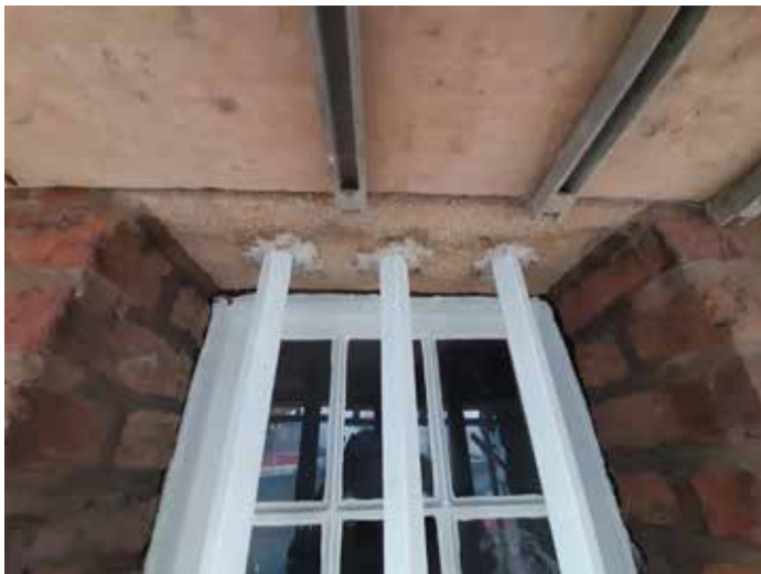
A1031: Lintel damaged: Header repair required. anticorrosion works to security bars, rub down and redecorate)
