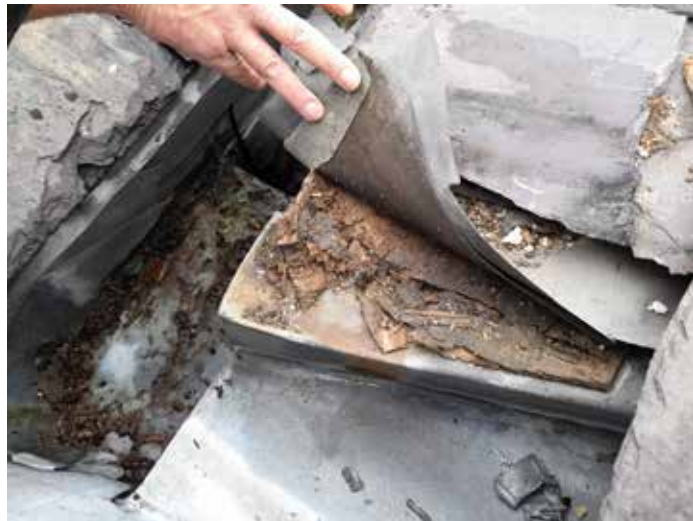
A1052: Valley gutter poor damp and friable. Timber repair required and make good. Slate battens or pegs to underside could be decay
