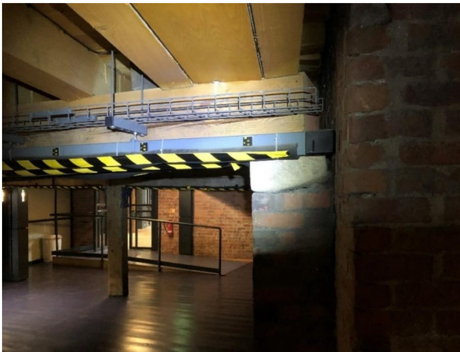
Photograph 08 – A photo of a ground floor pier at the inside of the Southern elevation, providing limited lateral restraint to the head of the wall.
