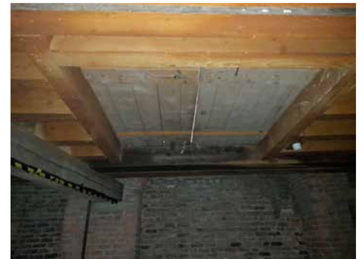
.Check stability. Review with Structural engineer. Reinforce
