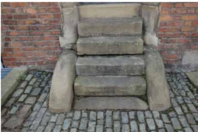
Settlement of steps. Dismantle and rebuild on new foundation.
