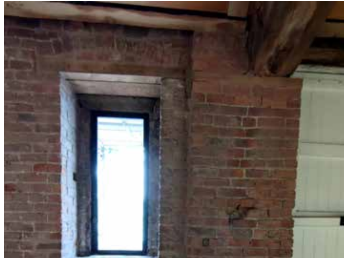
A0054: Brickwork damaged. Brick repair required
