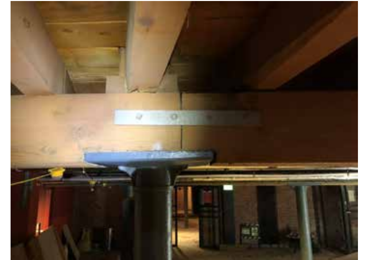
Floor beam 'but' connection off centre overcast iron columns. floor beam eccentrically loading cast iron plate.
