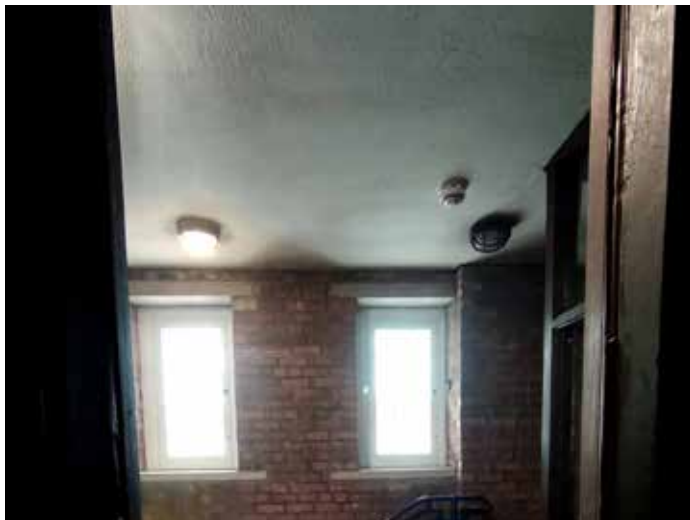
A0050: Brickwork damaged. Brick repair required
