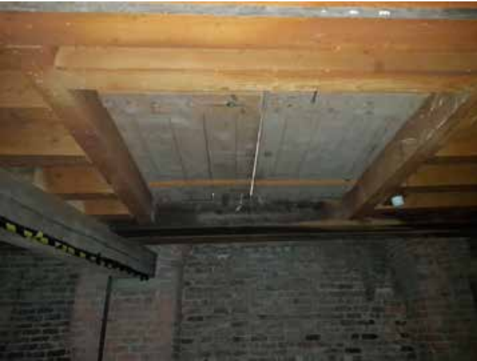
A0005: Check stability. Review with Structural engineer- Rein-force
