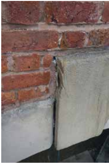
S1011: Material loss to keystone. Indent repair to stone block.
