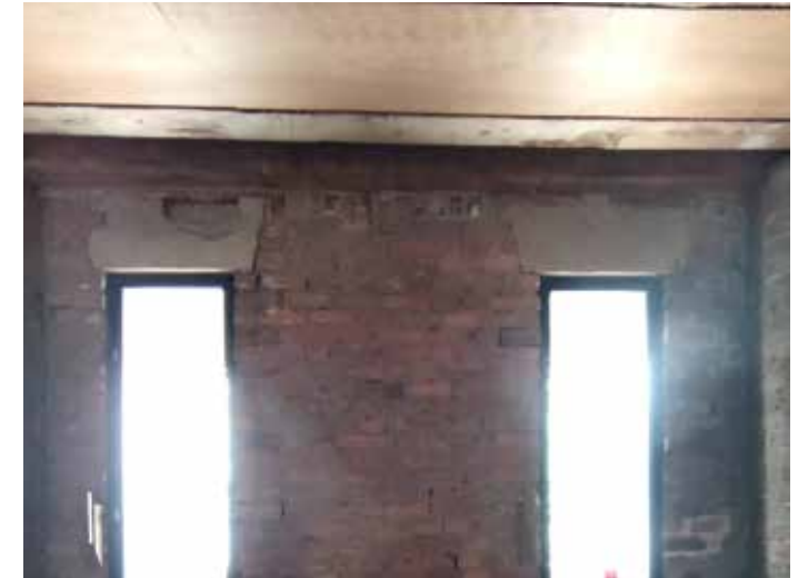
A0060: Stone lintel damaged. Repair lintel
