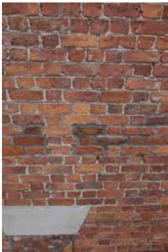
S1071: Diagonal cracks, 2mm width. Repoint using lime mortar.
