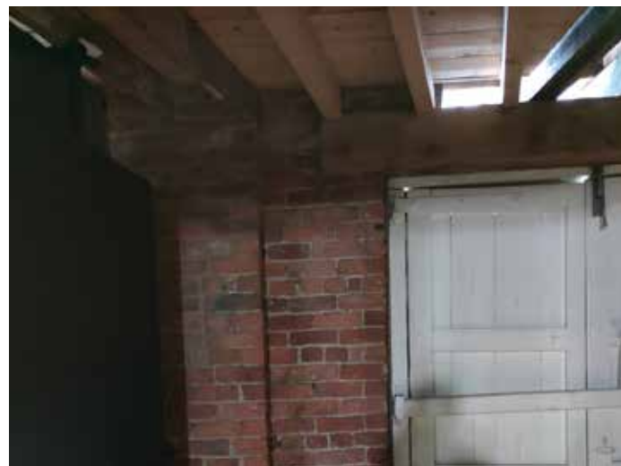
A0071: Brickwork damaged. Brick repair required
