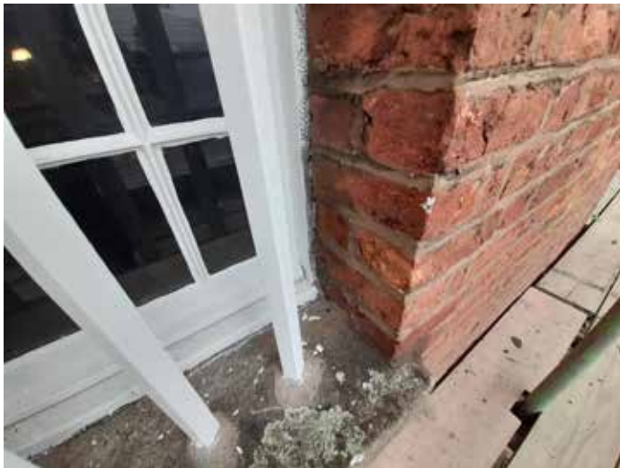
A1030: Sill damaged. Sill repair required. Associated anticorrosion works to security bars, rub down and redecorate)
