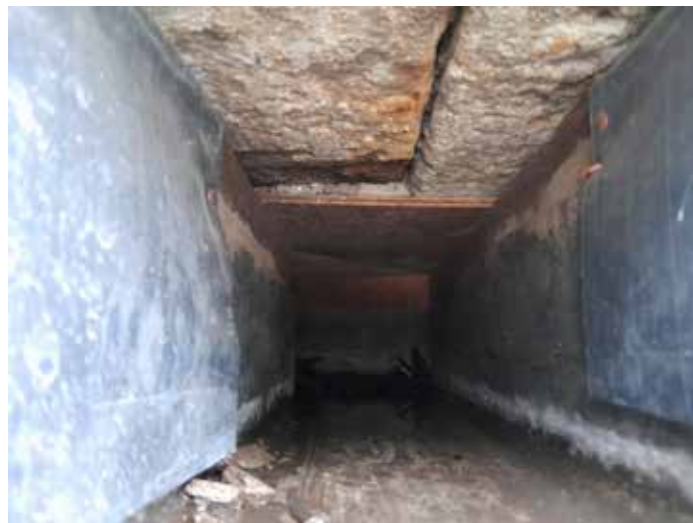
A1017: Damaged leadwork. Replace lead lining to chute (generally)
