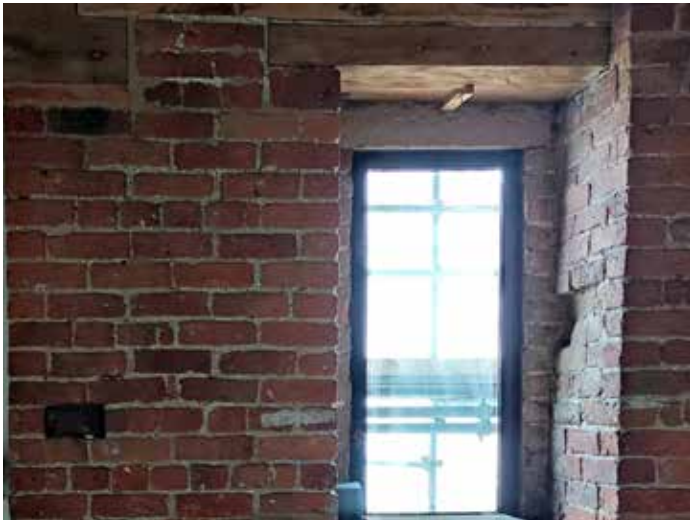
A0032. Brickwork damaged. Brick repair required
