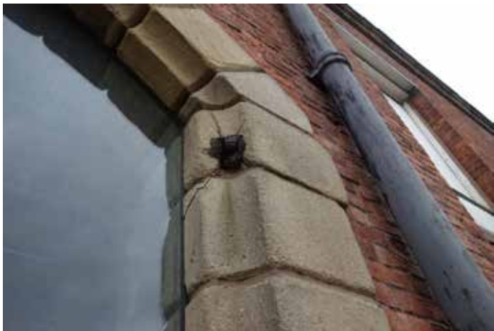
Crack/spall to block at hinge fixing. Treat ironwork, indent repair to stone block.
