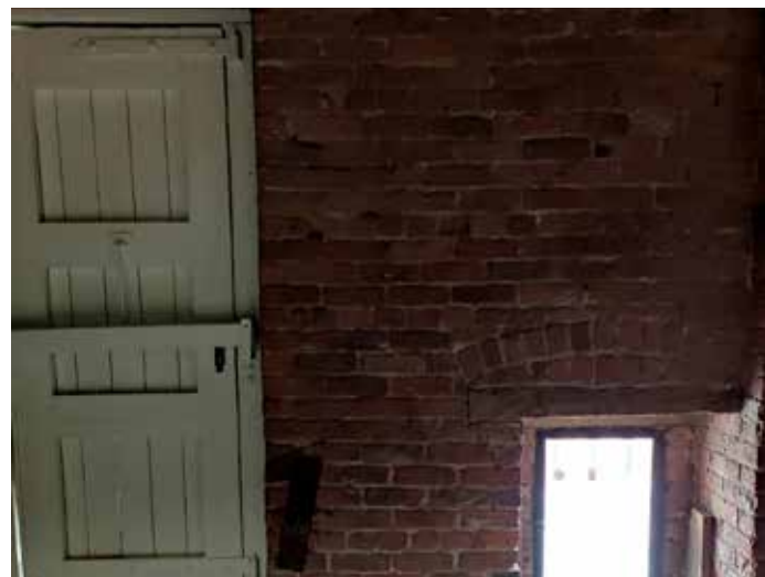
A0067: Wood piece fixed to wall. Remove and replace with salvaged brick
