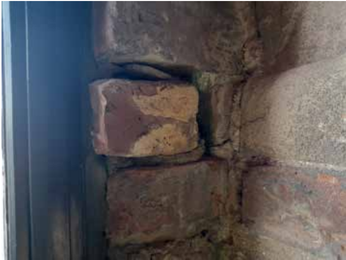
A0013: Damaged brick. Repair brick required
