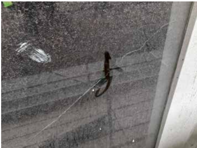
A1038: Cracked glazing. Replace glass or coat in anti-shatter film.
