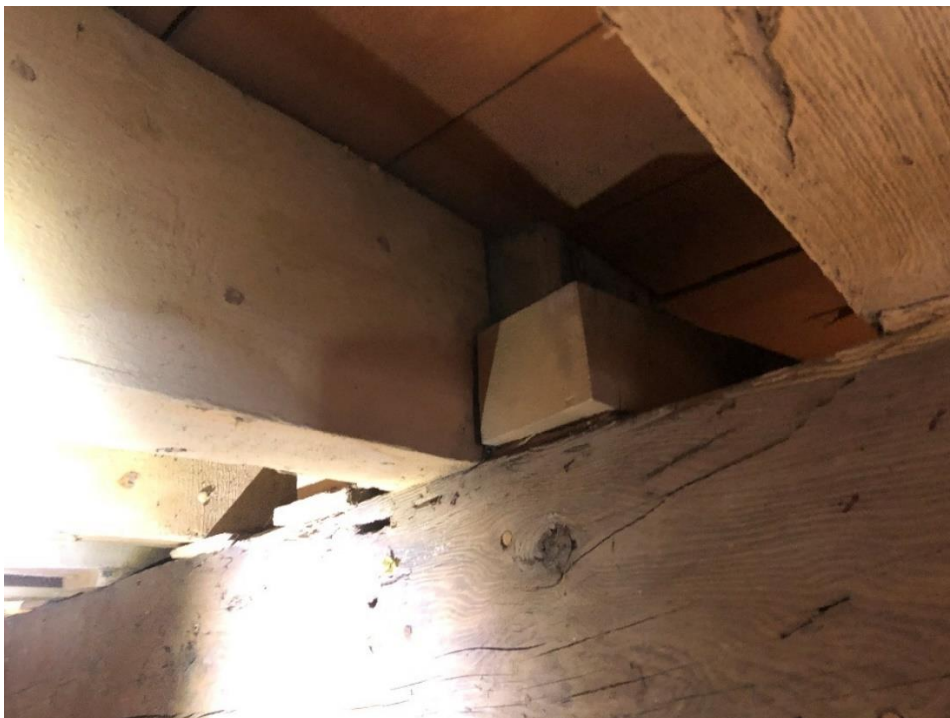
Photograph 03, 04: limited bearing of timber floor joist.
