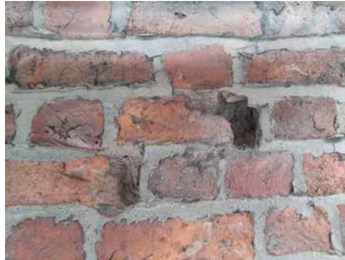
A1002: Damaged Brick. Brick repair required
