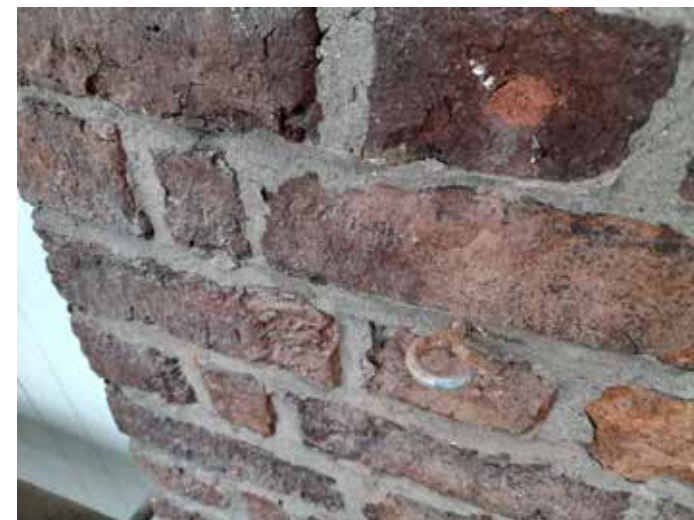
A1011: Metal hooks fixed to wall. Remove hooks and repair
