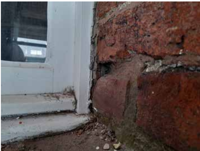
A1039: Defective pointing: Repoint
