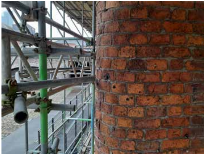
A1029: Metal sockets inserted to wall. Remove sockets
