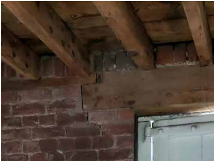
Brickwall crack. Brick repair required.
