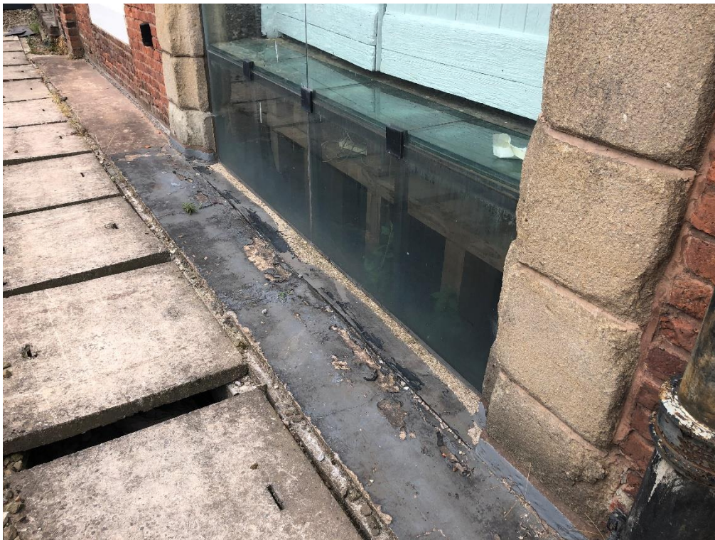
Photograph 1: General view of the lower part of the glazing externally showing sill/base flush with the external ground level.
