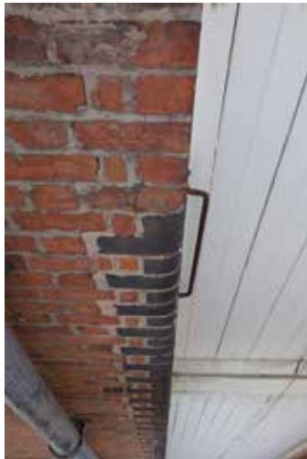
S1045: Vertical crack, 1-2mm width Pin bricks with Cemties. Repoint crack with lime mortar
