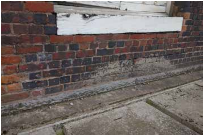
Patches of eroded pointing. Repoint using lime mortar.
