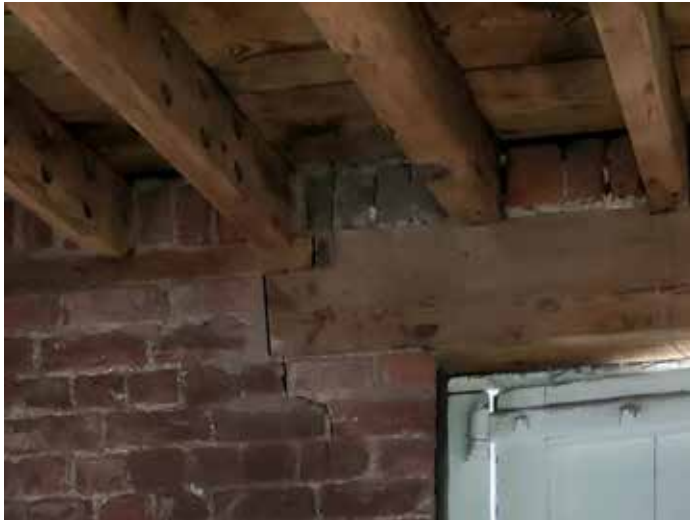
A0025. Brick wall crack. Brick repair required
