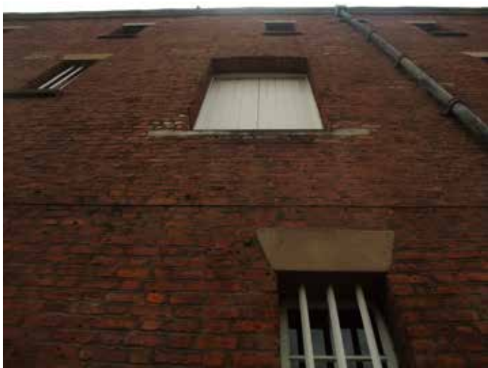
A1026: No drip detail to concrete sill, stain to brick below. Replace concrete sill.
