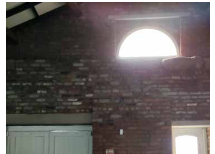
A0069: Wall stains. Remove white stains to wall
