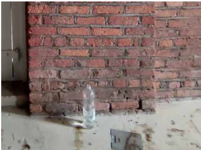
A0051 Defective pointing. Re-point
