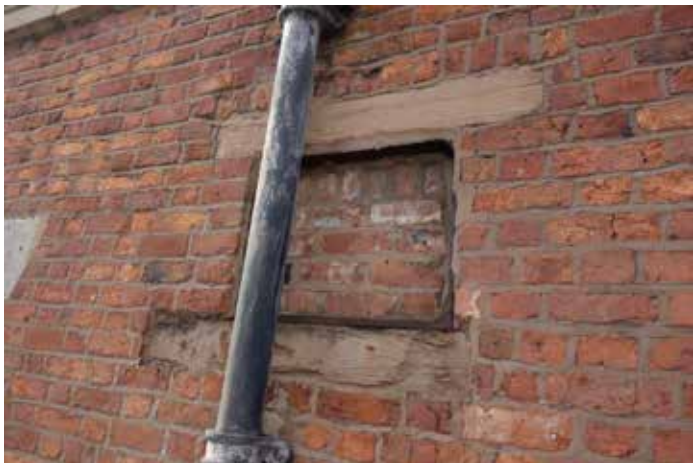
Metal duct frame is corroded. Cut out and brick in the opening. Material loss/spall. Indent repair to stone cill.
