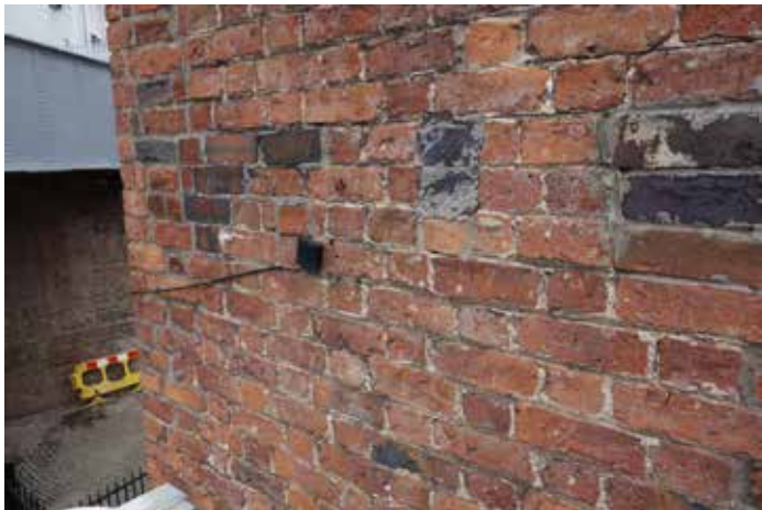
West elevation. Multiple vertical cracks in brickwork.Repair using helical bar stitching. Repoint using lime mortar.
