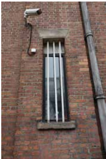
S1059: Corrosion of iron bar ends and cracks to cill and lintel. Cut out around bar embedments and treat iron. Repoint cracks using lime mortar.
