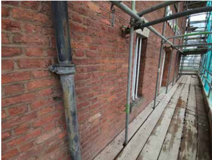
A1027: Damaged RWP. RWP to be redecorated or replaced
