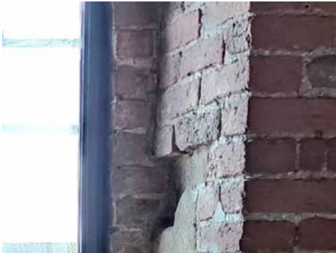
A0031: Missing masonry. Masonry repair required
