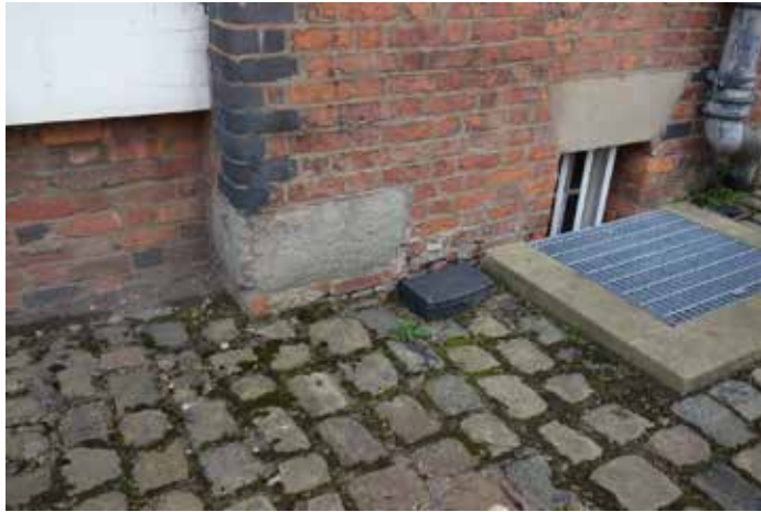
S1037: Patches of eroded pointing. Repoint using lime mortar.
