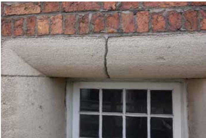
Vertical crack, c7mm width.Repoint using lime mortar.
