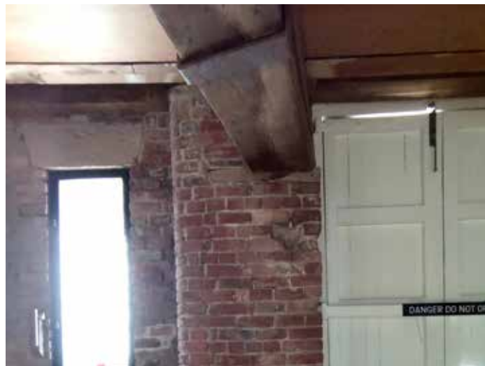
A0061 Brickwork damaged. Brick repair required
