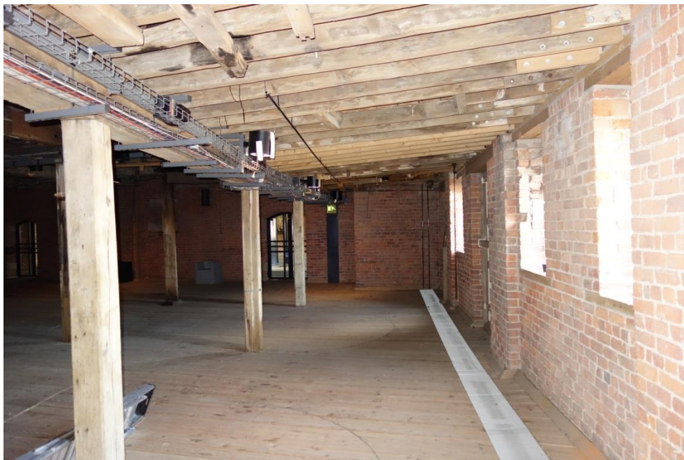
Photograph 17, 18 – View from first (16) and second (17) floor level of general depression in floor level
