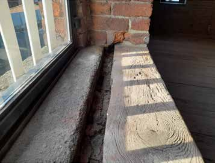
A0016: Damaged timber or deteriorate. Repair sill (historic detail)
