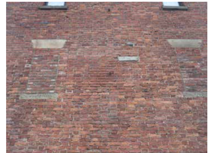
A1020: Vertical line of metal brackets, poor pointing in brick. Remove metal fixed to wall and repoint
