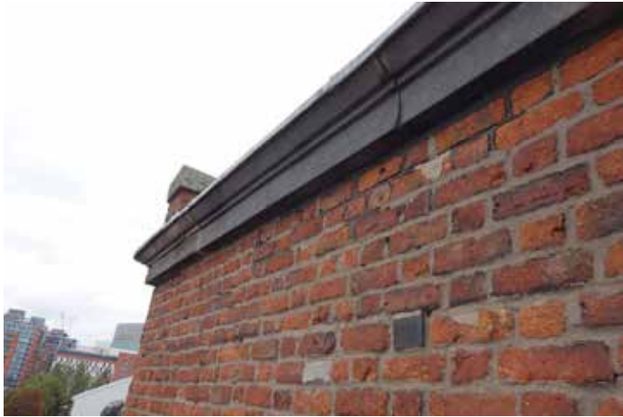
S1063: Open joints to cornice. Repoint using lime mortar.
