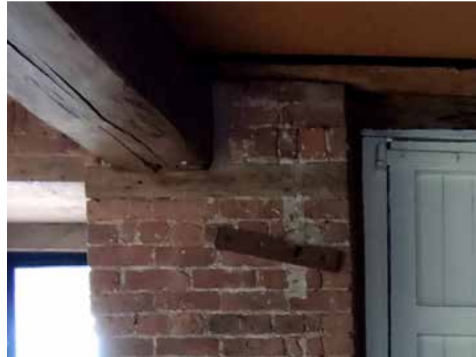
A0055.1: Defective pointing. Re-point
