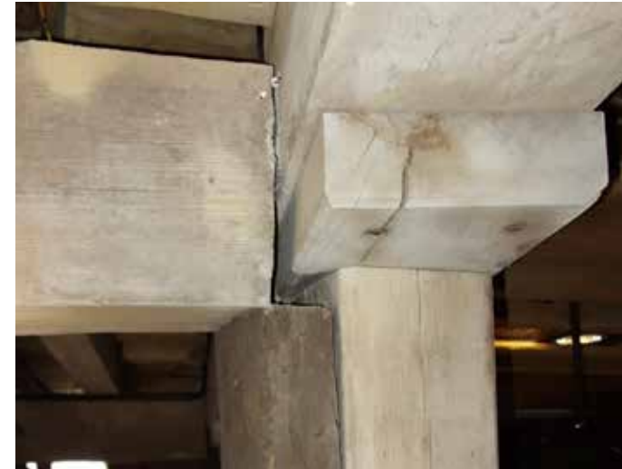
View from ground floor mezzanine of east west beams with limited bearing on vertical plate. Vertical plate bolted to column using single M20 bolt. Shrinkage and frame racking has pulled the timber off this bearing and it now very little contact remains.
