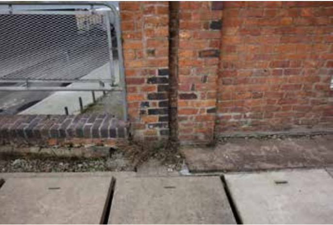
S1001: Patches of eroded pointing. Repoint using lime mortar.
