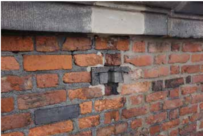
Decayed embedded timber. Remove timber and brick-in void.
