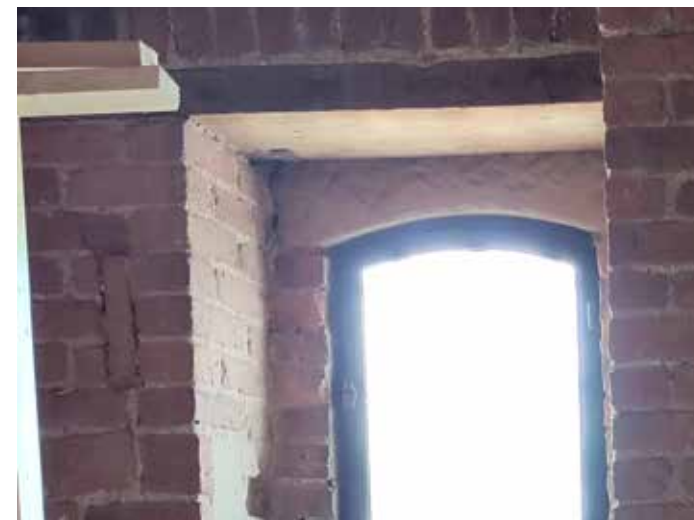
A0072: Brickwork damaged. Brick repair required
