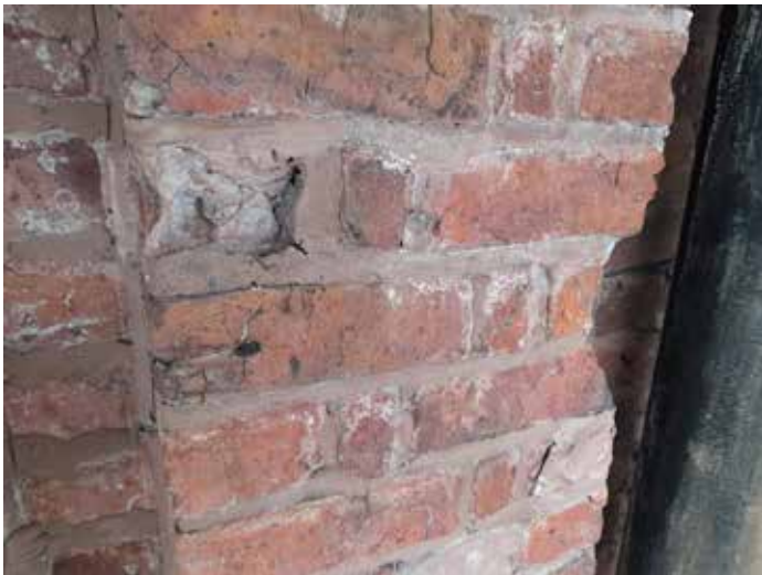
A1034: Damaged brick. Brick repair required
