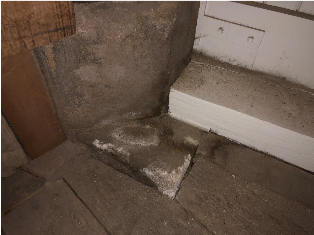
Photograph 12: Water staining internally at the Bay 4 door opening.
