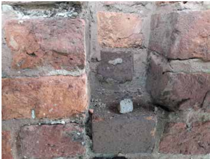
A1044: Defective pointing: Repoint
