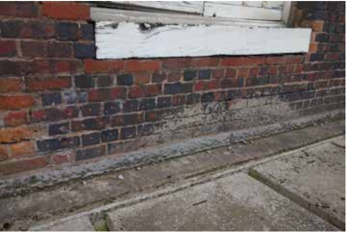
S1004: Patches of eroded pointing. Repoint using lime mortar.
