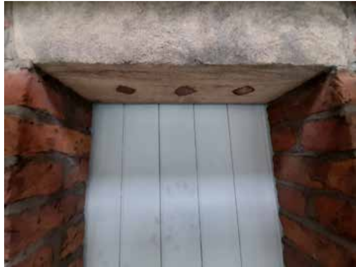
A1013: Lintel damaged. Header brick repair required
