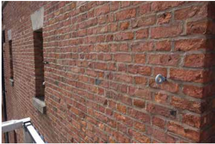
S1033: Various redundant metal bolts and fixings. Remove and infill holes using lime mortar.
