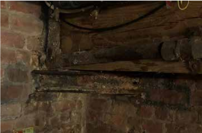
Looking at the southwest corner. corrosion in corner support to ground floor timber floor beam
