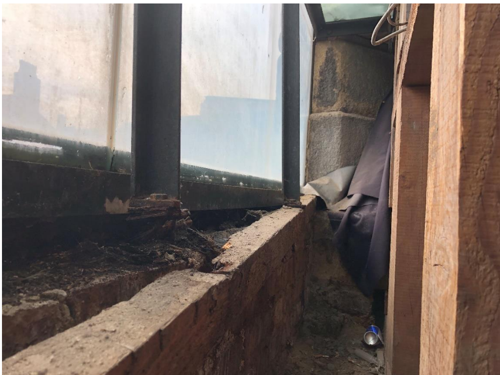
Photograph 3: Detail view showing severe timber decay to the sill.
