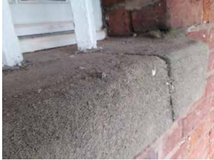
A1041: Sill damaged. Sill repair required
