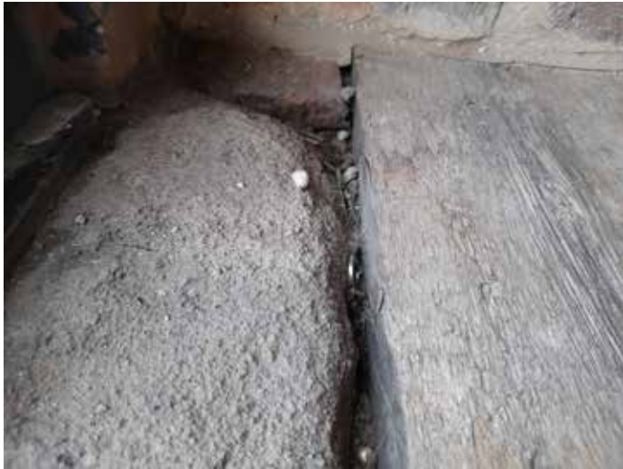
A0012: Damage timber. Repair sill (historic detail)
