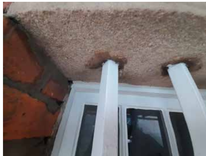
A1006: Lintel damaged. Header head repair required
