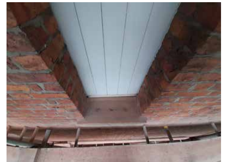
A1012: Sill damaged. Sill repair required
