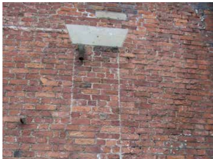
A1021: hole at lower right of GFL infilled window, extensive cracking to brickwork, loss mortar, mid-left iron protruding. Brick repair required
