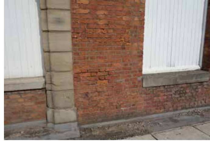
S1027: Patches of eroded pointing. Repoint using lime mortar.
