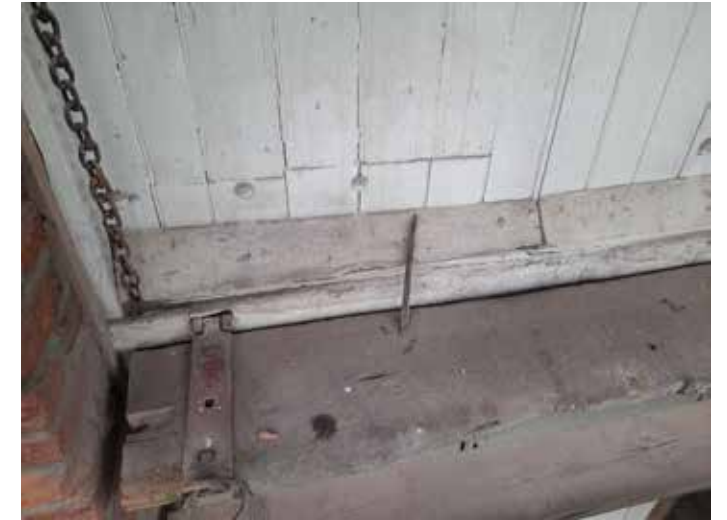
A1016: Loose sill. Check sill stability/replace sill (historic detail)
