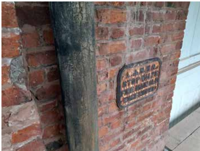
A1035: Damaged brick. Brick repair required
