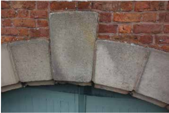
S1003: Open joint at keystone. Repoint using lime mortar.
