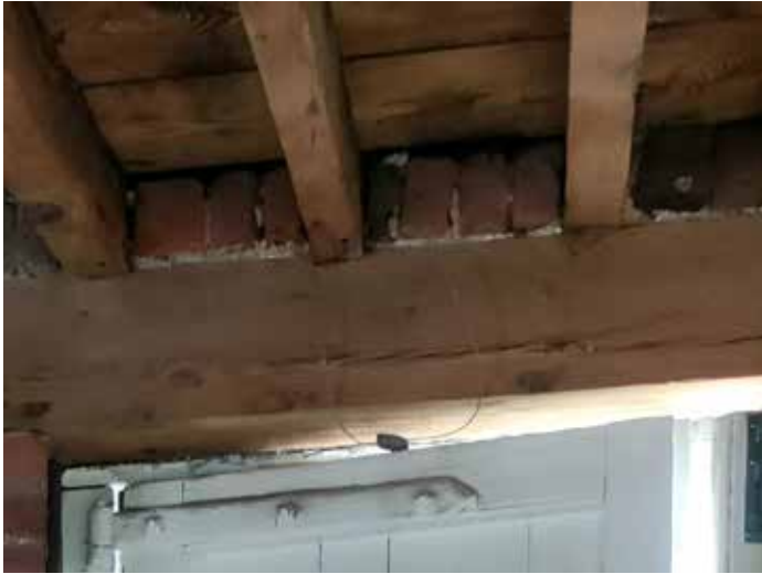
A0026: Defective pointing. Re-point
