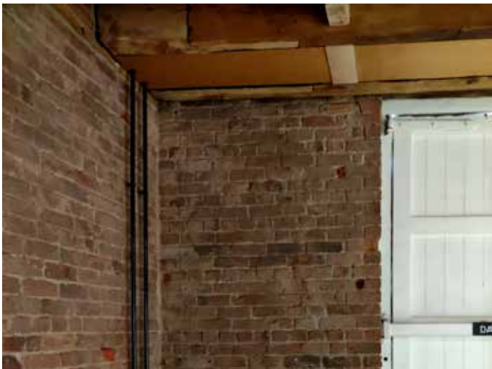
A0053 Brickwork damaged. Brick repair required
