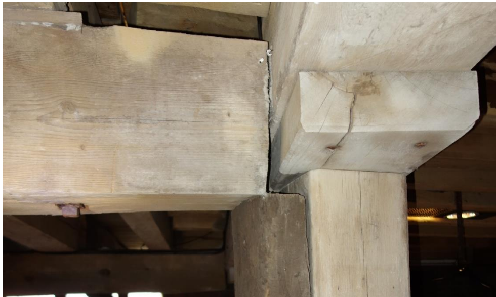
Photograph 11, 12 – View from ground floor (11) mezzanine (12) of east west beams with limited bearing on vertical plate. Vertical plate bolted to column using single M20 bolt. Shrinkage and frame racking has pulled the timber off this bearing and it now very little contact remains.
