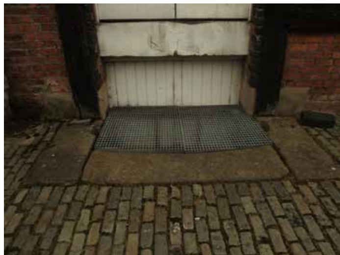
A1009: Stone step worn, grating is not level. Level grating
