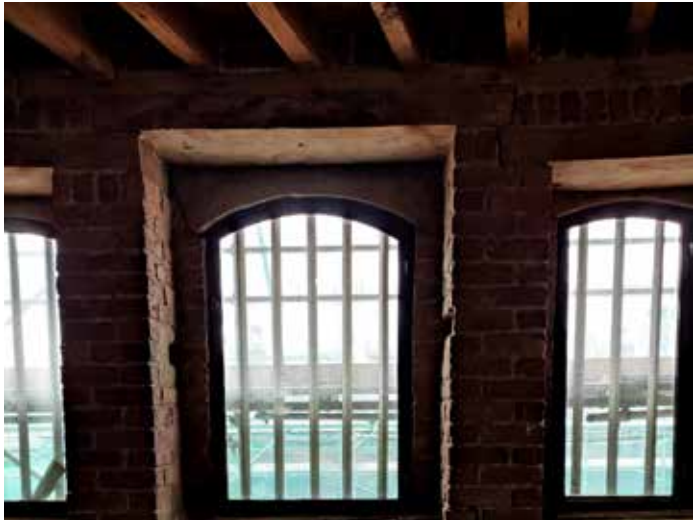
A0077: Brickwork damaged. Brick repair required
