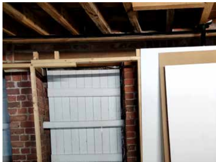
A0070: Loose sill. Check sill stability and repair.
