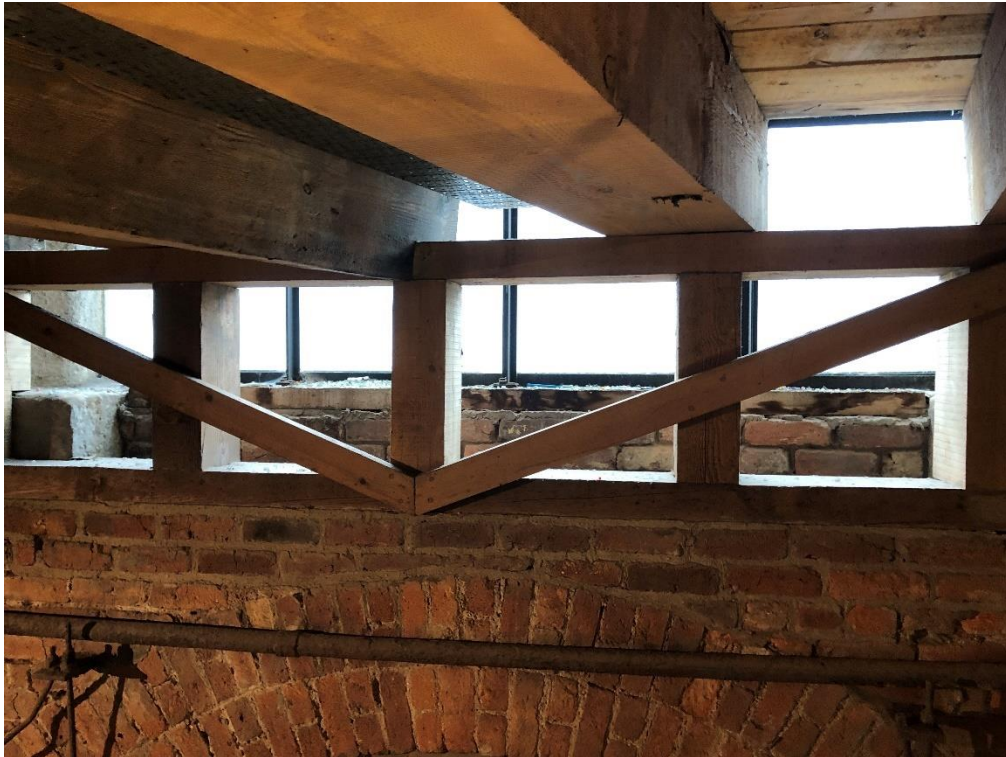
Photograph 9: General internal view of glazing support and floor framing arrangements at Bay 3 showing water staining to the timber support at the base of the glazing.
