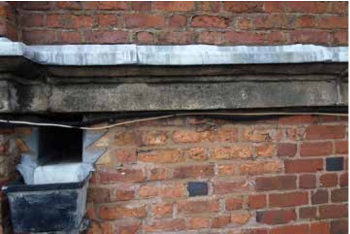
S1008: Bolt shell and adjacent spall. Remove bolt shell and undertake indent repair to cornice.
