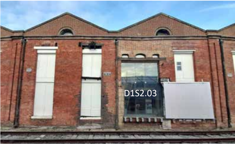
Wagon Arch D1S2.03 Externally: • Glass window_double height. • Straight wood lintel to head, • Stone reveal in part, brick reveal. • Decayed cut short joist ends • Brickwork below sill
