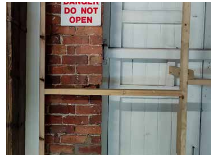
A0073: Brickwork damaged. Brick repair required
