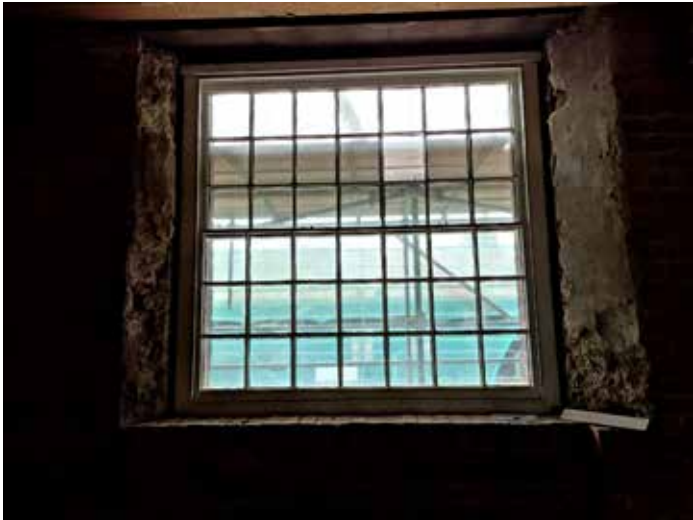
A0080: Damaged window reveal. Repair window reveal.
