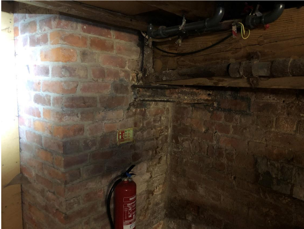
Photograph 01: Looking at the southwest corner. corrosion in corner support to ground floor timber floor beam
