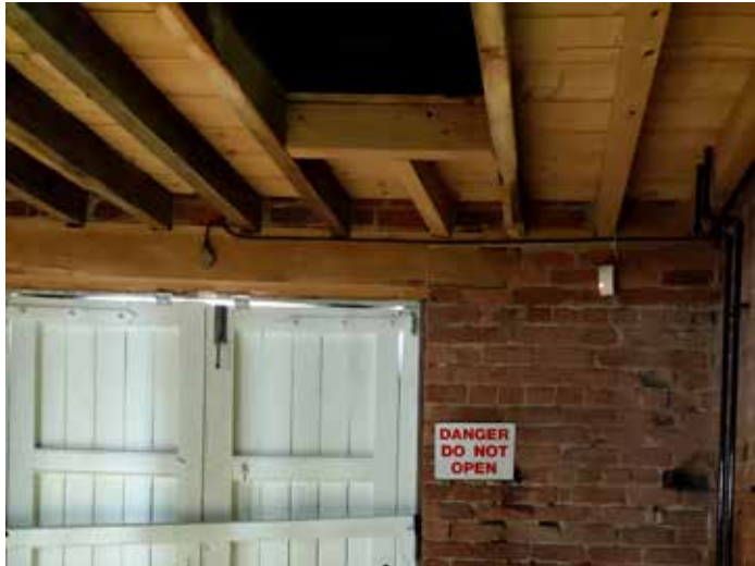
A0076: Defective pointing. Re-point
