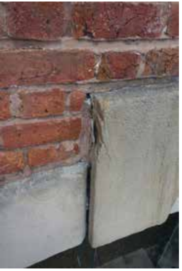
S1012: Open joints at keystone. Repoint using lime mortar.
