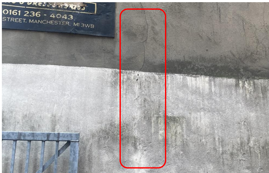
Photo 7. Vertical cracking to right-hand (west) gable wall
