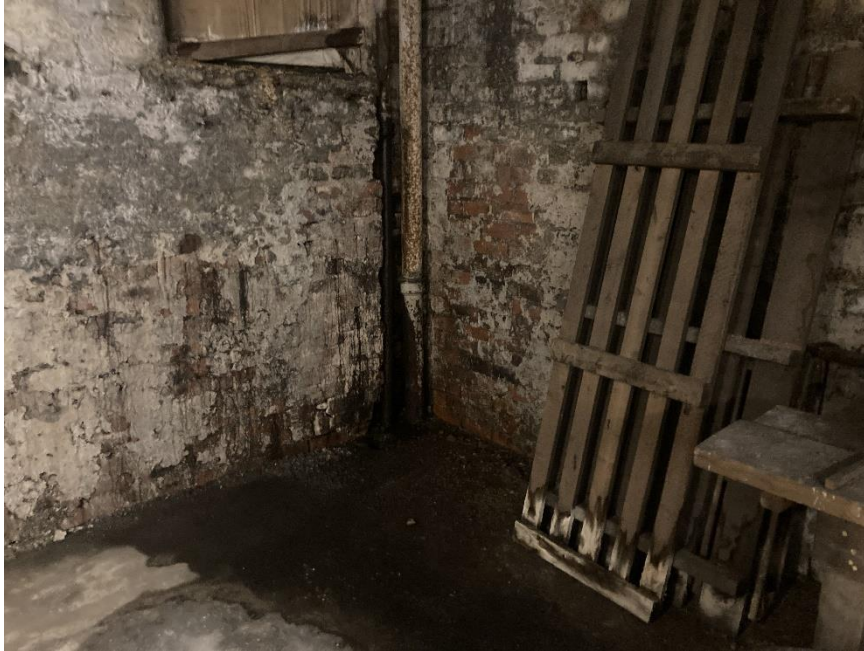
Photo 14. Basement water ingress through rear elevation
