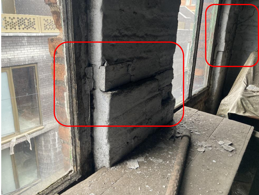
Photo 24. Structural movement to masonry piers at second-floor level
