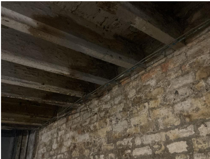
Photo 15. Ground floor joists appeared damp where built in to external walls
