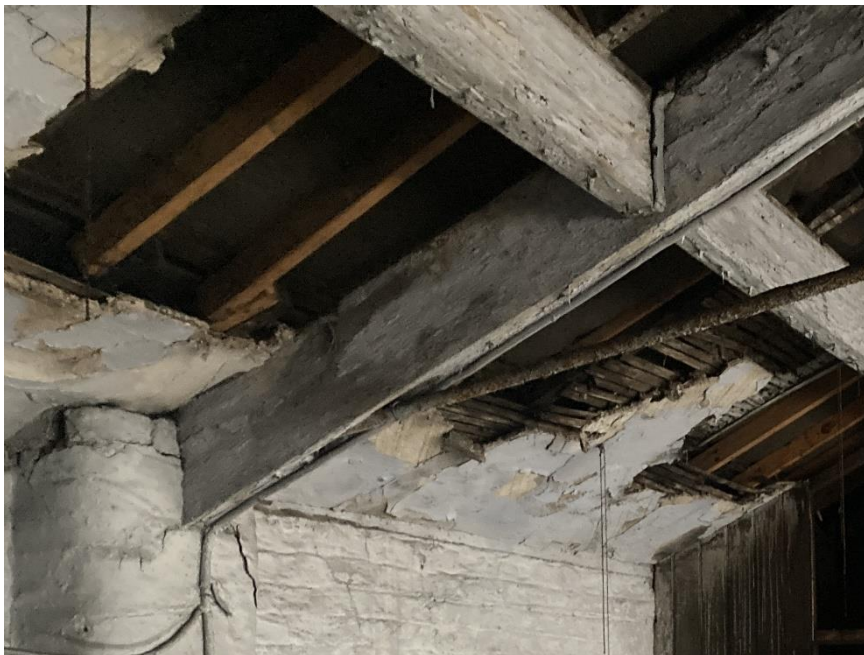
Photo 23. Previous damp conditions evident
