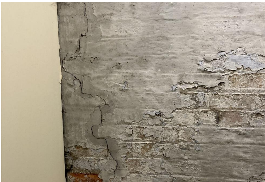
Photo 19. Internal cracking to south-west corner at first-floor level
