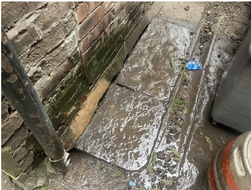
Photo 9. Saturated ground and RWP discharge adjacent basement corner
