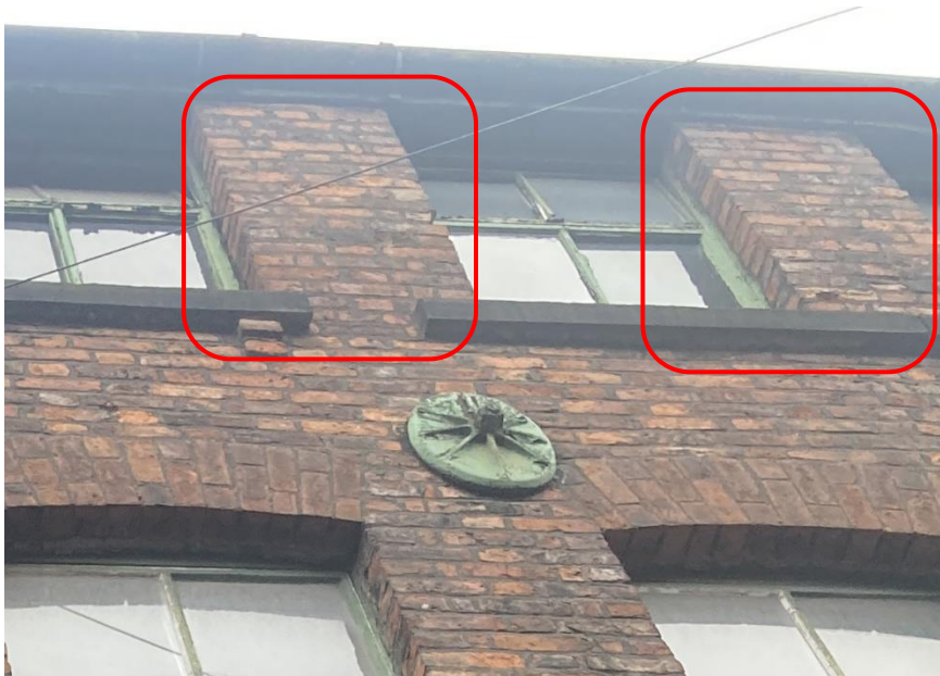
Photo 5. Rotation of brickwork piers at second-floor level to front (north) elevation
