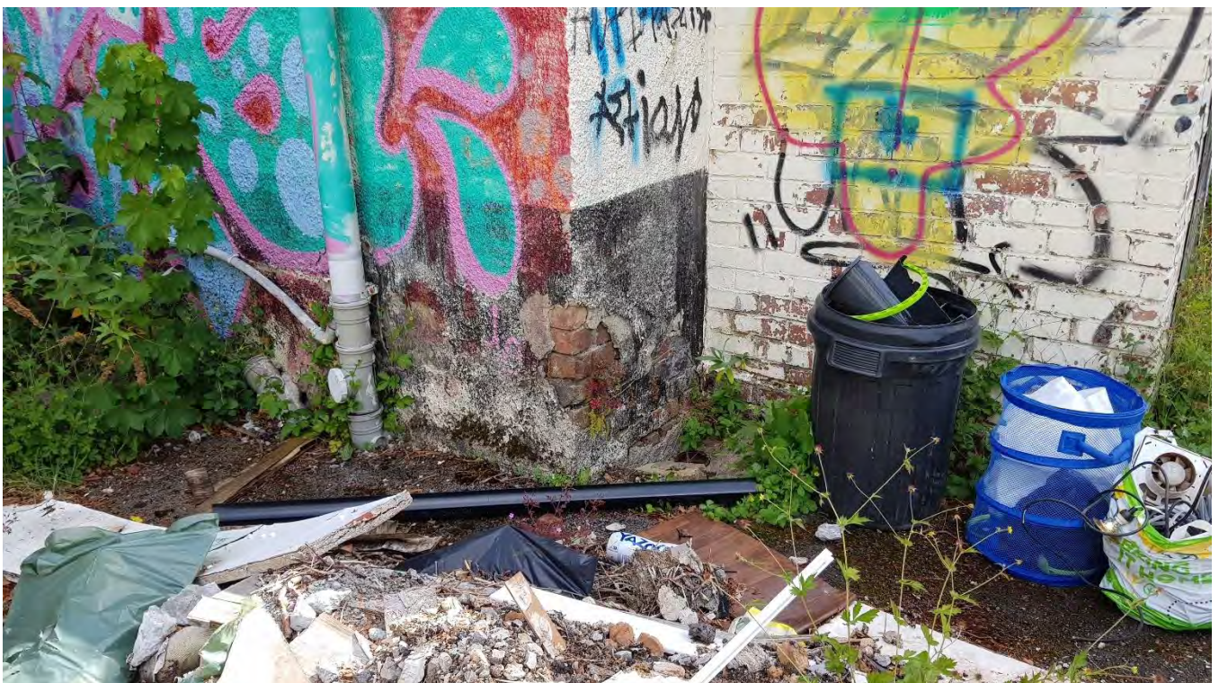
Loose render. Debris externally
