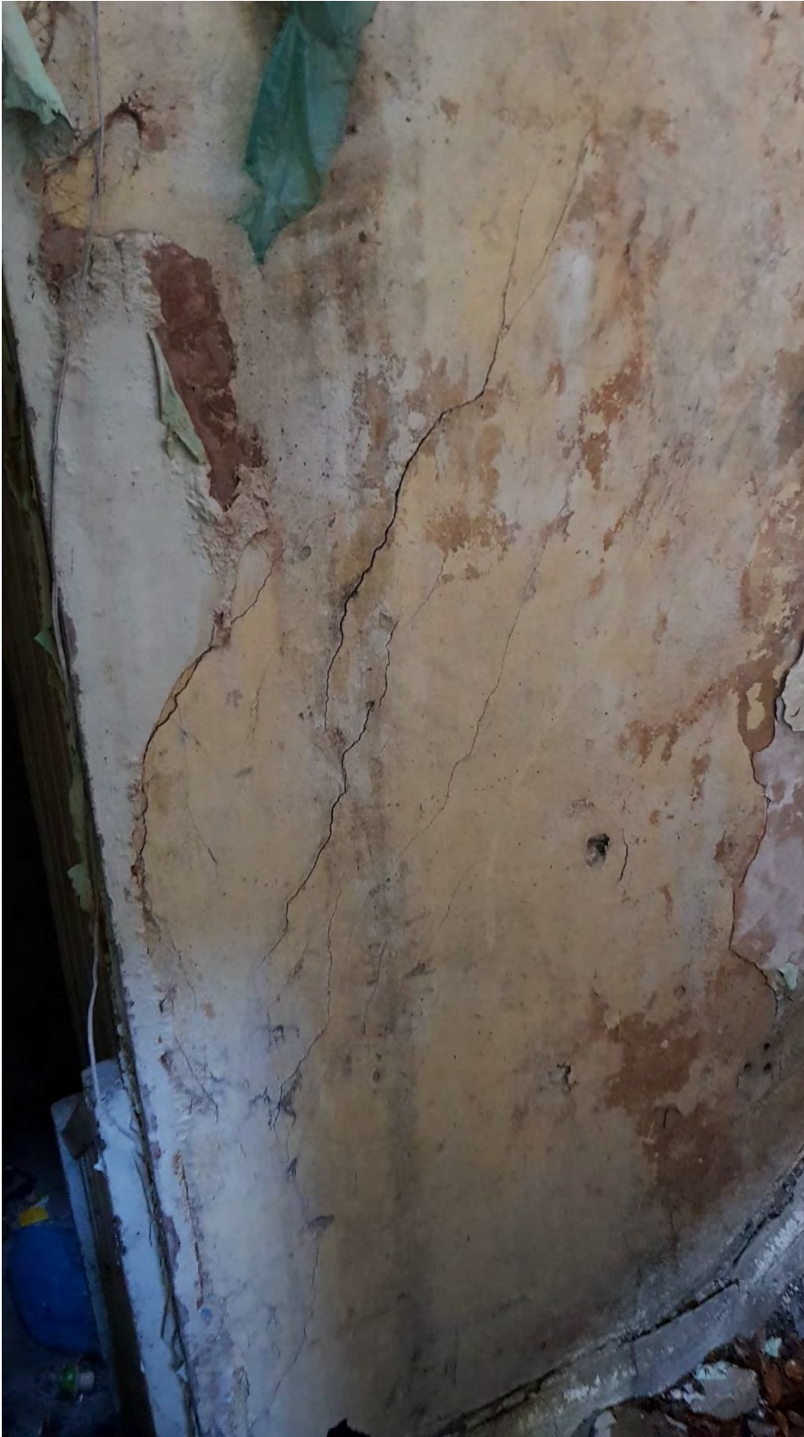
Cracking to internal walls
