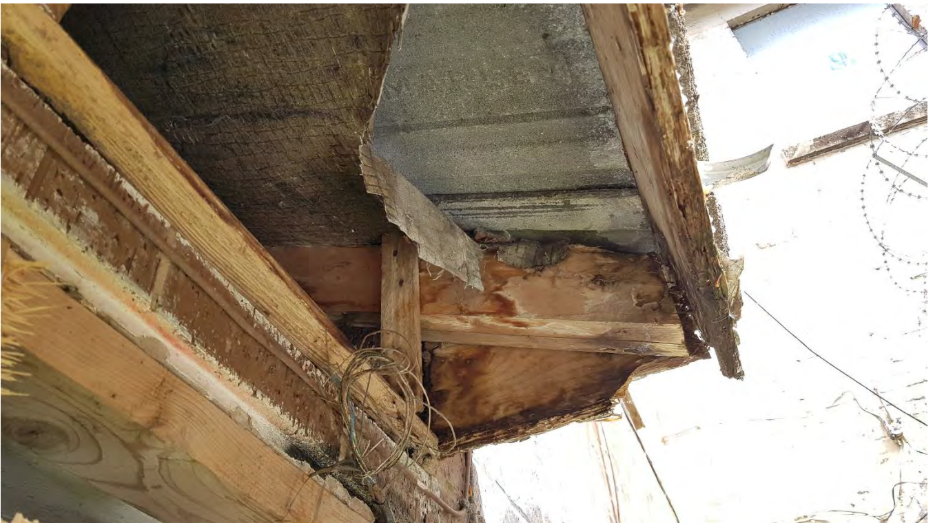
Exposed and water stained timbers to SW extension
