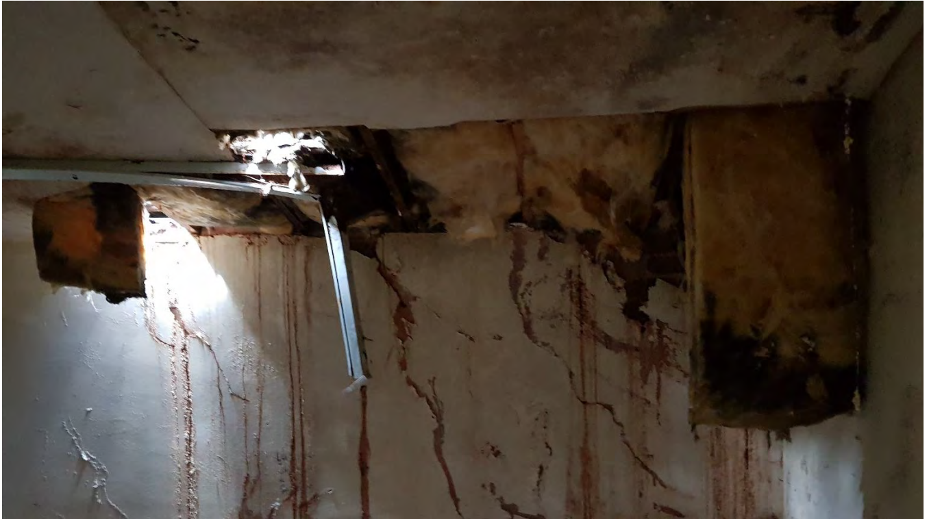
Partially collapsed ceiling and water damage in the two-storey link structure
