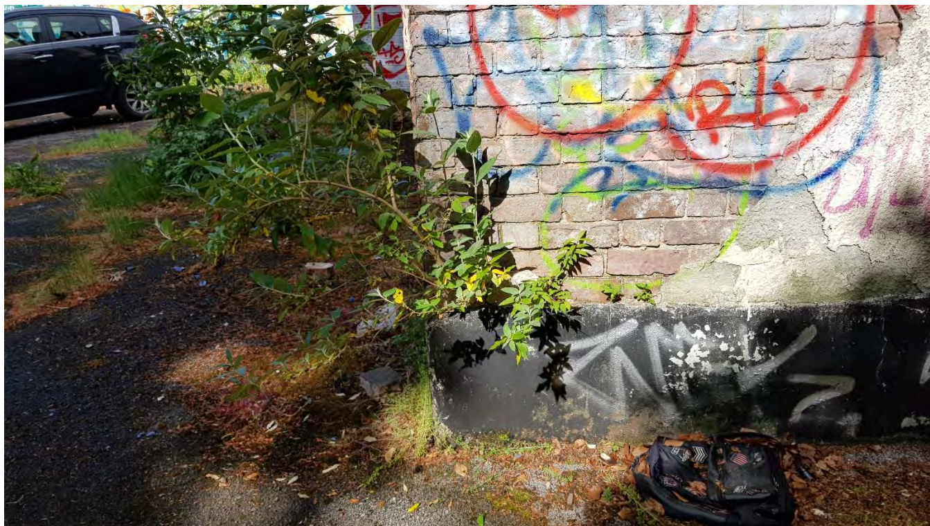
East elevation – vandalism, loose render and vegetation growing out of the wall
