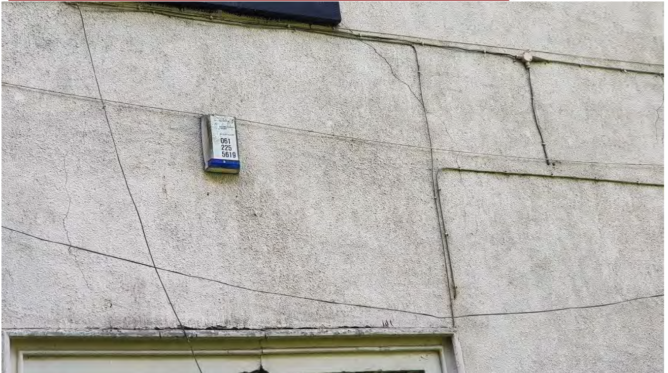
Cracking to render
