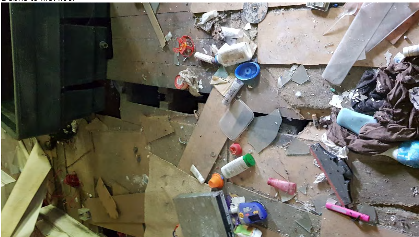
Broken glass and holes through floors prevent better access
