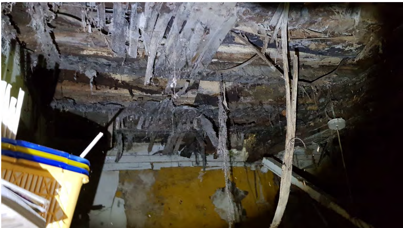
Partially collapsed ceilings. Rotten first floor timbers
