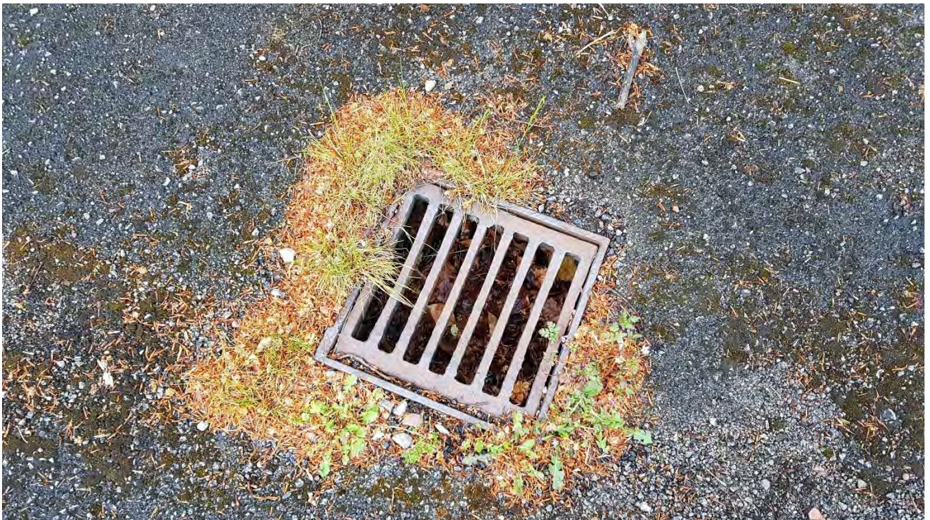
Blocked drains through lack of maintenance. The area around this gully is sunken which could mean further issues with leaking drains.
