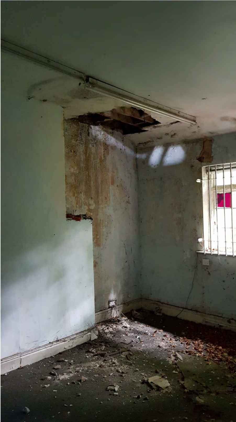
Partially collapsed ceiling above first floor
