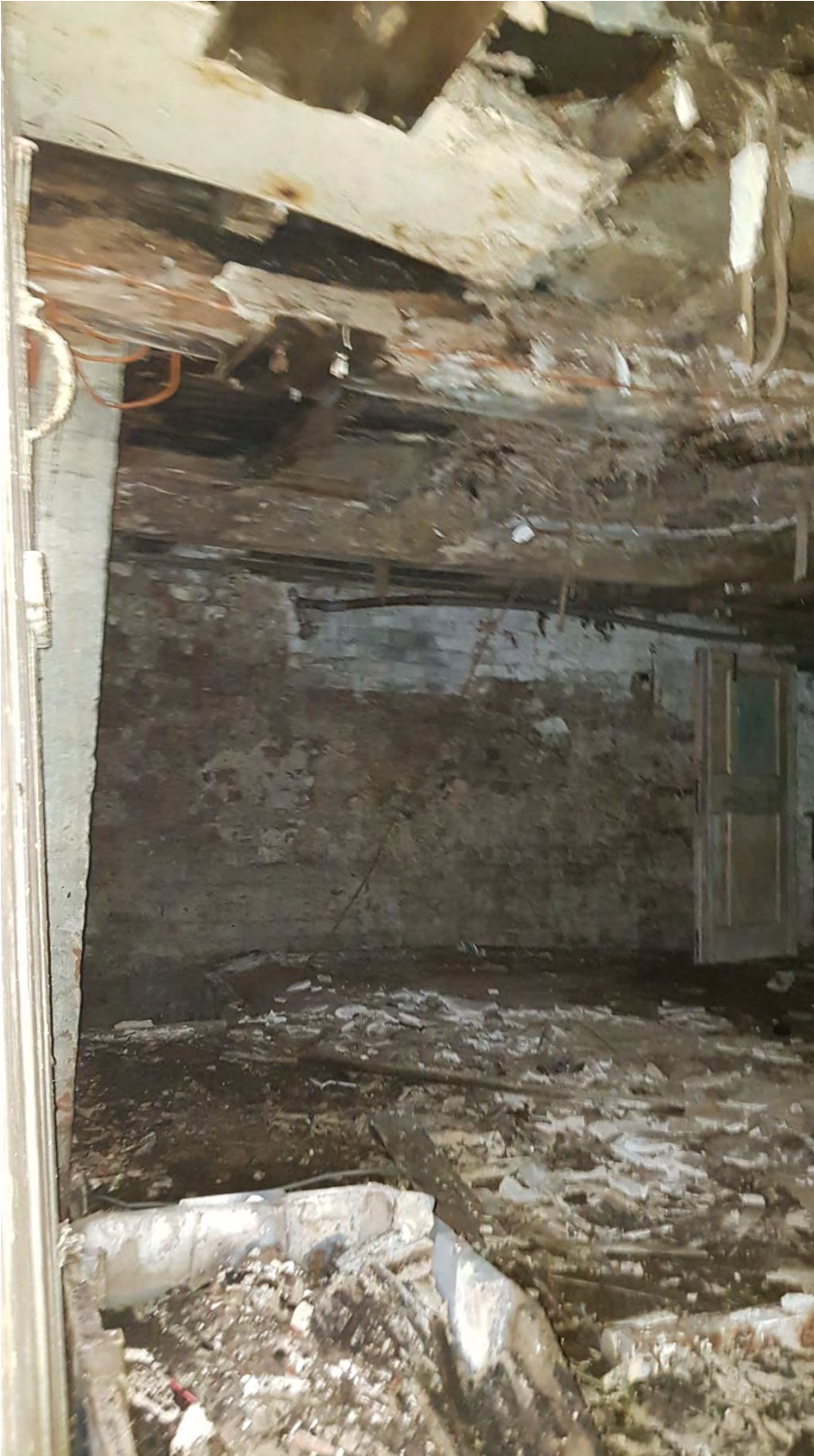
Storage space under ground floor – note rotten timbers and debris
