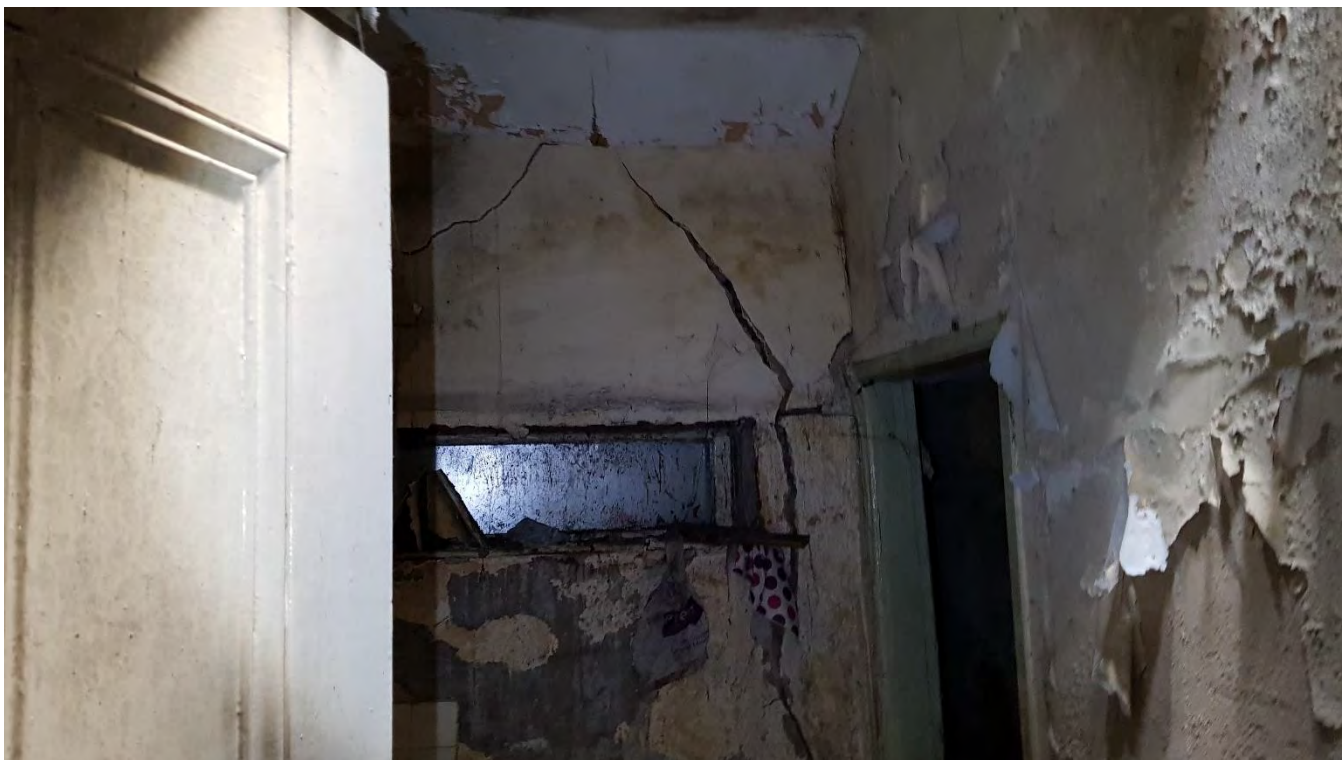
Significant cracking to internal walls
