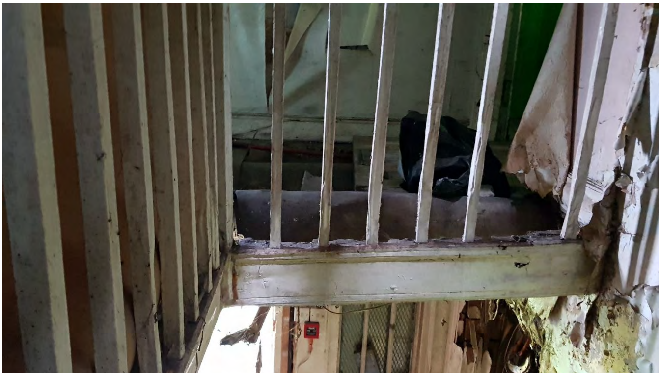
Floorboards missing to first floor
