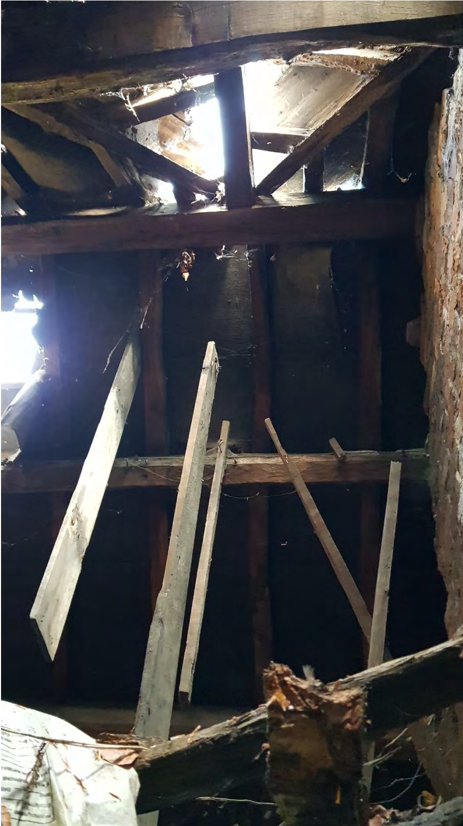
Collapsed roof and ceiling over stair
