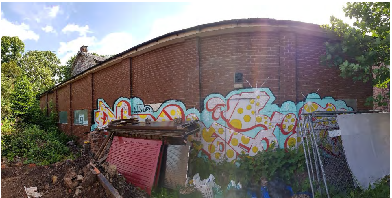
West elevation of single storey extension. Area vandalised and being used to store materials. (Panoramic shot, ignore distortions)
