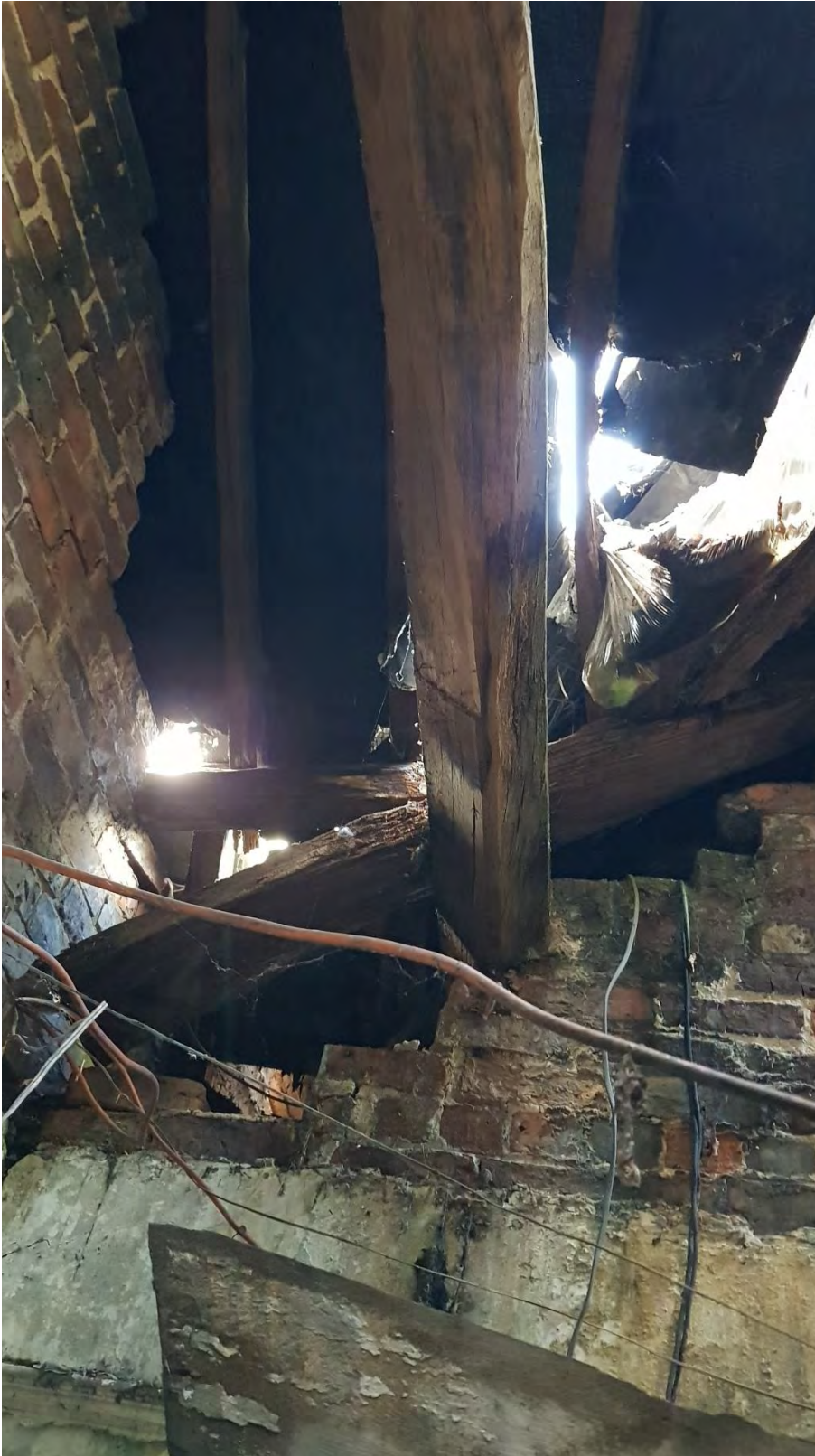
Partial collapse of roof. Purlin support inadequate due to masonry removal
