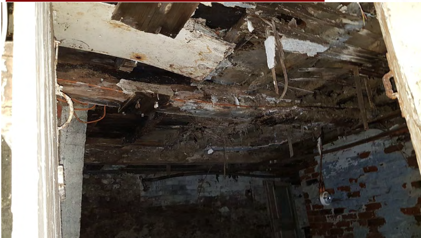
Underside of ground floor – note rotten timbers
