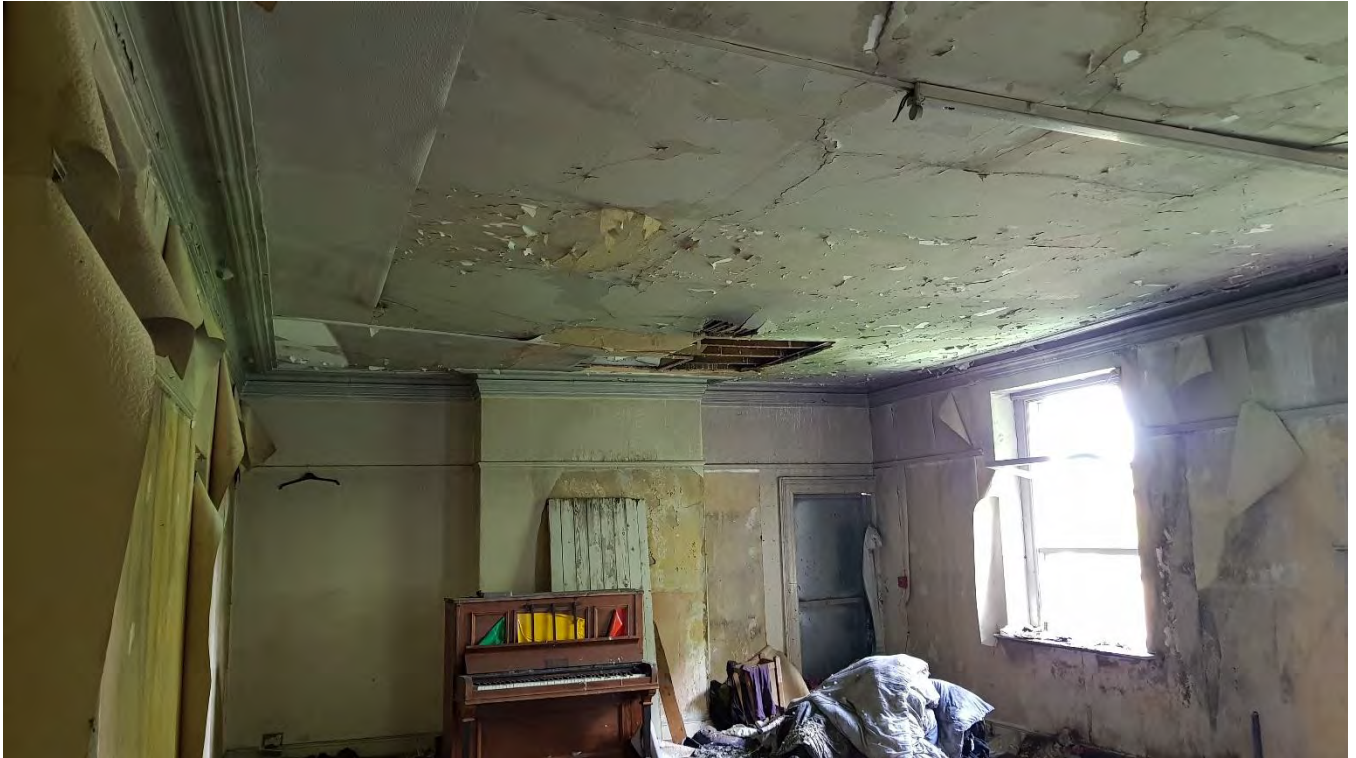
Partial collapsed ceiling in original house (west end of north wing above first floor)
