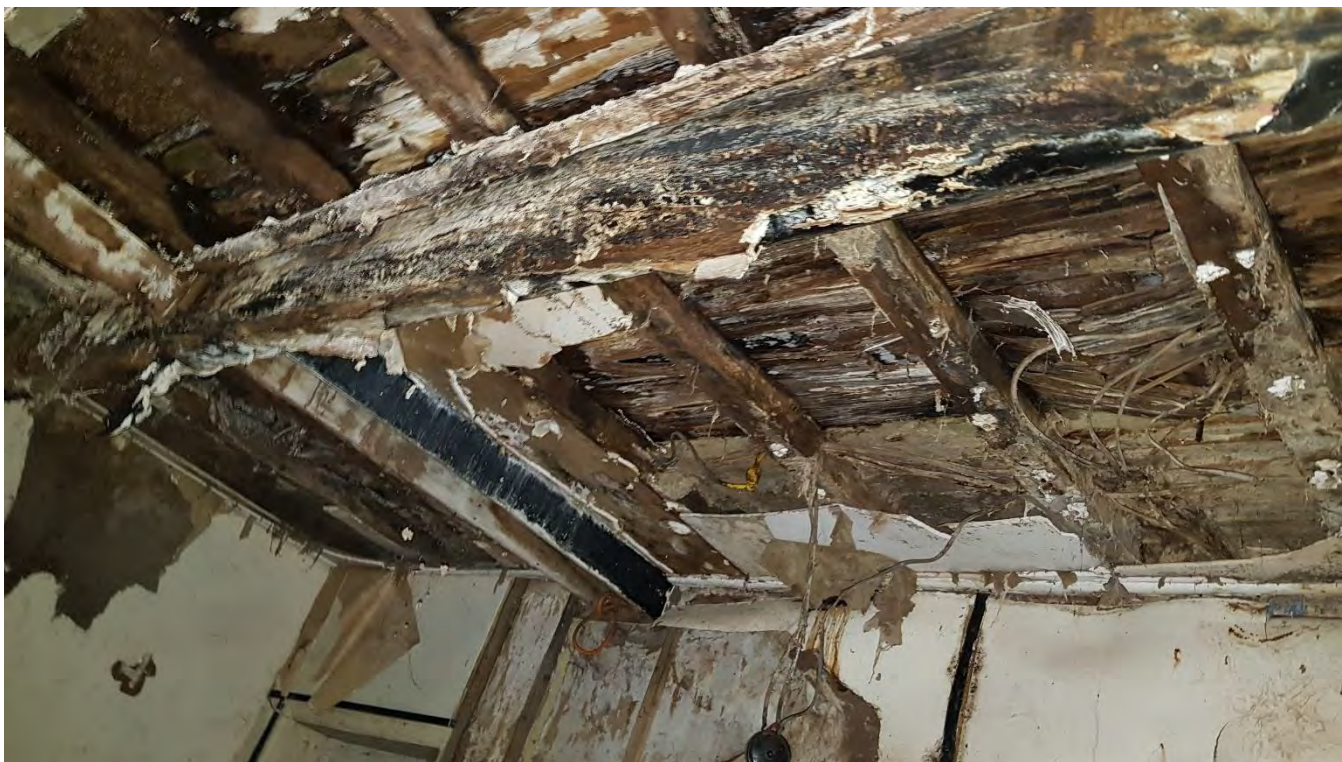
Rotten timbers to underside of ground floor
