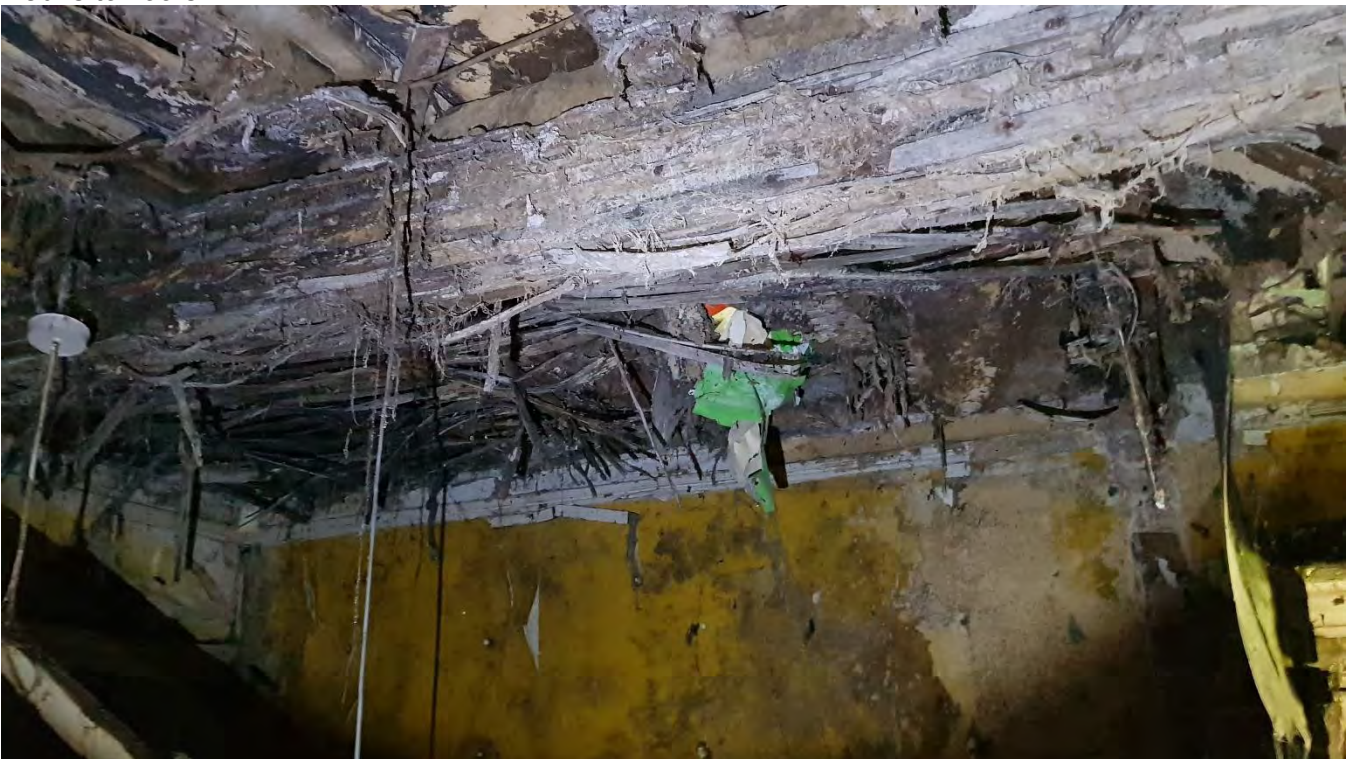
Rotten first floor timbers
