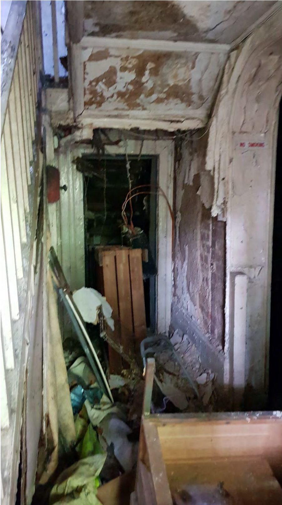
Debris and rubbish scattered throughout
