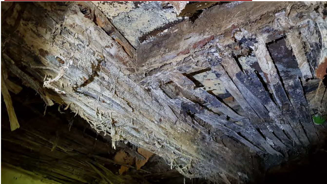
Ceiling over the room in the previous photo. Rotten first floor timbers
