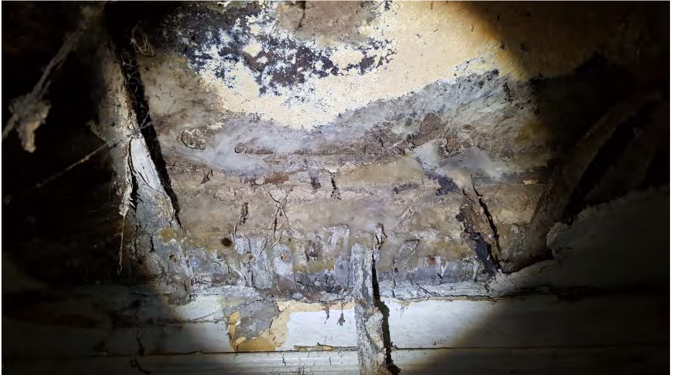
Potential dry/wet rot
