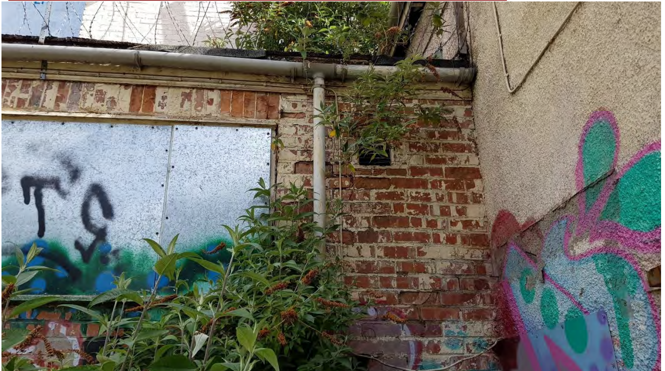
Vegetation growing out of the walls. Spalling masonry where render has been removed (possibly a weak brick that was rendered because of the spalling)
