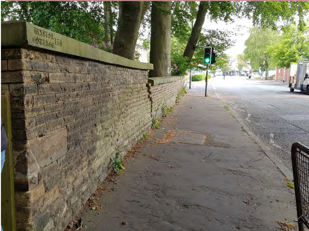
External boundary wall leaning out, damage due to tree growth
