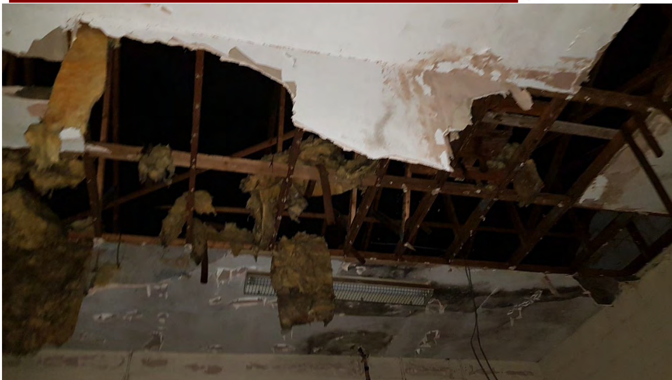
Collapsed ceiling in single storey extension
