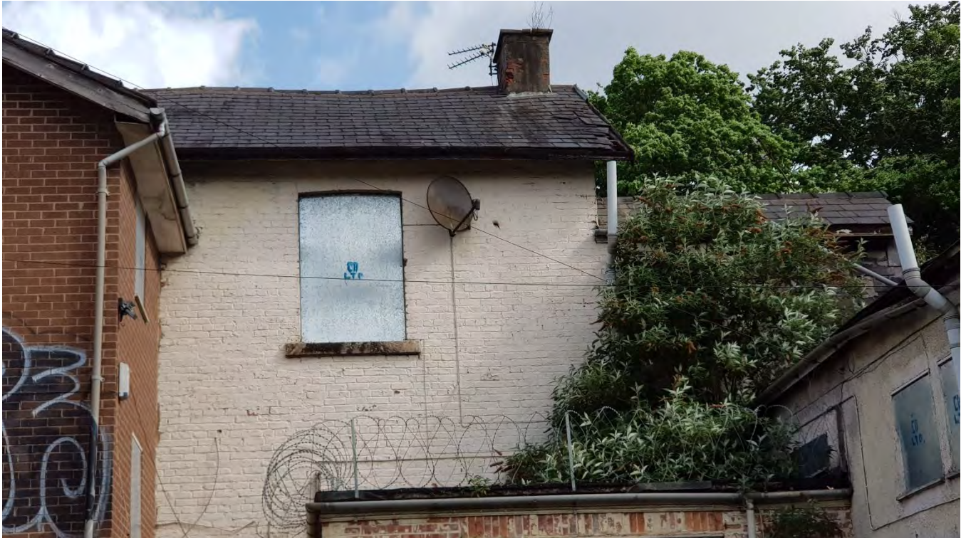
Original roof has settled (partially collapsed in parts). Vegetation growing out of the roof. Chimney in poor state of repair
