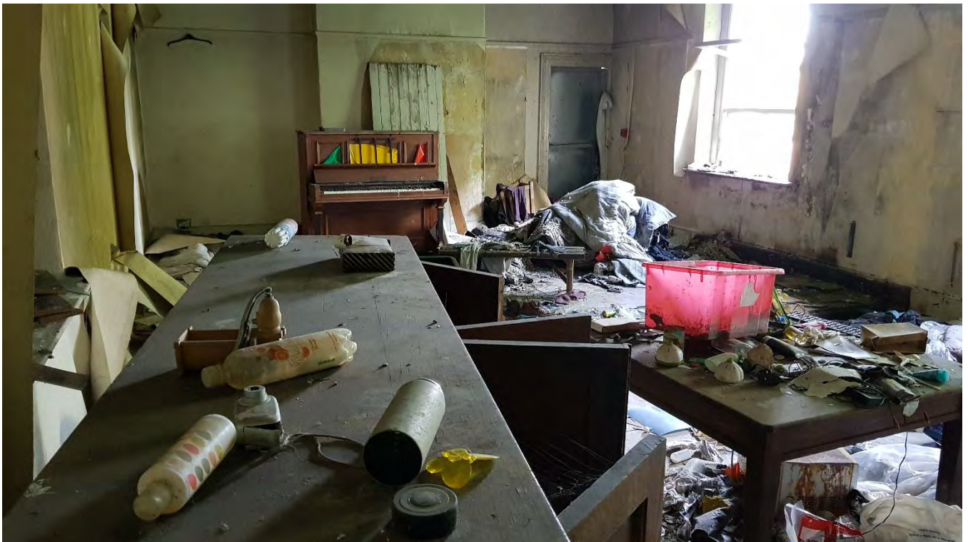
Debris and holes through first floor prevent access
