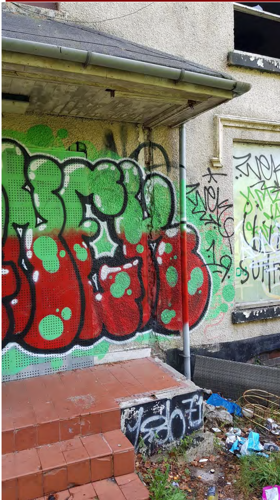
Porch support post missing at north entrance
