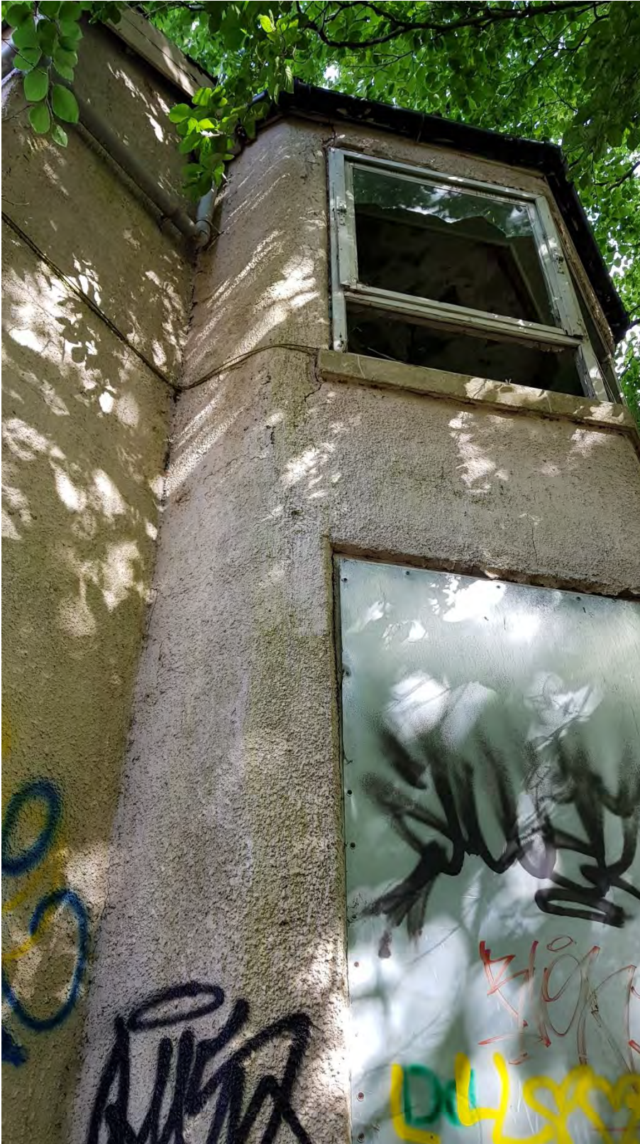
Smashed windows throughout. Minor cracking at the junction of the bay at the main wall. Cracked/ loose render at the corner of the window
