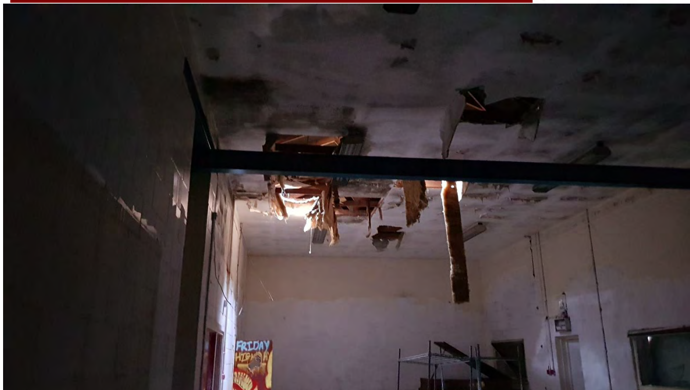
Holes in the ceiling of the single storey extension
