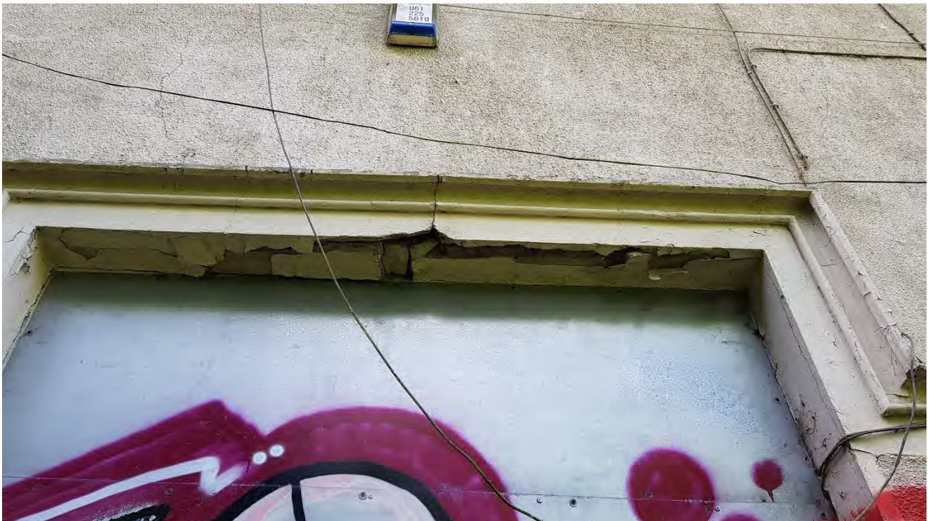
Possible failing lintel to north elevation
