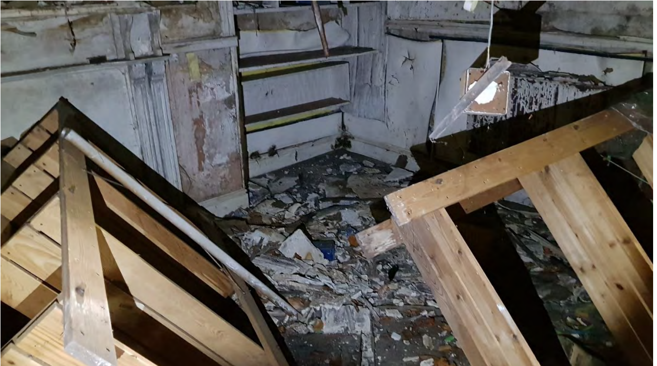
Debris to floors
