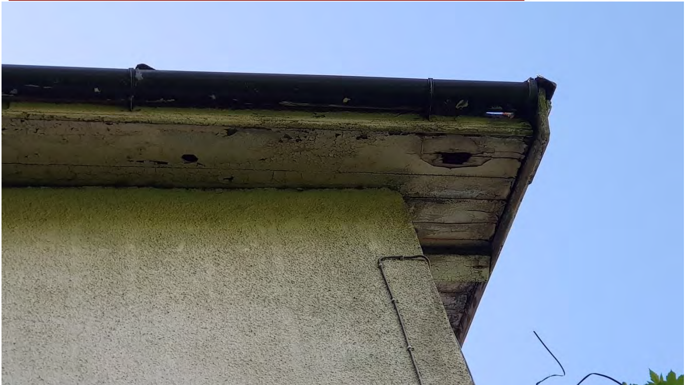
Rotten timbers to roof
