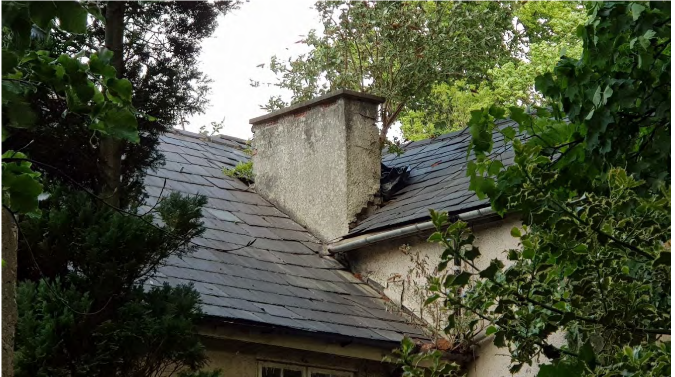
Original roofs in poor condition with numerous holes
