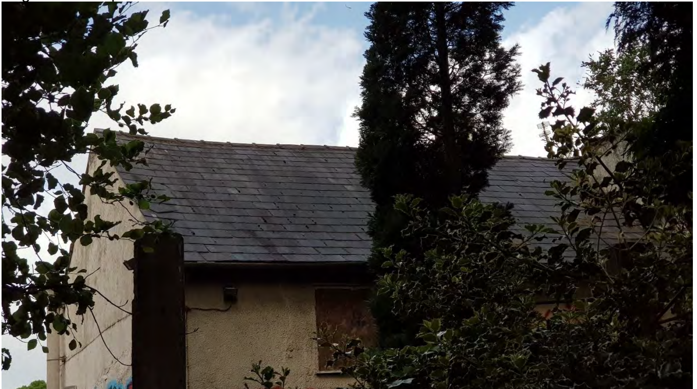
Original roof line distorted where the roof has settled due to rotten timbers, partial collapse
