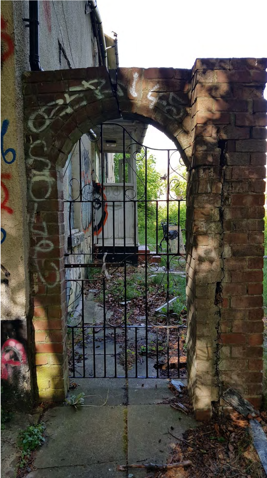
Masonry arched has failed
