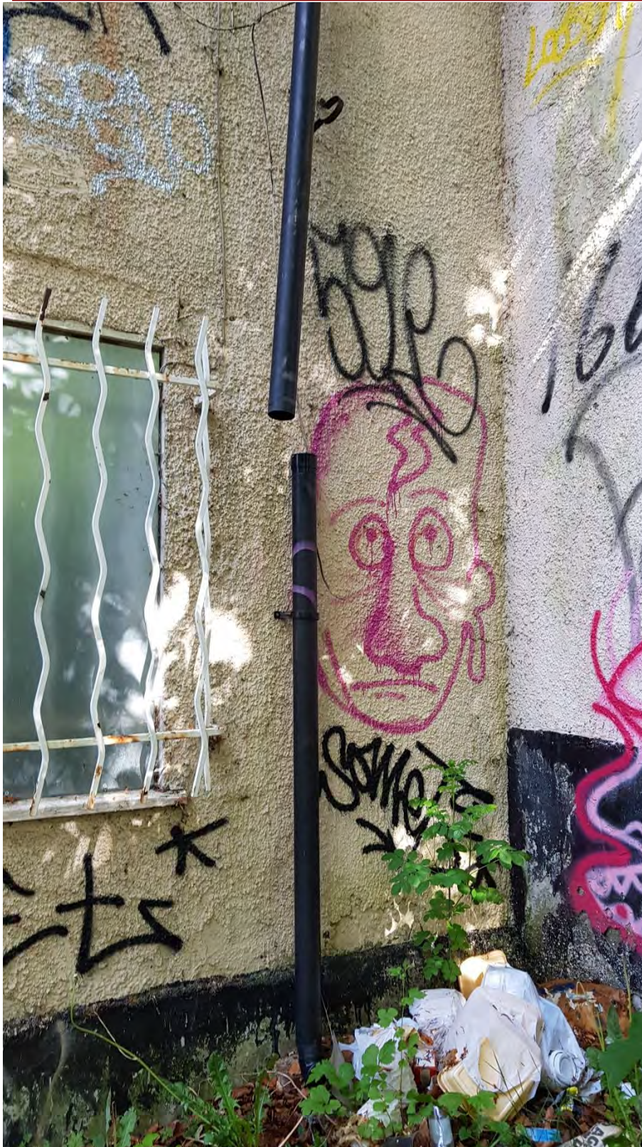
Broken rainwater goods throughout
