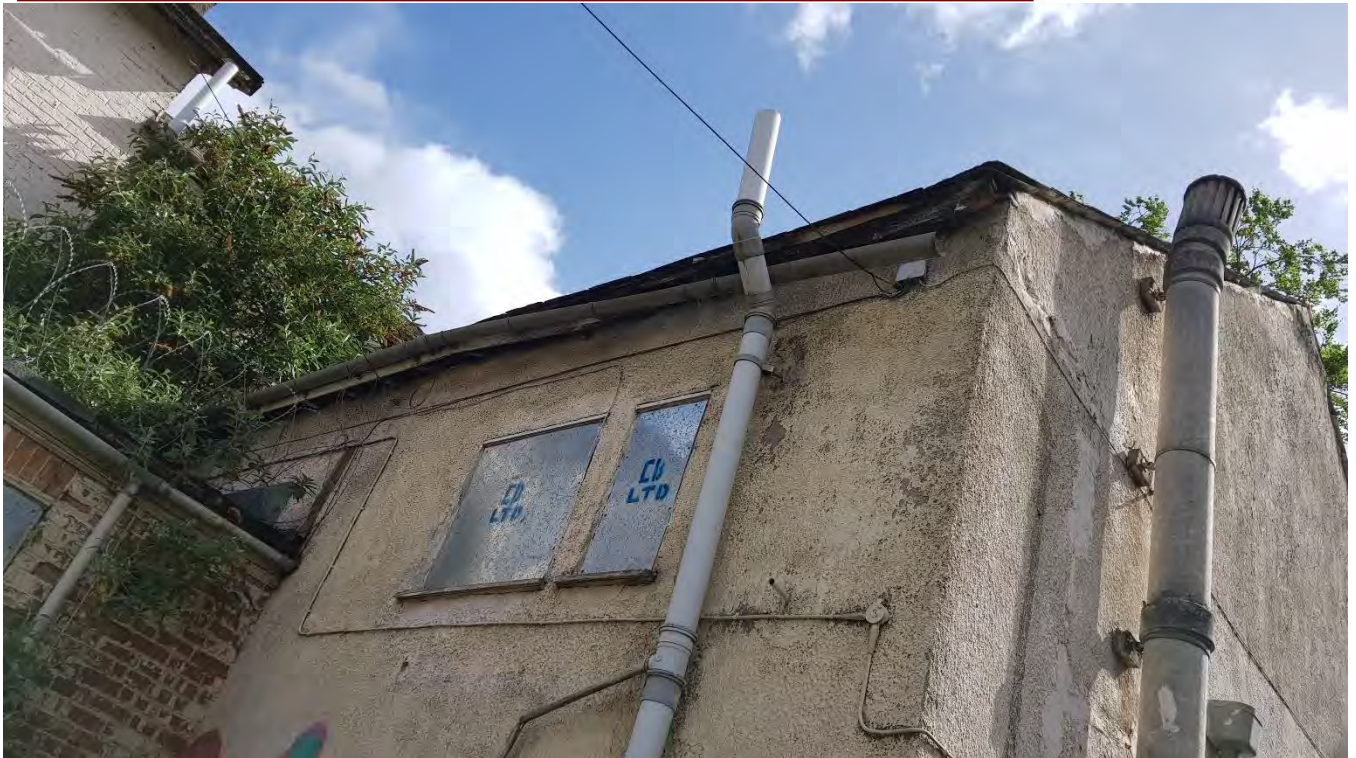
West facing elevation of the south section of the original house. Note vegetation growing out of the roofs
