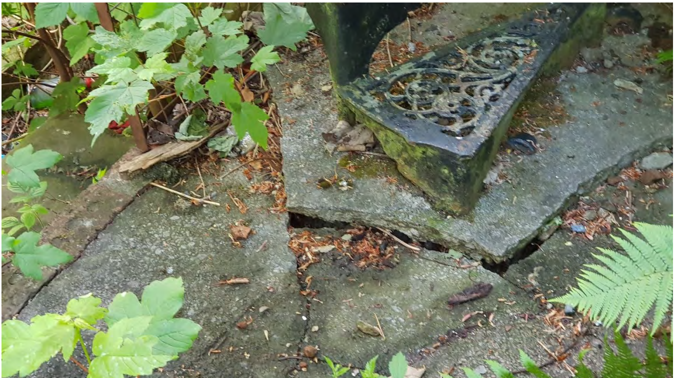
Potential ground movement at rear spiral staircase
