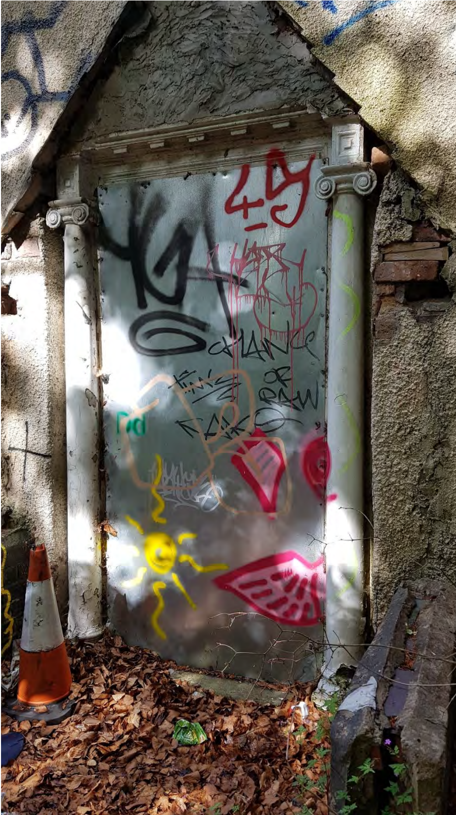
East entrance to original house – vandalised, porch removed, holes through wall
