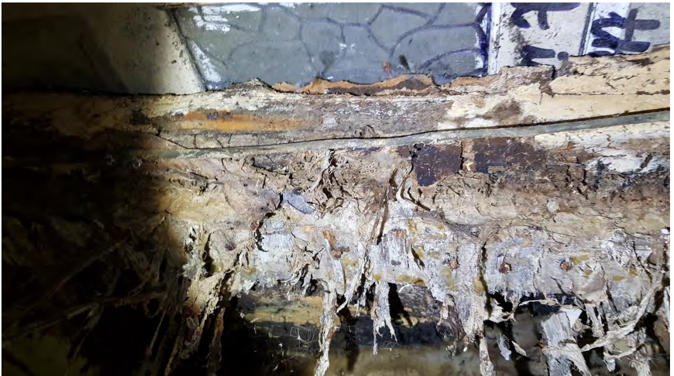
Potential dry/wet rot
