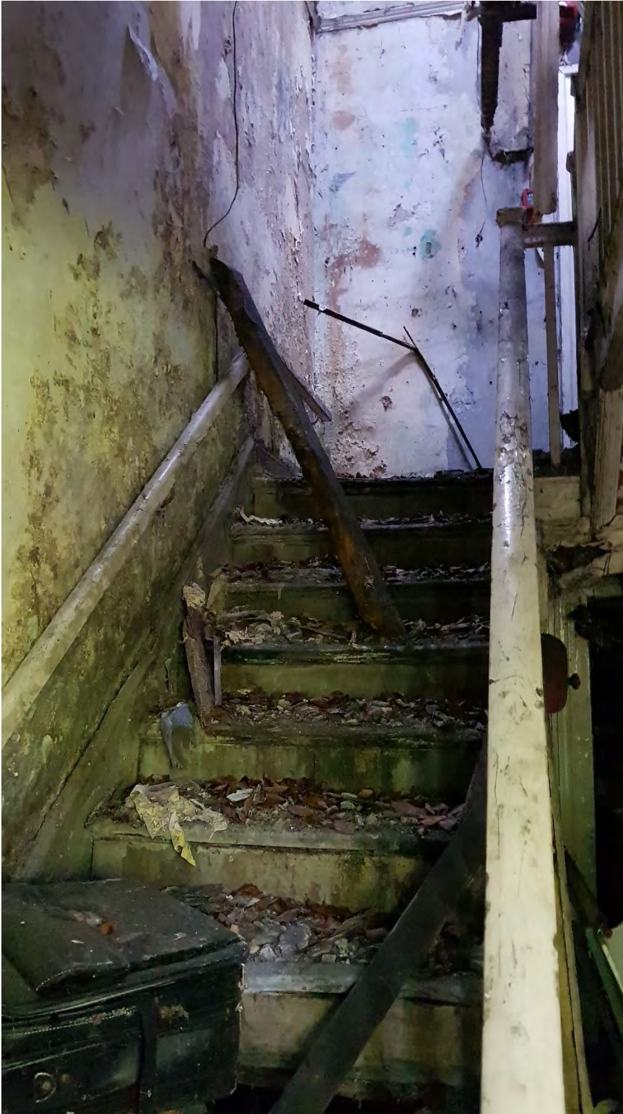
Internal staircase – roof and floor above are partially collapsed. The bottom step and handrail are rotten and no longer connected to anything
