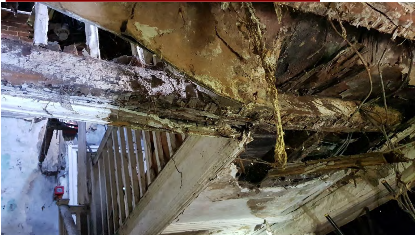
Rotten timbers support stair and landing
