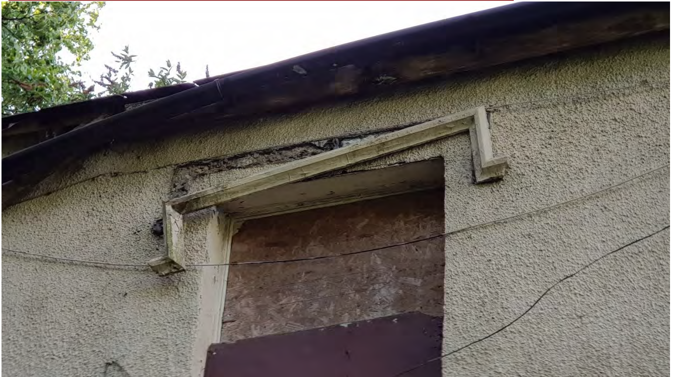
Broken rainwater gutter, rotten timber fascia's, dislodged decorative wall finish
