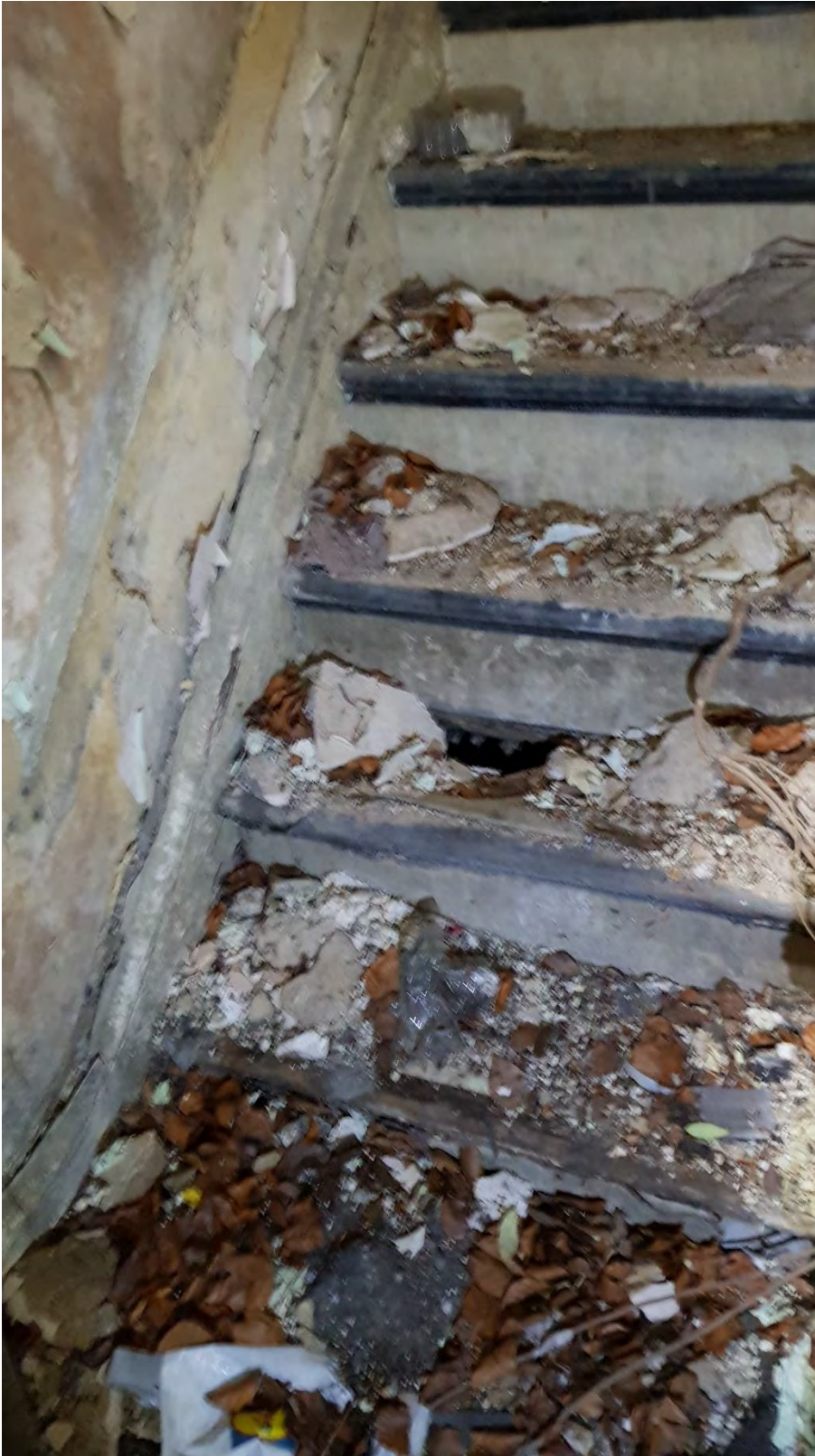
Holes in existing timber stairs (tread partially collapsed) and debris
