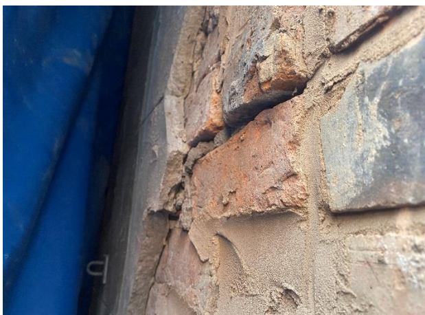
Photo 5: Missing mortar and render on the eastern elevation, covered by PVC sheeting.
