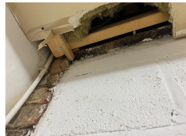
Photo 6: Internal hole in bulk head at south eastern corner.
