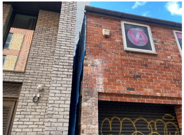
Photo 4: Large piece of PVC sheeting located on the eastern side of the building.
