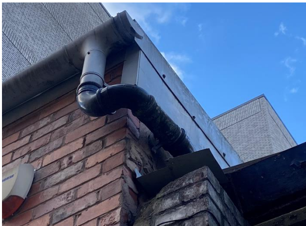
Photo 3: Missing mortar and brick on western corner of the building.
