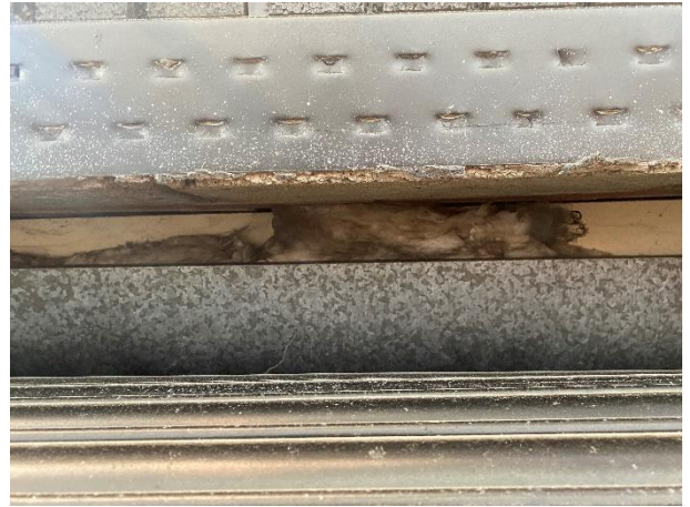
Photo 2: Gap above roller shutter with insulation material visible.
