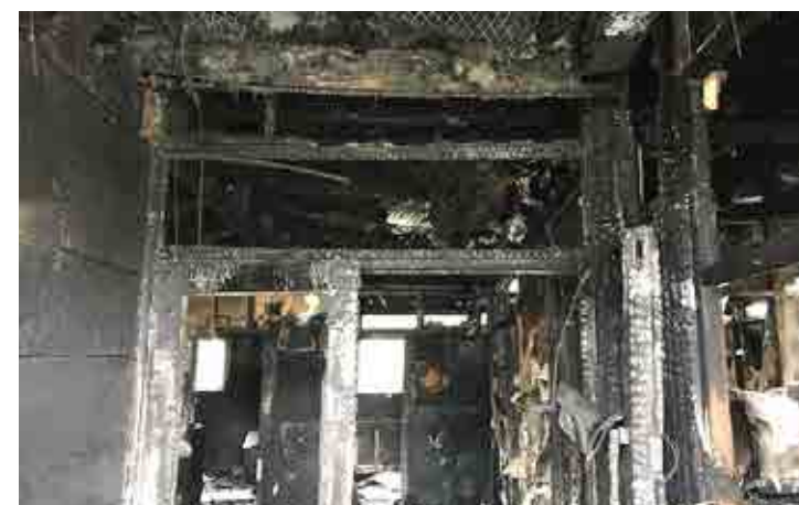
FIRE DAMAGE TO THE FORMER NURSERY
