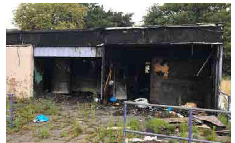
FIRE DAMAGE TO THE FORMER NURSERY
