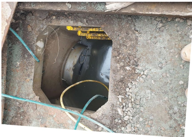
Hydro Brake Chamber
