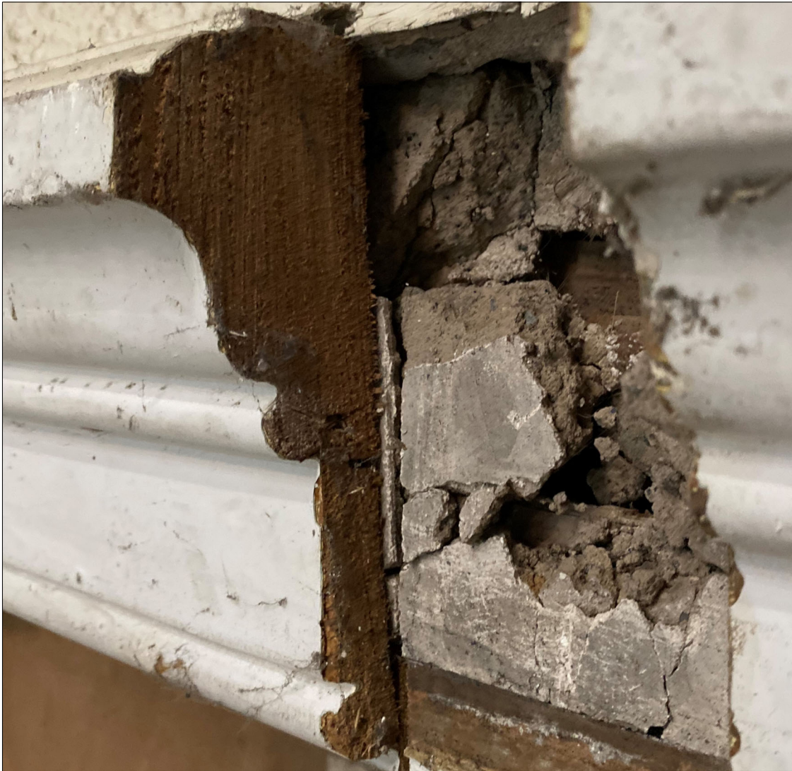
IMAGE OF DAMAGED SECTION OF WINDOW SURROUND SHOWING PROFILE
