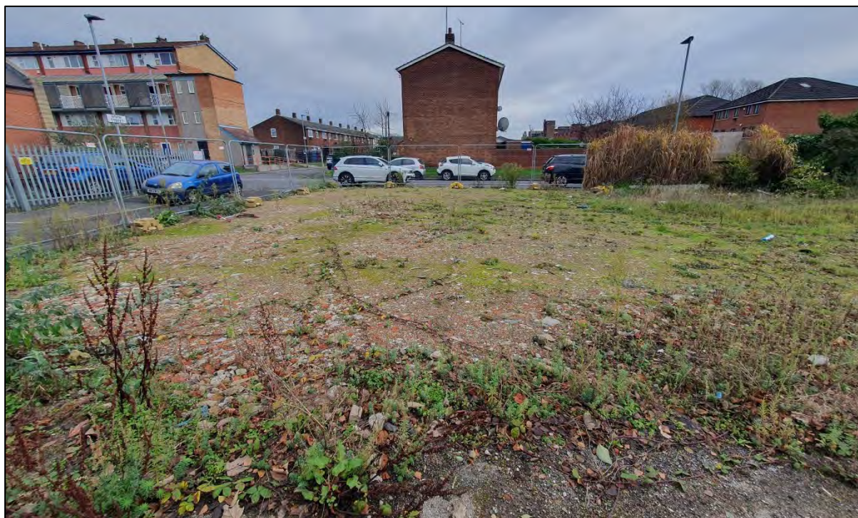
Plate 15 View of demolition rubble covering broadly the footprint of the former Park Inn, looking east to south-east
