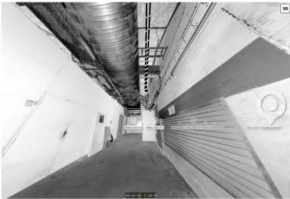
PHOTOGRAPH 02 CLEATED CABLES RUNNING ACROSS ROOF
