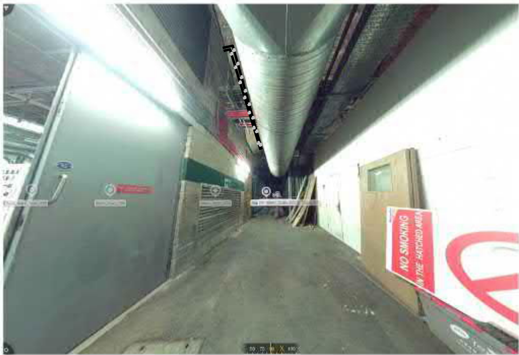
PHOTOGRAPH 01 EXIT FROM PLANTROOM
