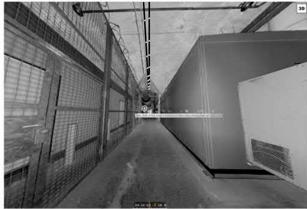
PHOTOGRAPH 04 CLEATED CABLES RUNNING ACROSS ROOF
