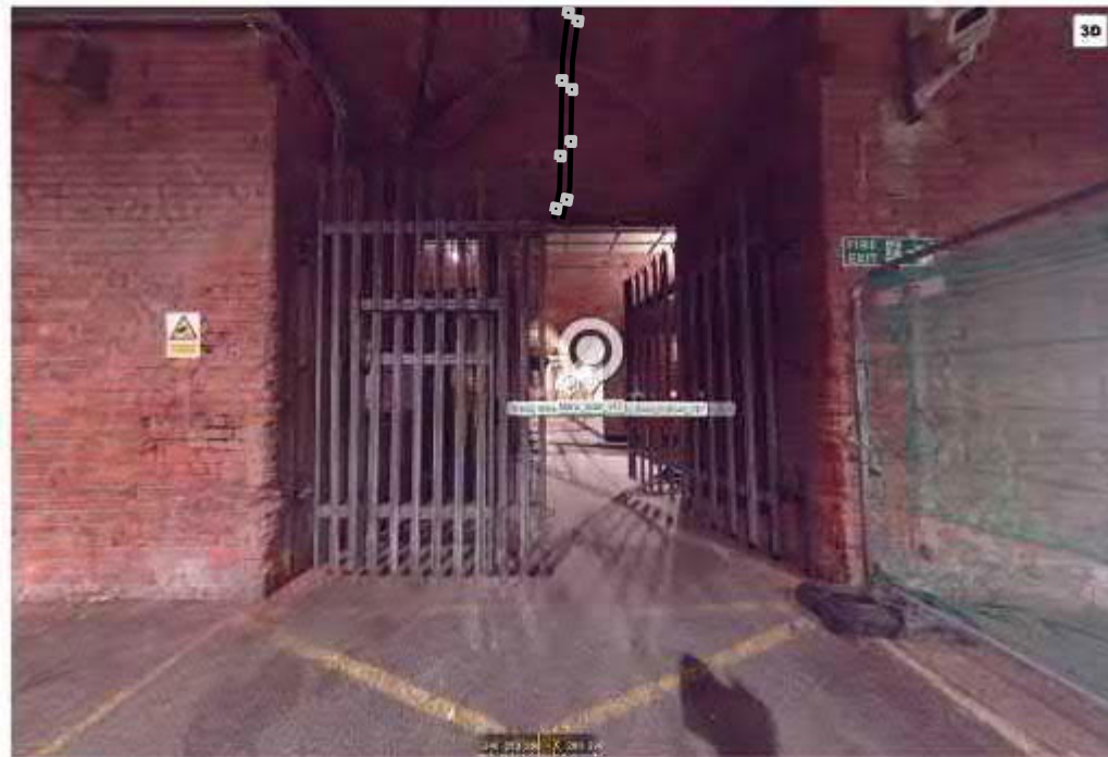
PHOTOGRAPH 06 CLEATED CABLES UNDER GATEWAY ARCH
