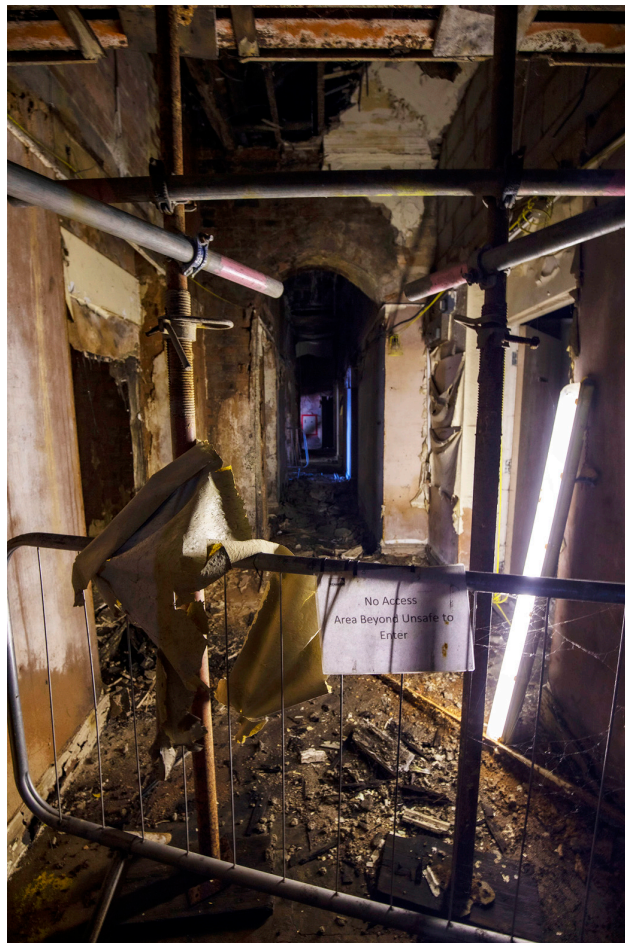
Figure 12 - Inaccessible areas due to risk of collapsing elements (Office wing extension - ground floor)
