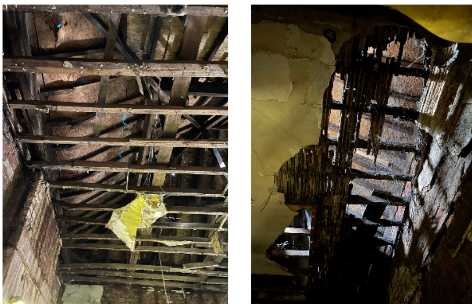
Figure 40 - Advanced state of deterioration of the timber elements of the roof structures
