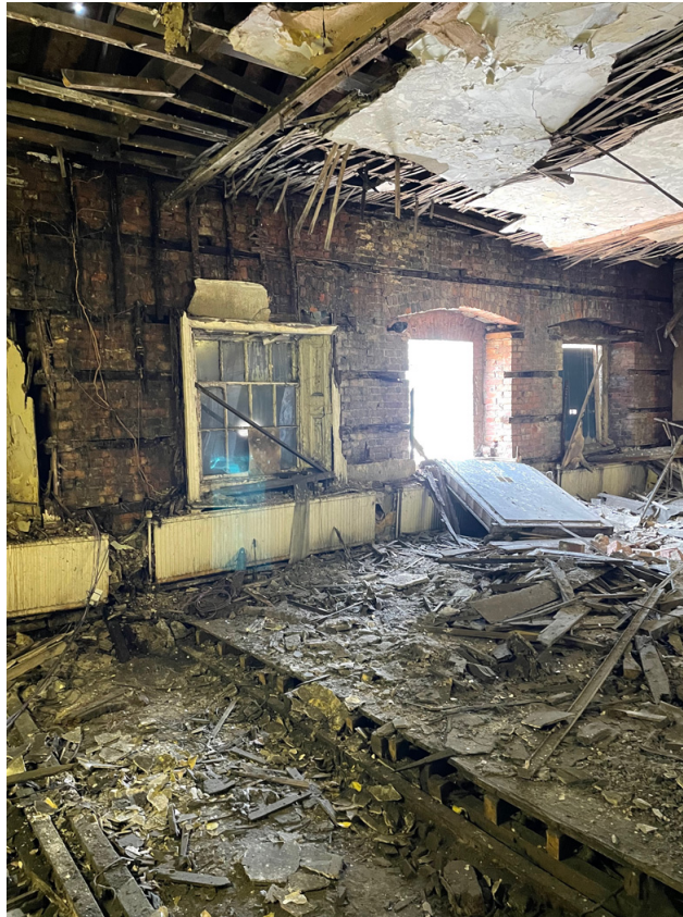
Figure 15 - Collapsed ceiling and windows (office wing extension - first floor)
