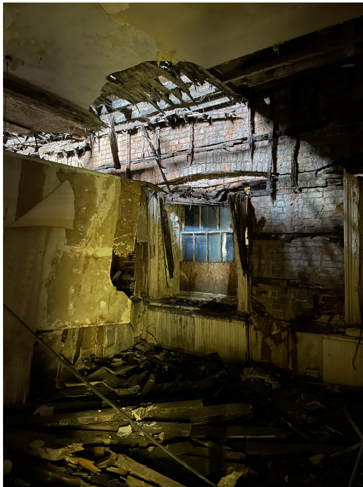
Figure 14 - Completely collapsed ceiling and exposed roof (office wing extension - first floor)
