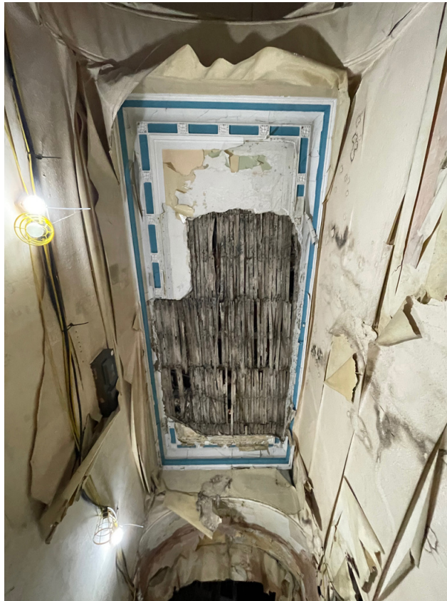
Figure 16 - Partially collapsed ceiling and damaged cornice (late 18 th century former dwelling - ground floor corridor)
