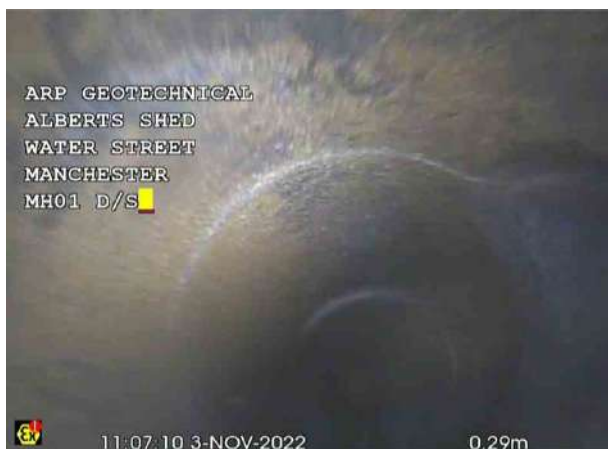
MH01X_6c986c9b-7597-4e10-bd14-b7b09cb2373c_20221103_111732_185.jpg, 00:00:04, 0.29 m Junction at 2 o'clock, 100mm dia
