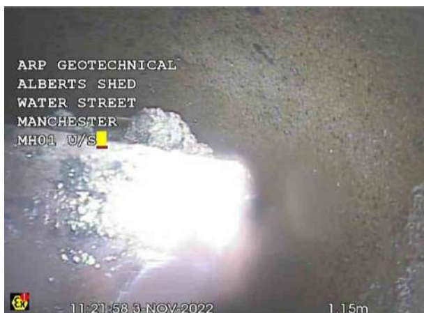
UPSTREAMX_e9b5231e-8ef0-4888-a9ec-0526debadabe_202 21103_113849_327.jpg, 00:00:16, 1.15 m Settled deposits, fine, 80% cross-sectional area loss, BRICK
