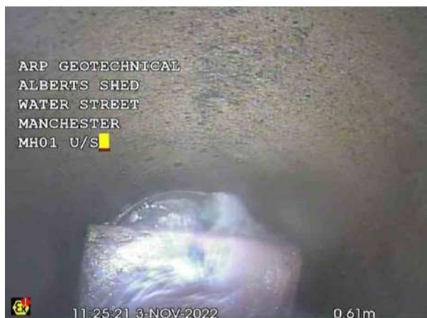
UPSTREAMX_f23bd0f1-b6de-409b-a45d-34eea2a08706_202 21103_114950_325.jpg, 00:00:14, 0.61 m Survey abandoned, DUE TO BRICK IN THE LINE
