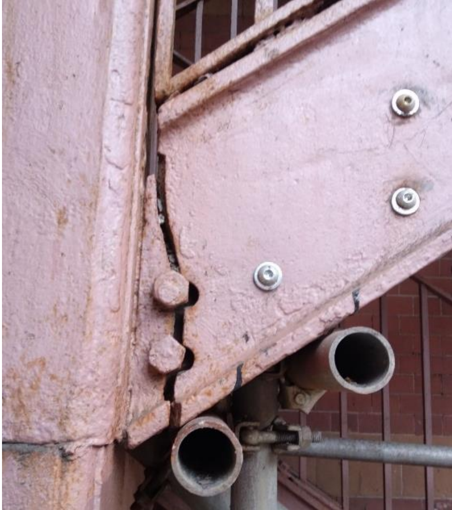
Recent stringer connection failure due to stress in beam.
