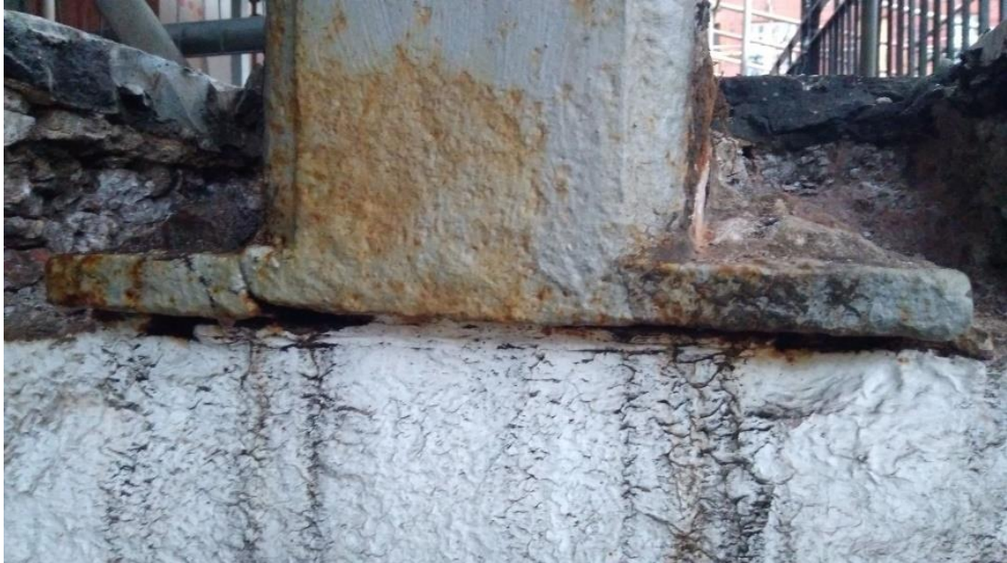
Cast iron column cracked baseplate. Also oversailing side of wall.
