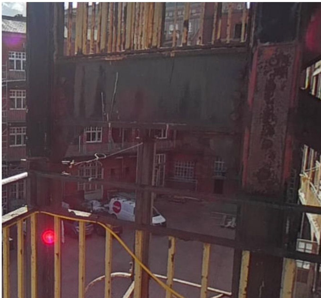
Tension cables added in 20 th century. Ineffective repair. Now removed.
