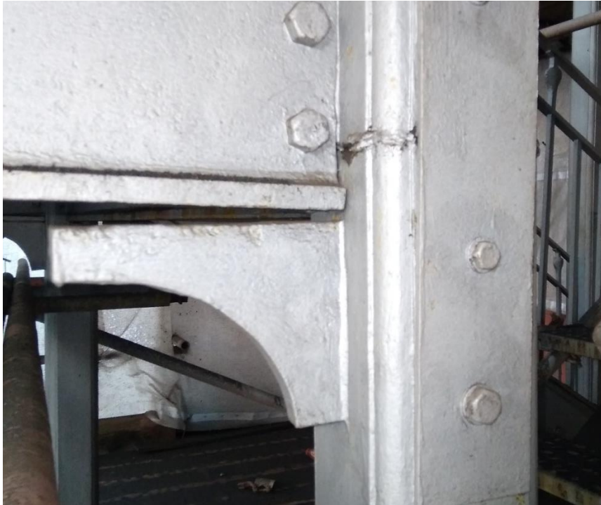
Columns showing welded brackets for supporting landing beams / stair stringers. Ineffective.
