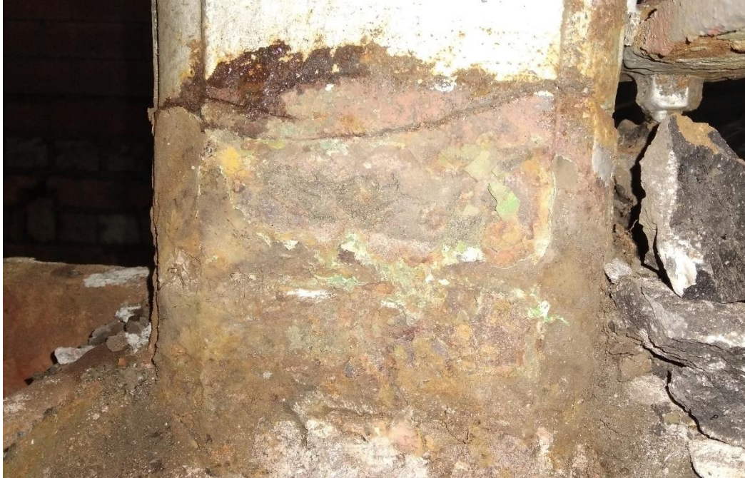
Column cracking (level 2 flat roof)
