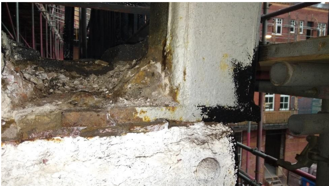
Cast iron column cracked baseplate. Column also oversailing both directions.
