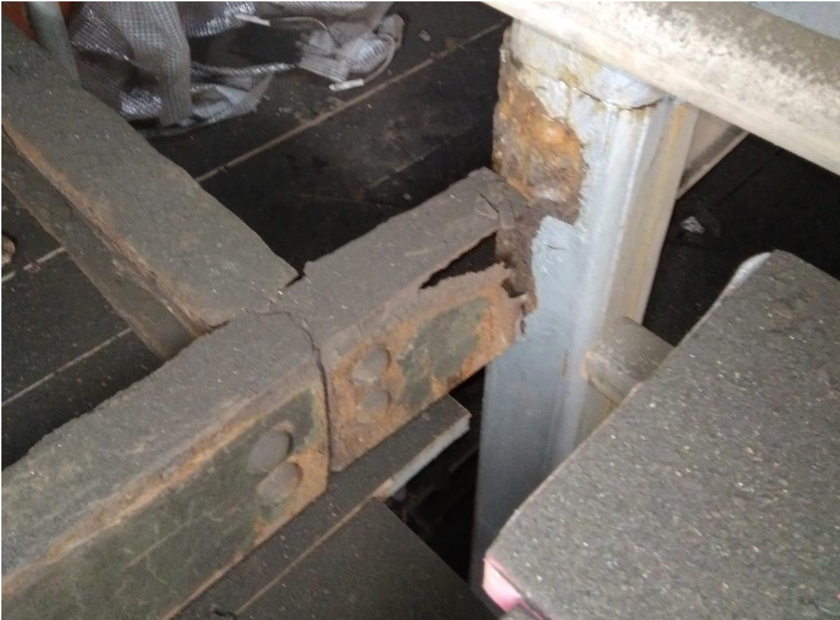
Beam-column corrosion and connection failure.
