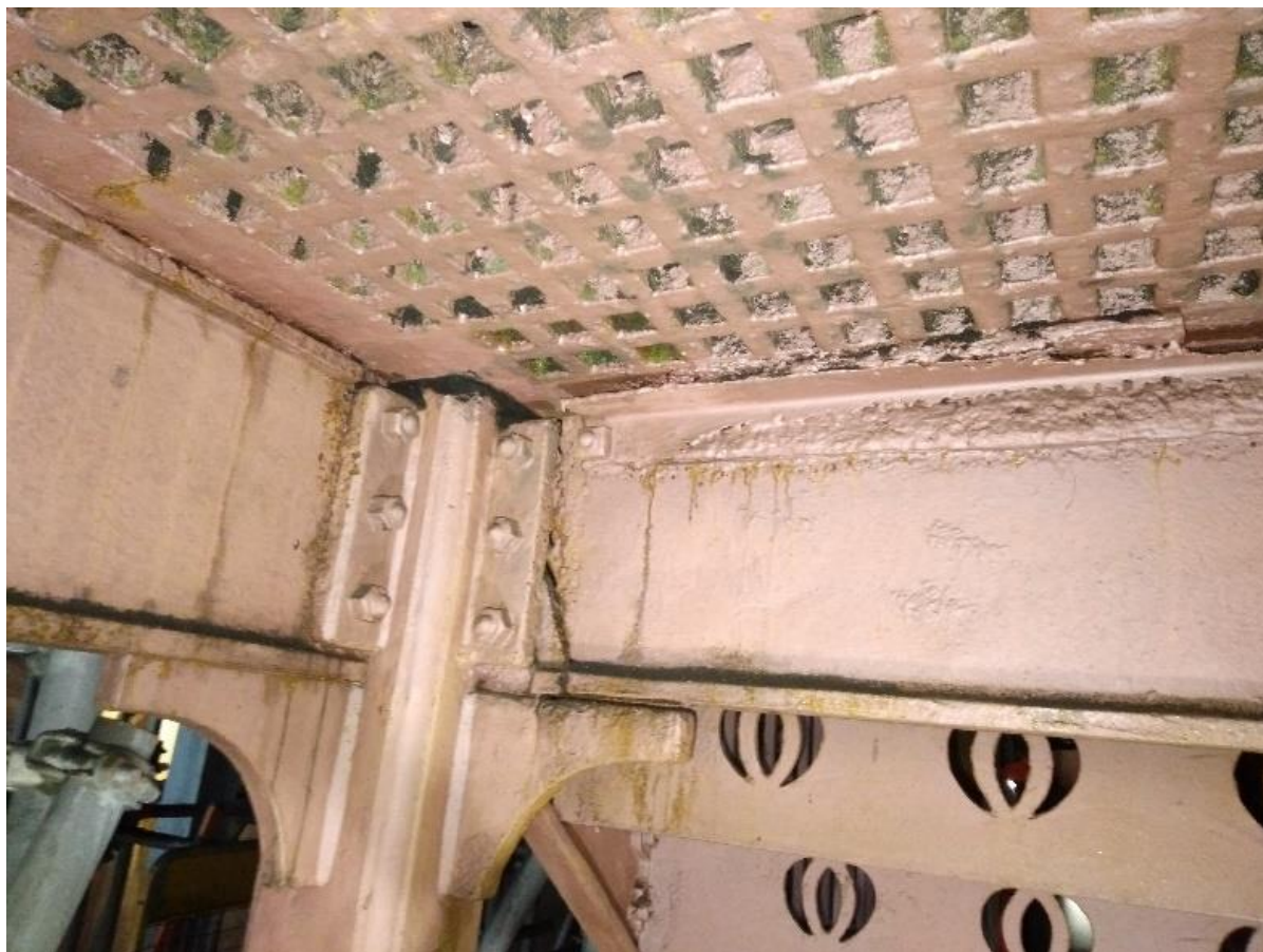
Cracked landing beam at connection.
