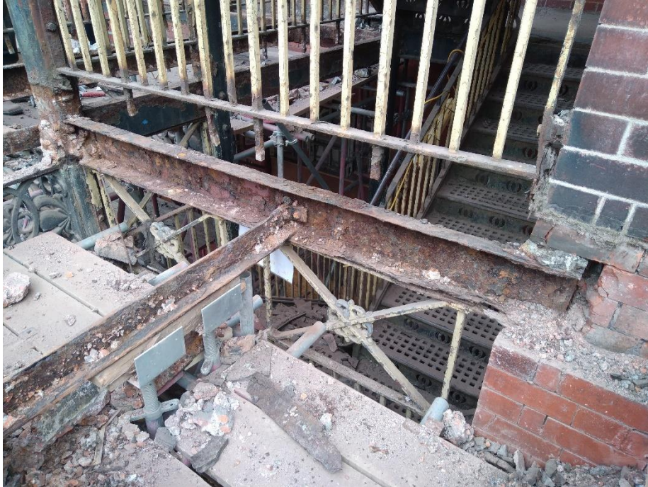
Level 1 showing severely corroded mild steel beam. Replaced as part of Balcony works.
