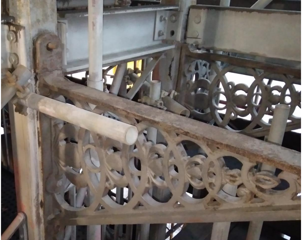
Cracked corbel at bolted connection.
