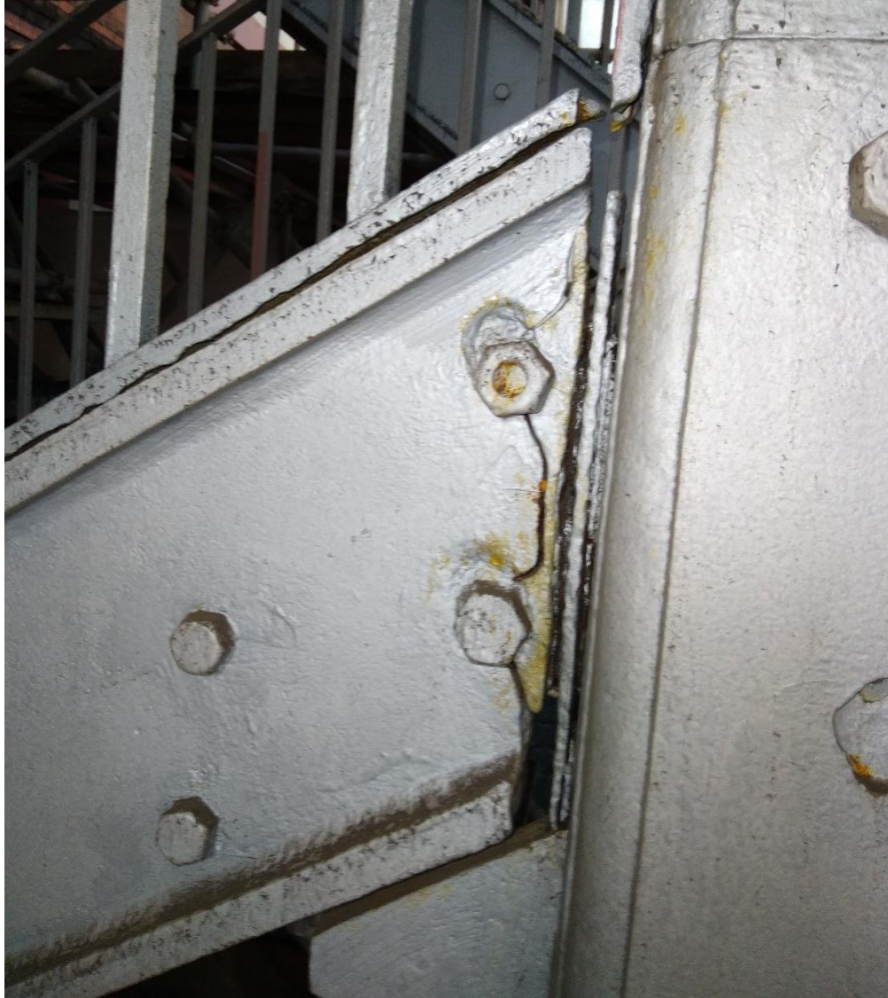
Cracked stringers with what appears historic repairs (bolt replacement).
