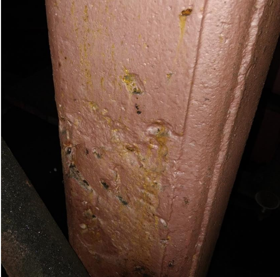
Iron Column corrosion (pitting)
