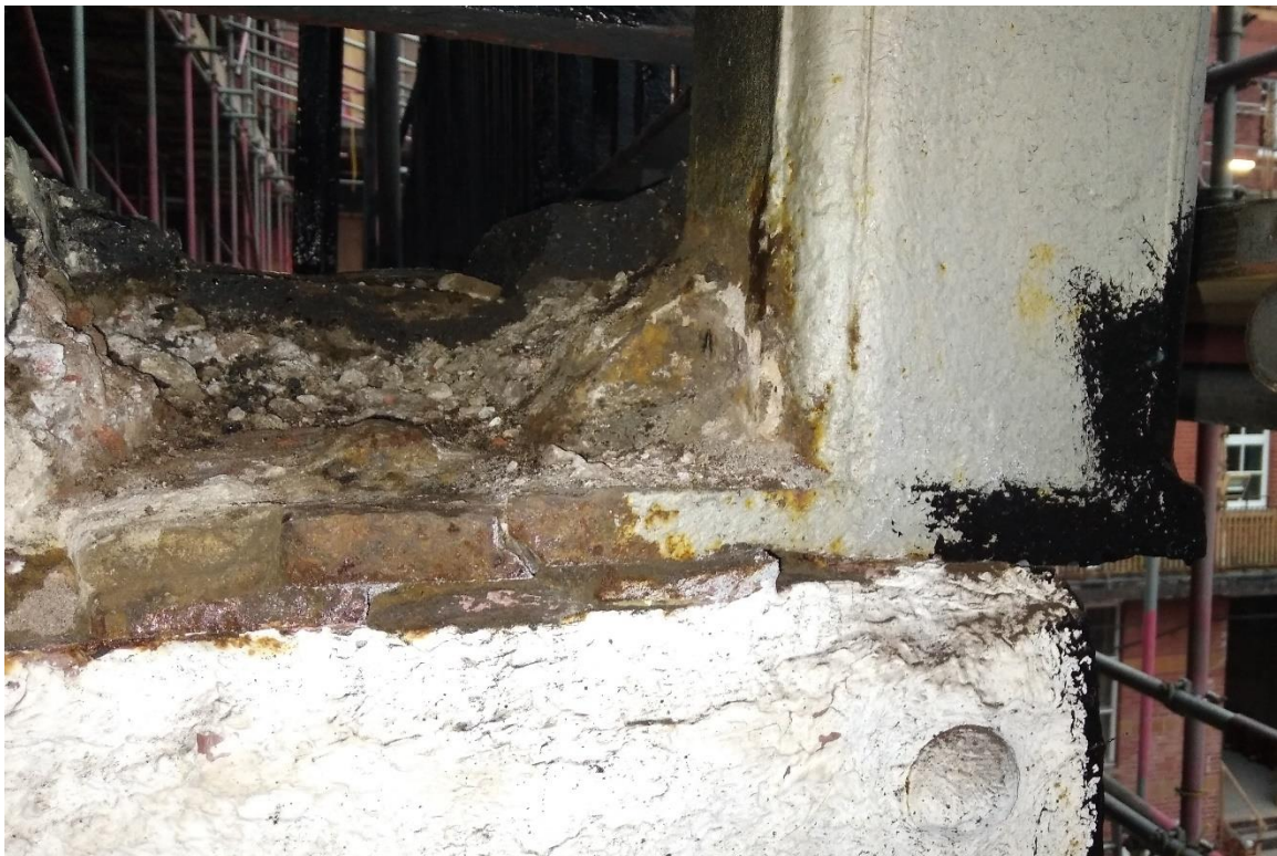
Further historic column cracking encountered to column bases / baseplates at Level 2 flat roof.
