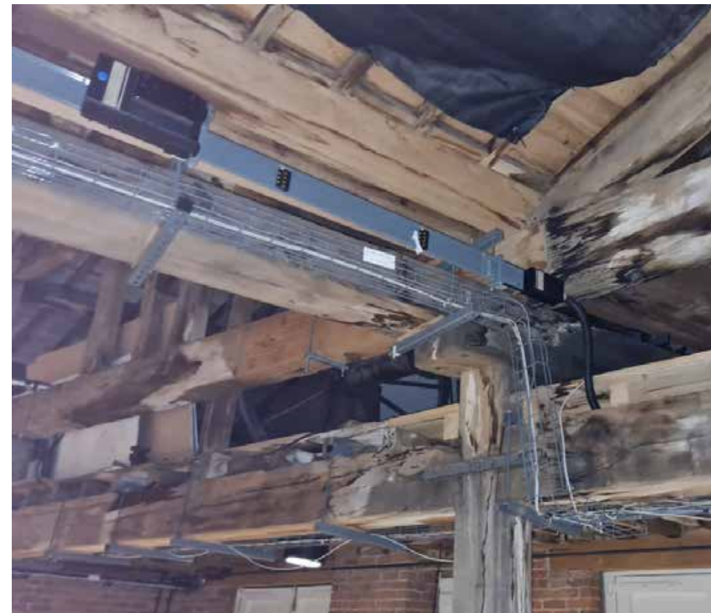
Example of existing services run below roof valley gutters.
