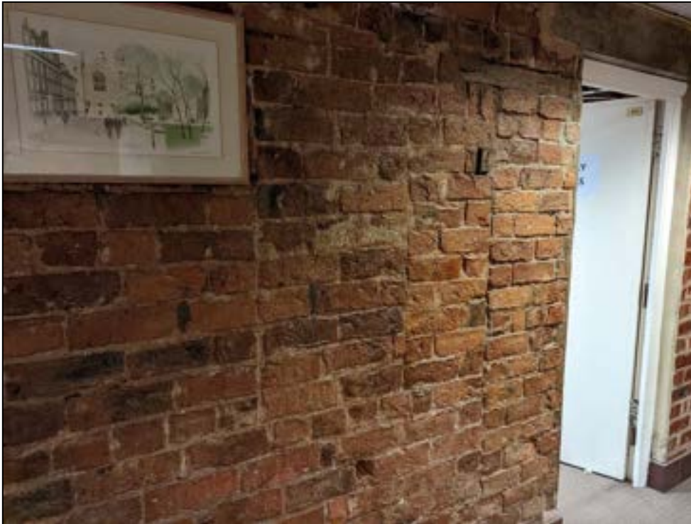
Plate 45: Doorway to be enlarged (item 6) showing possible blocked window and rebuilt wall to the right
