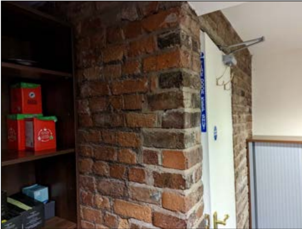
Plate 42: West end of item 4 showing rough joint
