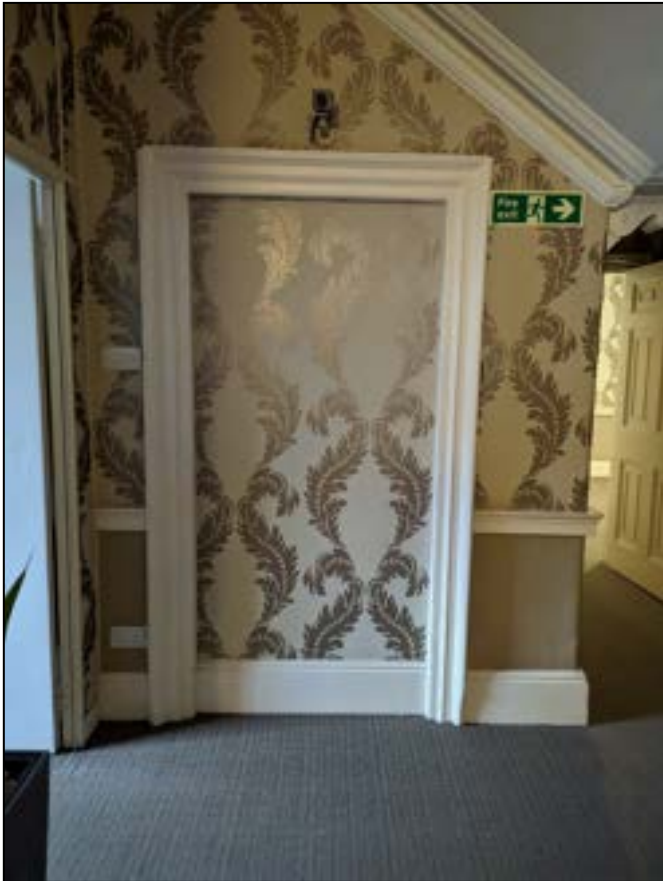
Plate 22: Blocked doorway to room 3 in corridor
