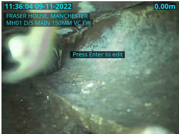
MH 01X_9495520f-13f5-4970-9f07-6edb2390ad7b_20221126_10 5153_408.jpg, 00:00:05, 0.01 m Broken pipe from 2 o'clock to 6 o'clock
