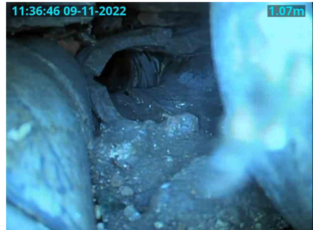
MH 01X_801bd1fc-71e2-480f-a4d8-c5f6b2f04110_20221126_105 307_415.jpg, 00:00:47, 1.07 m Broken pipe from 12 o'clock to 12 o'clock
