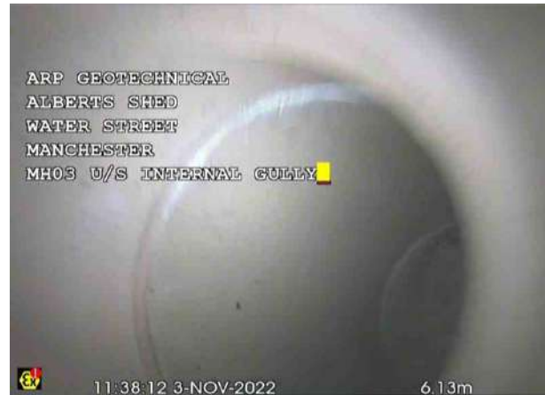
INT GULLYX_3ca9e406-385c-4cb3-aac4-e32f2ab4b197_20221103_111020_695.jpg, 00:00:20, 6.13 m Line deviates right
