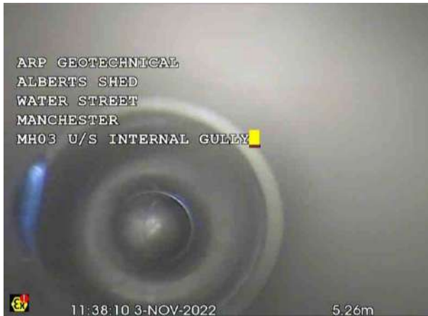
INT GULLYX_62ca5182-b463-47c2-afca-743c1606bd9a_20221103_111008_920.jpg, 00:00:18, 5.62 m Sealing ring intruding from 8 o'clock to 10 o'clock
