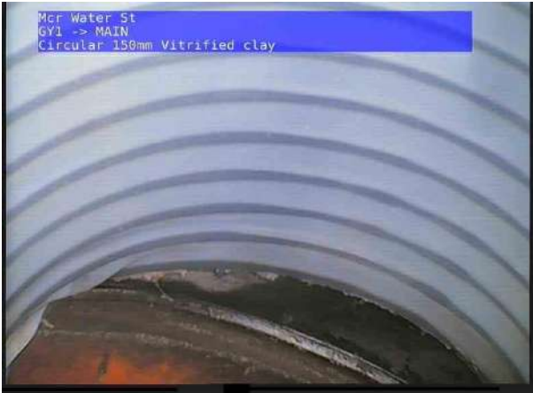
GY1X_d305ec1e-7a58-4598-add2-ba499467c92f_20221005_203459_956.jpg, 00:00:06, 0.24 m Pipe material changes to polyvinyl chloride at this point
