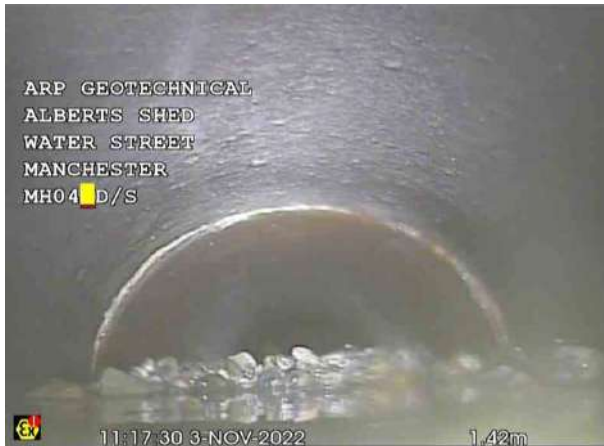
MH04X_aedf9866-95a1-47ce-85b5-e0ea0ae17a03_20221103_113512_208.jpg, 00:00:22, 1.42 m Settled deposits, fine, 50% cross-sectional area loss
