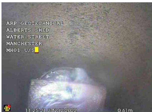
UPSTREAMX_bbbd1632-55f8-432d-908a-931082e5bfa0_202 21103_114936_236.jpg, 00:00:14, 0.61 m Settled deposits, fine, 80% cross-sectional area loss, BRICK
