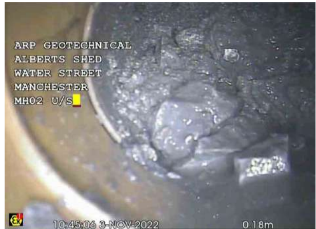
PIPE AX_fd4dab9d-f328-4d40-8b53-bb00776ffb41_20221103_115656_375.jpg, 00:00:17, 0.18 m Survey abandoned, DUE TO SILT
