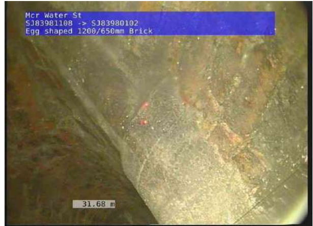
SJ83981108X_ecb20e68-b8b5-4a7c-8daf-c439e93fb031_202 21005_195602_766.jpg, 00:05:28, 31.52 m Other obstacles, protruding through wall from 1 o'clock to 5 o'clock, 30% cross-sectional area loss
