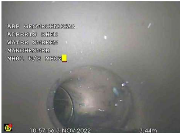
MH02X_5649f3a6-fc35-4340-aa58-f5dd11ebddb5_20221103_115149_741.jpg, 00:00:12, 3.44 m Line deviates left
