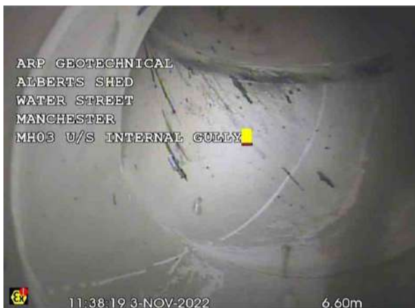
INT GULLYX_b44b2059-3500-4da4-b404-f4379f5f0aee_20221103_111043_704.jpg, 00:00:27, 6.60 m Finish node, other special chamber, reference: INT GULLY, INTERNAL GULLY
