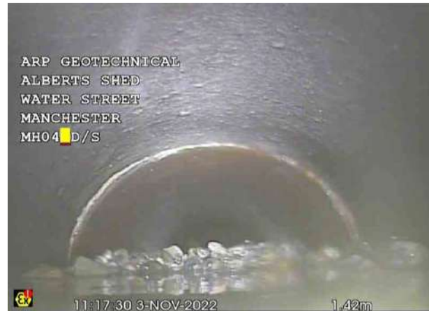
MH04X_86c1a2af-402a-432c-99a1-a51d12199534_20221103_113525_263.jpg, 00:00:22, 1.42 m Survey abandoned, DUE TO SILT AND DEBRIS
