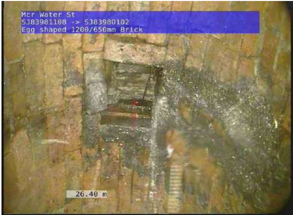
SJ83981108X_2d31f6c7-d1ba-4647-a7ba-8a75d3cb57f2_202 21005_195425_046.jpg, 00:04:05, 26.40 m Connection other than junction at 12 o'clock, 225mm dia
