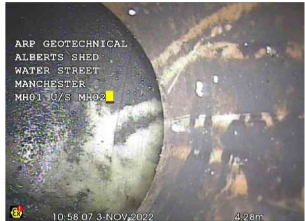
MH02X_0c80a264-7722-4266-bdd7-9a3ec675f348_20221103_115215_780.jpg, 00:00:23, 4.28 m Finish node, manhole, reference: MH02, INTERCEPTOR
