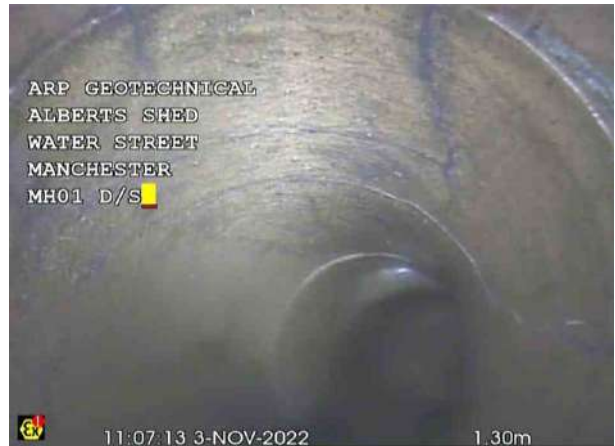
MH01X_ed977b99-f111-41eb-8f6f-aff2638454ed_20221103_111749_073.jpg, 00:00:07, 1.30 m Crack, circumferential from 10 o'clock to 3 o'clock
