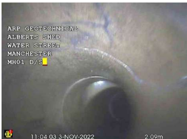
MH01X_758c0d89-b821-49e1-9045-a0146f49eaf0_20221103_111543_688.jpg, 00:00:08, 2.09 m Crack, circumferential from 10 o'clock to 3 o'clock
