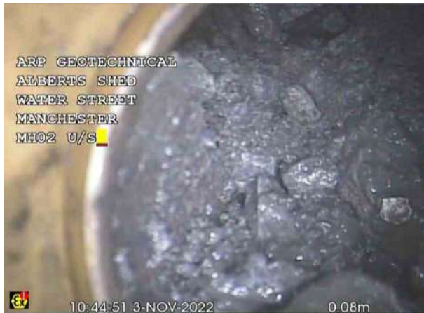
PIPE AX_f1247b96-911d-45ae-b513-4e620648cbef_20221103_115640_637.jpg, 00:00:01, 0.08 m Settled deposits, fine, 100% cross-sectional area loss
