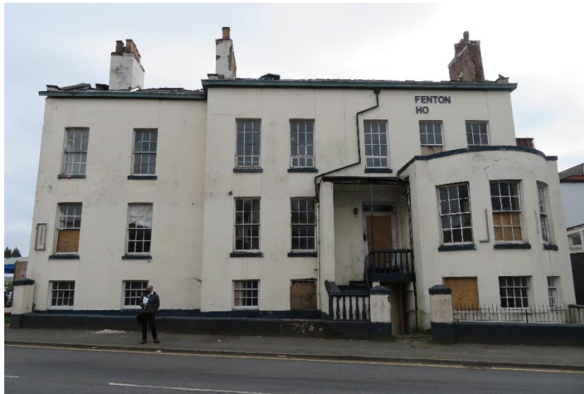
2021 Photograph of the west façade showing fire damage, generally deteriorating condition and historic alterations to the entrance doors and windows.
