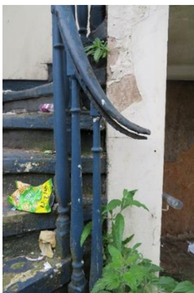
Damage to the bottom of the main cast iron banister at the main entrance steps.
