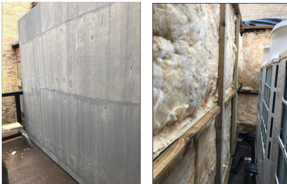
Figure 4 Photographs showing the installed screening (left- terrace side, right plant side)
