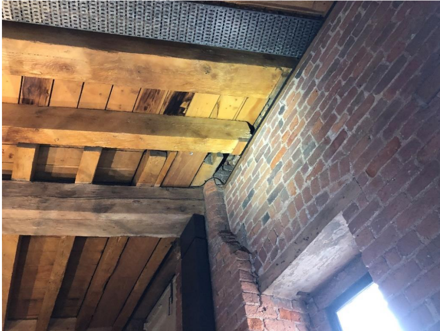
Photograph 07 – A full height photo of a ground floor pier at the inside of the Northern elevation, showing the extent of vertical cracking evident through bricks.
