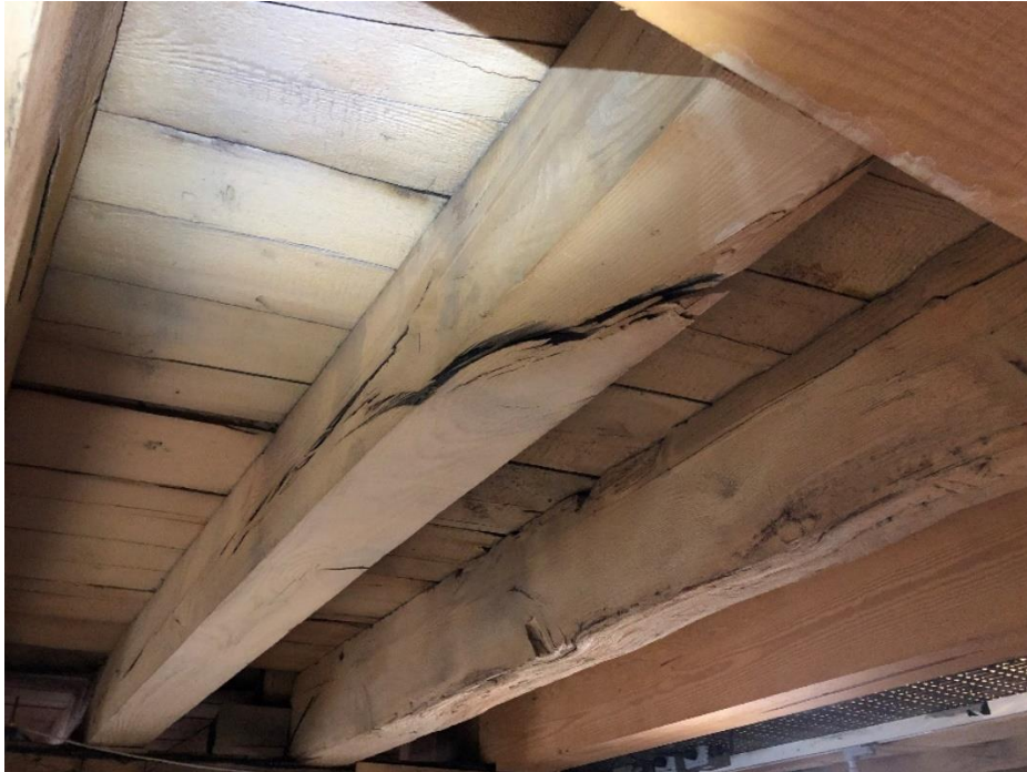
Photograph 13 – View from mezzanine floor level of cracking in floor joist.
