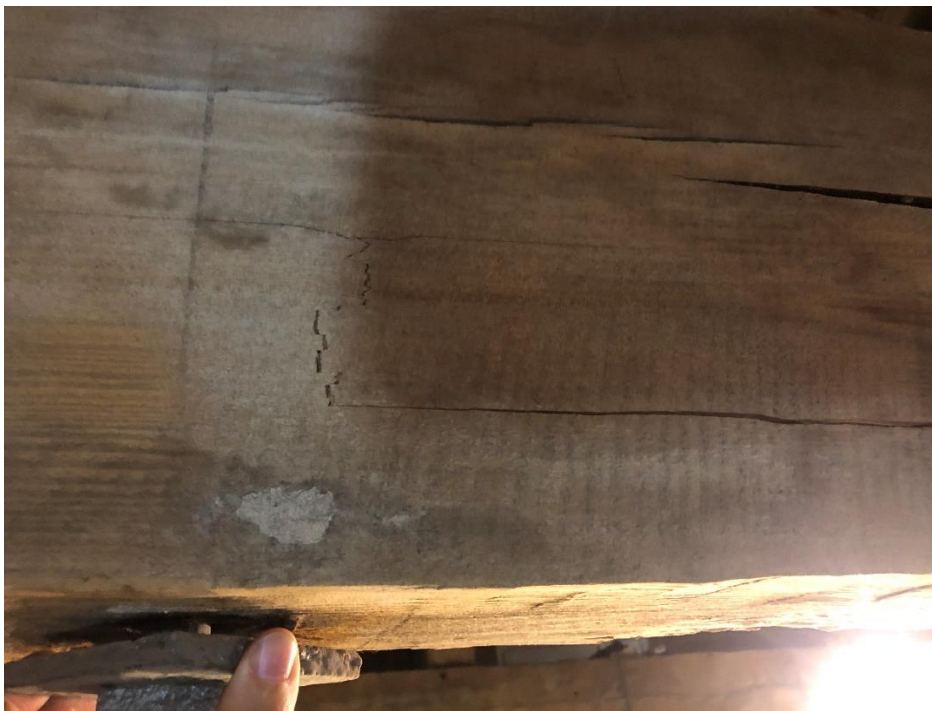
Photograph 24 – Close up of roof truss cracking, to the south of propped trusses in Bay 2, with cracking of main tie.
