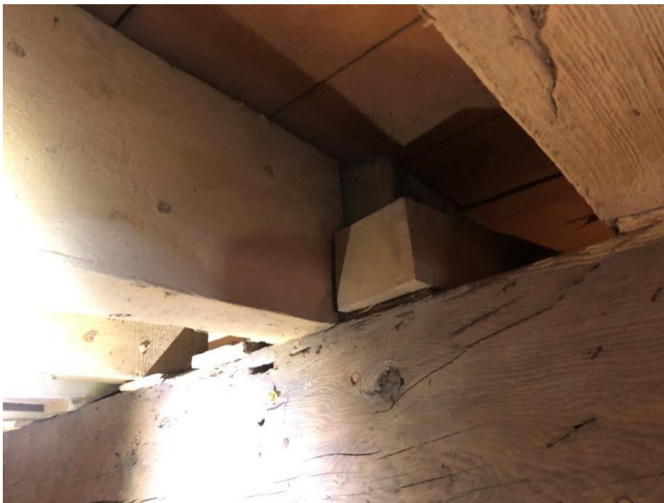
Photograph 03, 04: limited bearing of timber floor joist.
