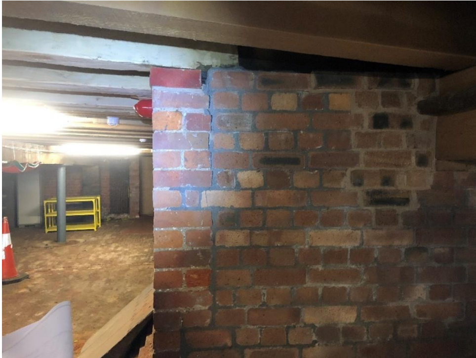
Photographs 05 - Stepped cracking, mortar loss and historic re-pointing at the face and return of the piers.
