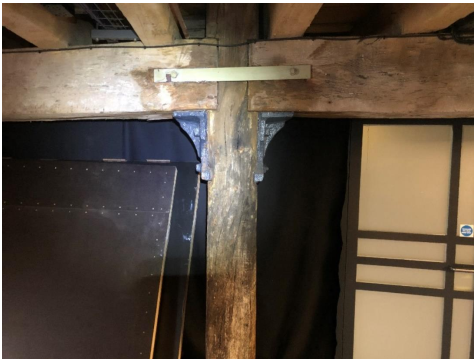
Photograph 10 – View from ground floor level of degraded timber post and beam, H&R to review level of rot.
