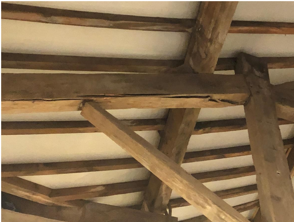
Photograph 25 & 26 – Roof truss in Bay 1 showing high level splitting in principal rafter.
