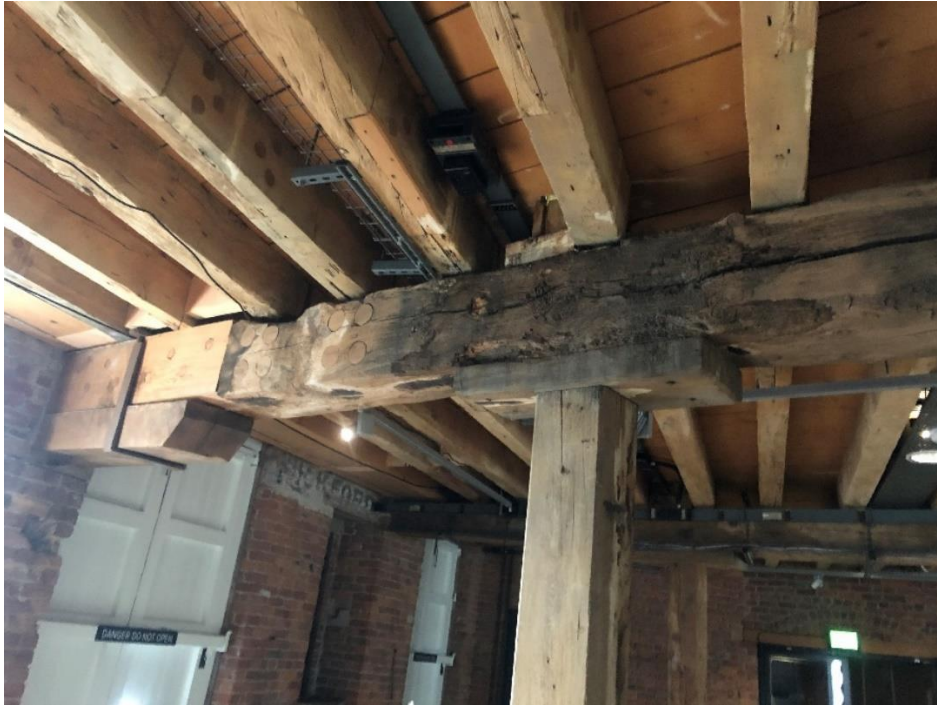
Photograph 15 – View from first floor level of degraded timber post and beam, H&R to review condition of timber.
