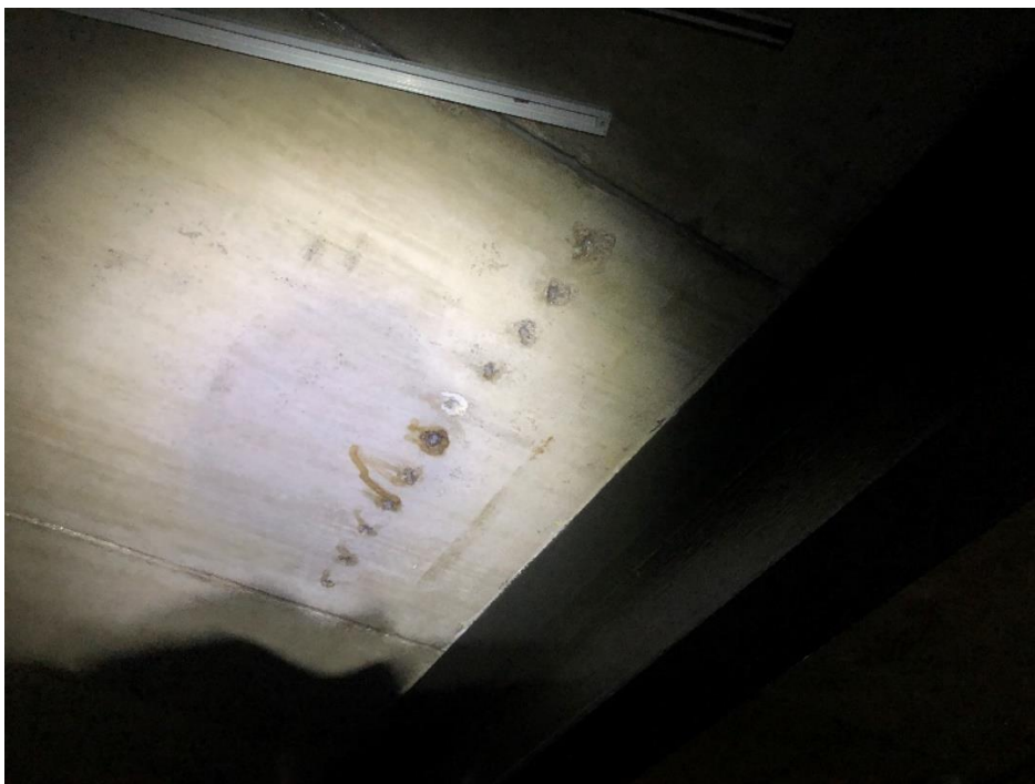
Photograph 14 – Service penetrations in precast concrete planks observed from first floor. locally filled using resin / mastic, however minimal corrosion assumed based on staining.
