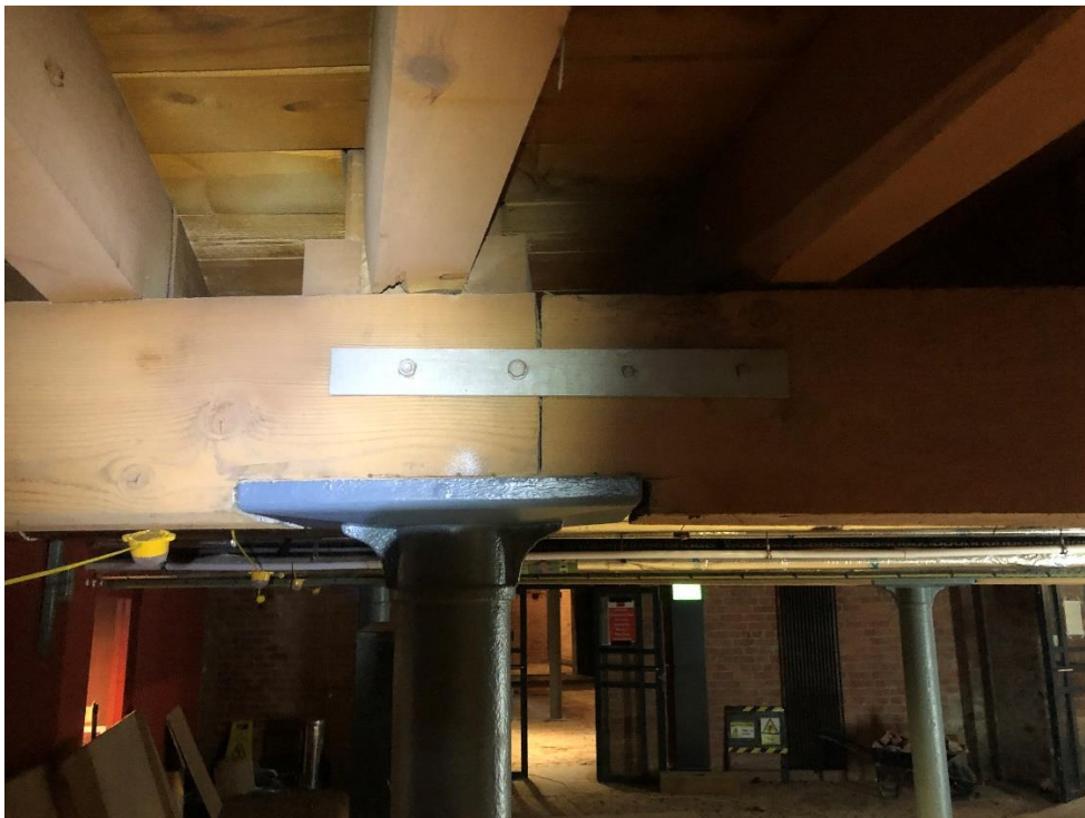
Photograph 06 - Floor beam 'but' connection off centre overcast iron column. s. floor beam eccentrically loading cast iron plate.
