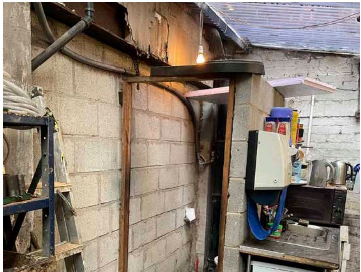
South west elevation as seen from inside garage, foul drainage and rainwater connected from rear. Corrugated plastic roof spanning off rear to create welfare facilities.
