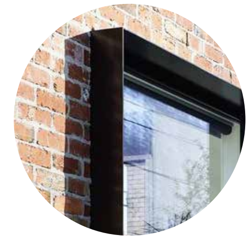
Protruding metal window reveals
