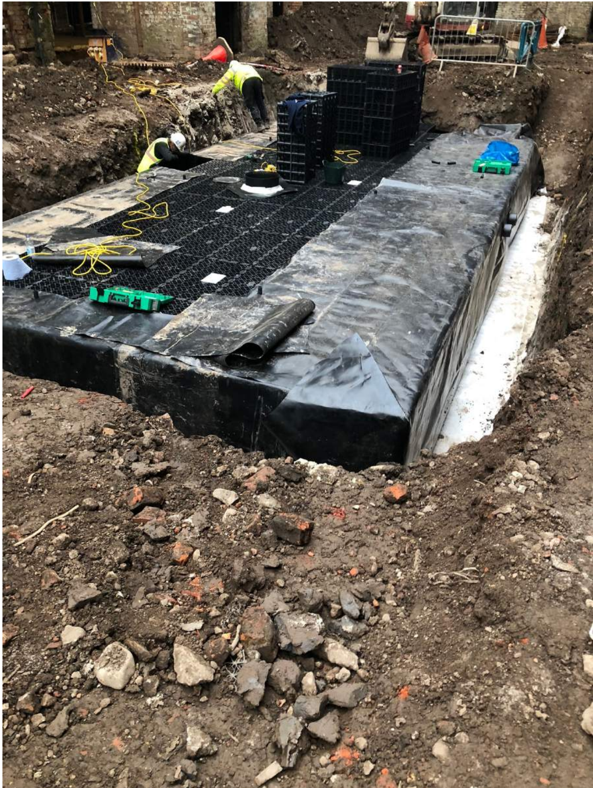
Surface water retention tank
