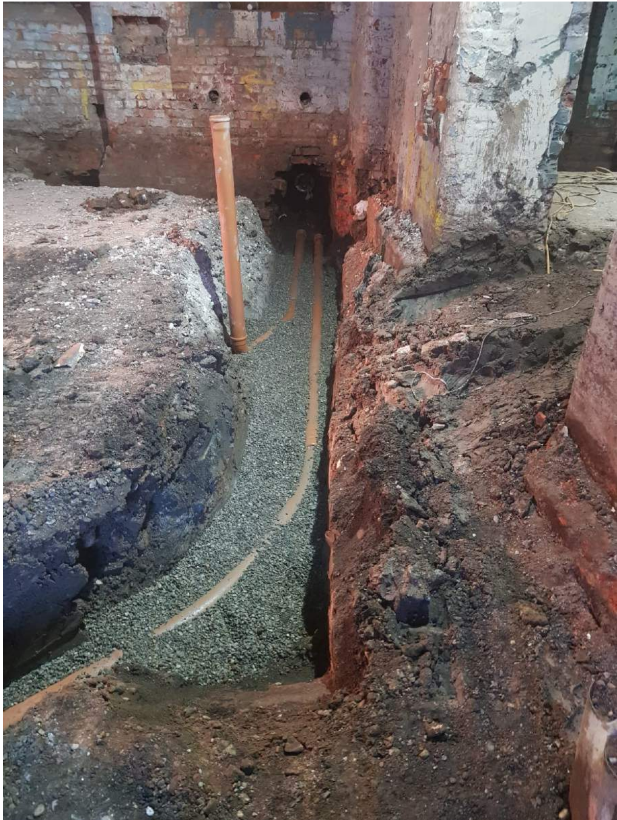
Building 2: Drainage passing below spine wall
