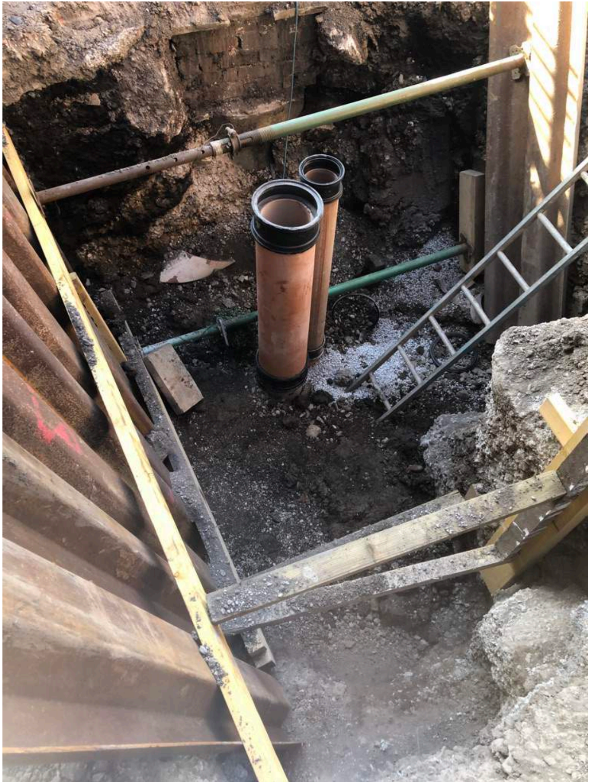
Main drain connection
