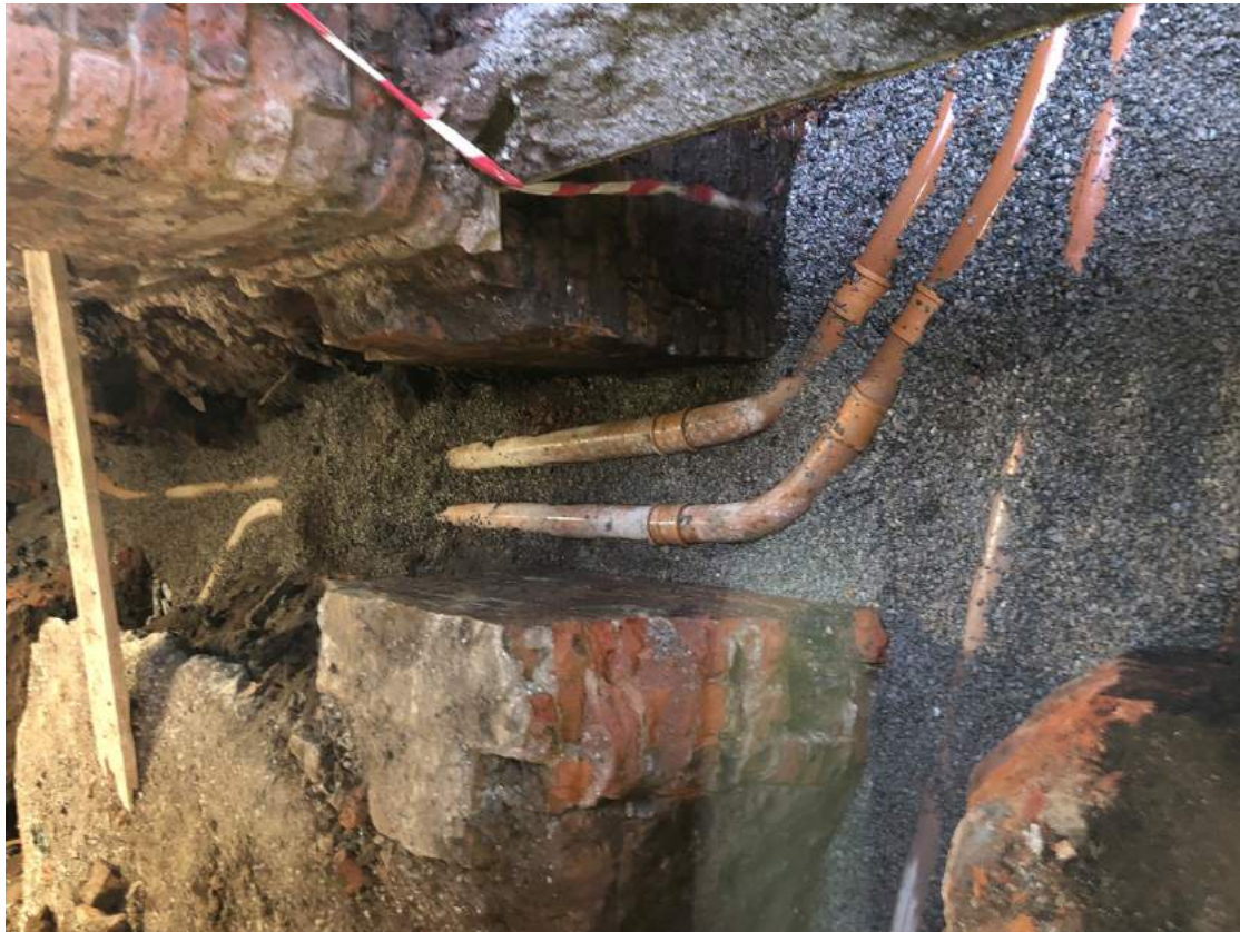
Building 2: Drainage passing from the building into the courtyard
