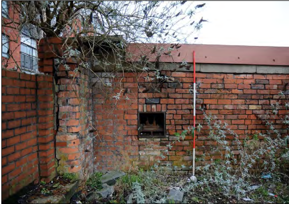
Plate 39. Location of line shaft bearing box, looking north
