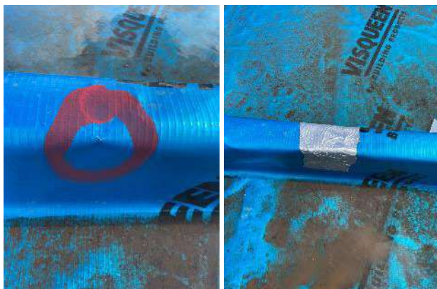
Figure 9 – Small hole noted and correctly patched using detailing strip.
