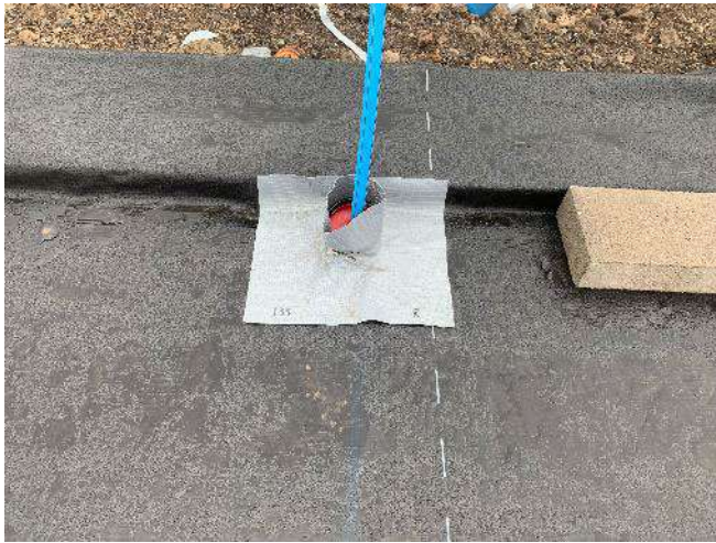
Figure 11 – Service penetration correctly sealed using a pre-formed top hat, double sided tape and jubilee clip.
