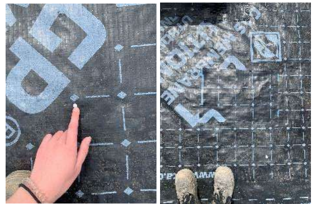
Figure 14 – Small hole noted and correctly patched using double sided tape.
