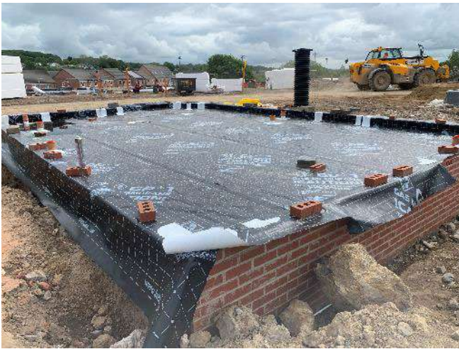
Figure 1 – Membrane neatly installed and in good condition.
