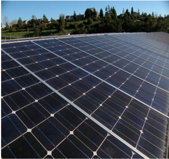
Figure 9: PV Panels/ Photovoltaic Array
